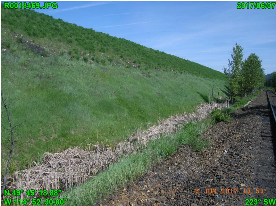
Photograph I - 9: Showing erosion at east slope toe of Lagoon C, looking north.
