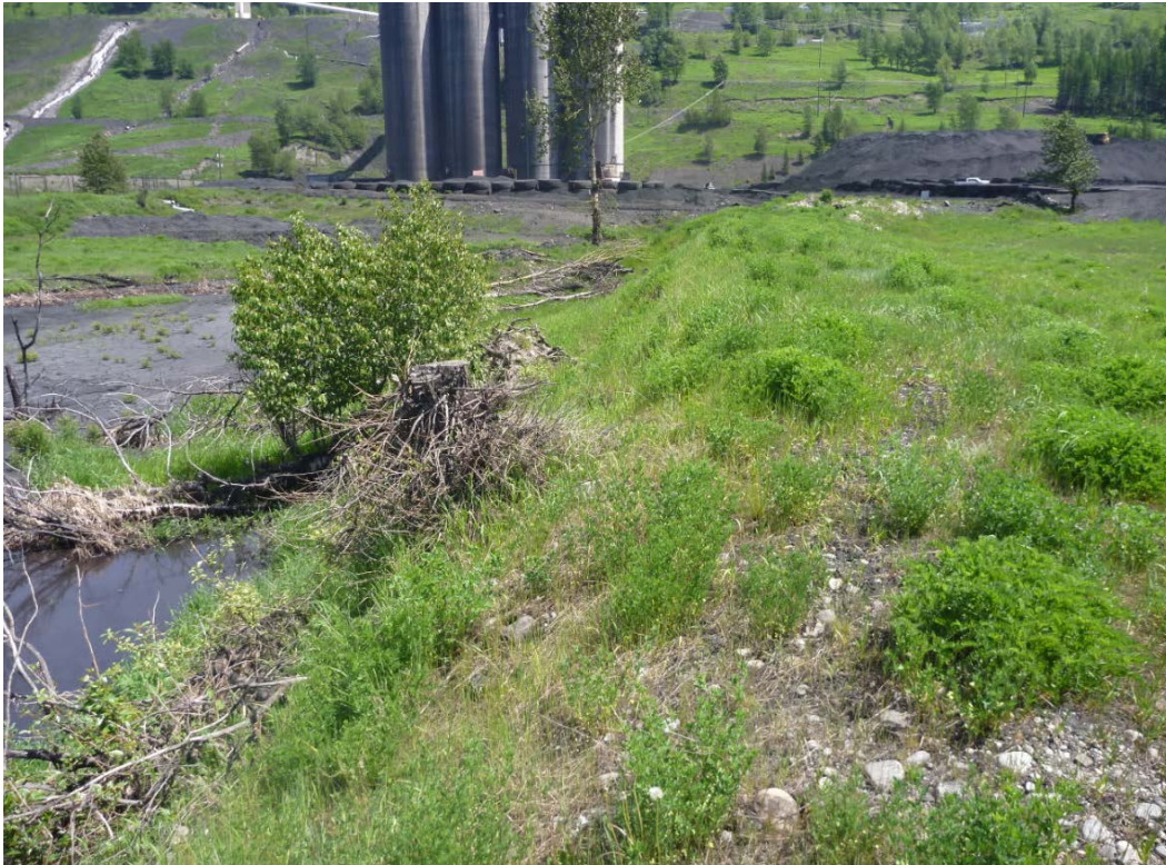
Photograph H - 3: Showing east end of the north embankment of Lagoon B, looking east. (Photo No. P1100789, 2017/06/07).
