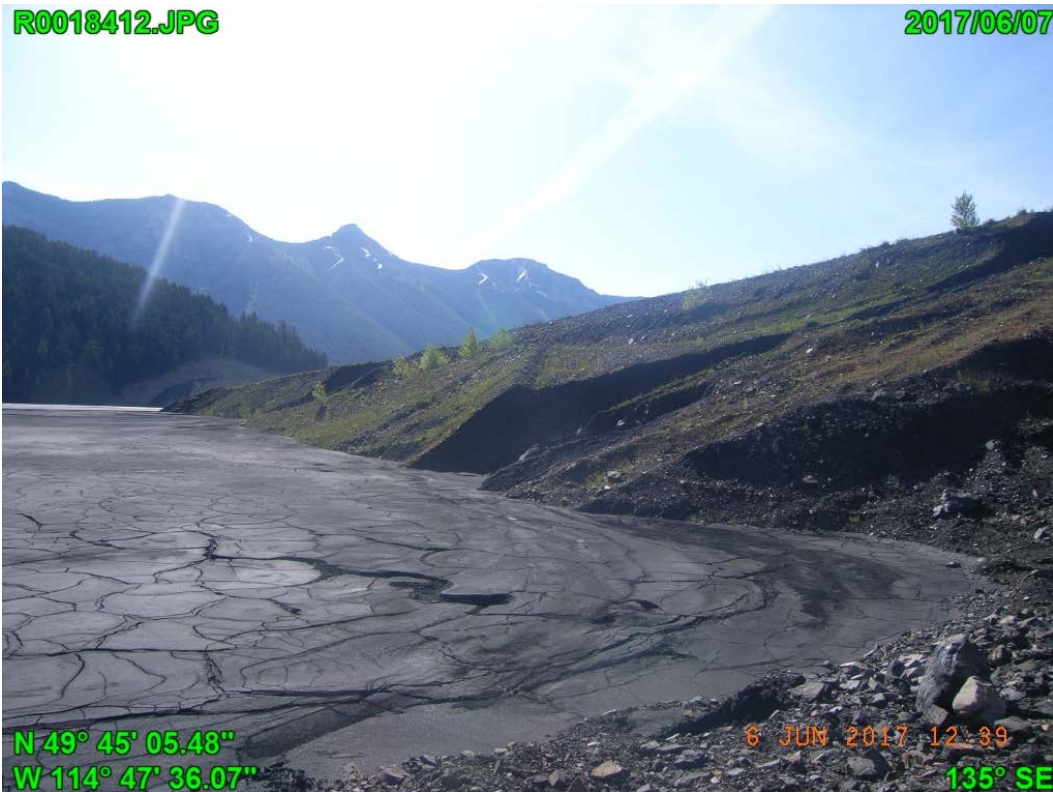
Photograph F - 8: Showing beach tailings on upstream, looking southeast from west abutment.
