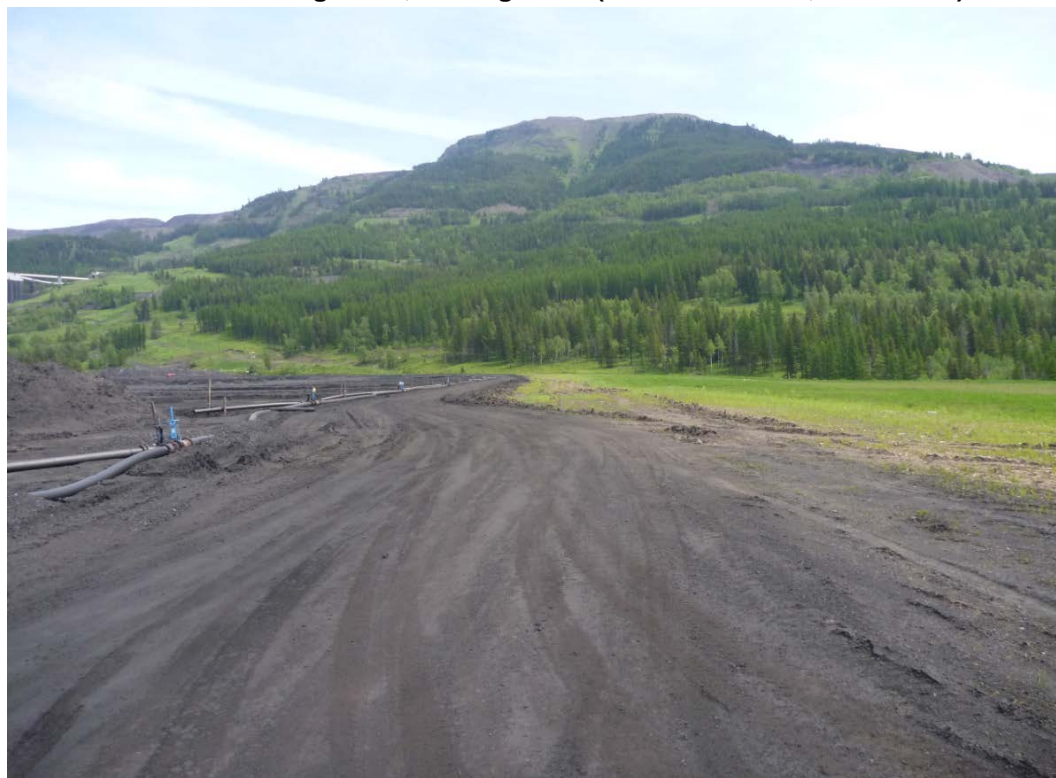
Photograph J - 32: Showing crest and upper south slope of Lagoon D, looking northeast. (Photo P1100736, 2017/06/06)
