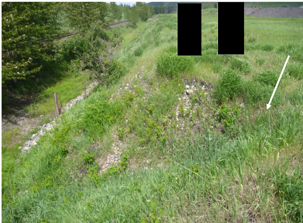
Photograph H - 8: Showing a pipeline at the toe at south end of the west embankment and an erosion gully, looking north. (Photo No. P1100775, 2017/06/07)
