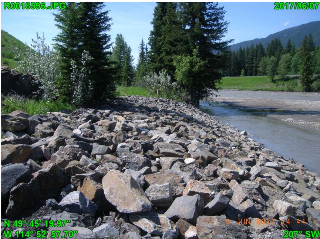
Photograph I - 23: Showing erosion riprap along the shoreline of the Elk River, at the west toe of Lagoon C, looking southwest.
