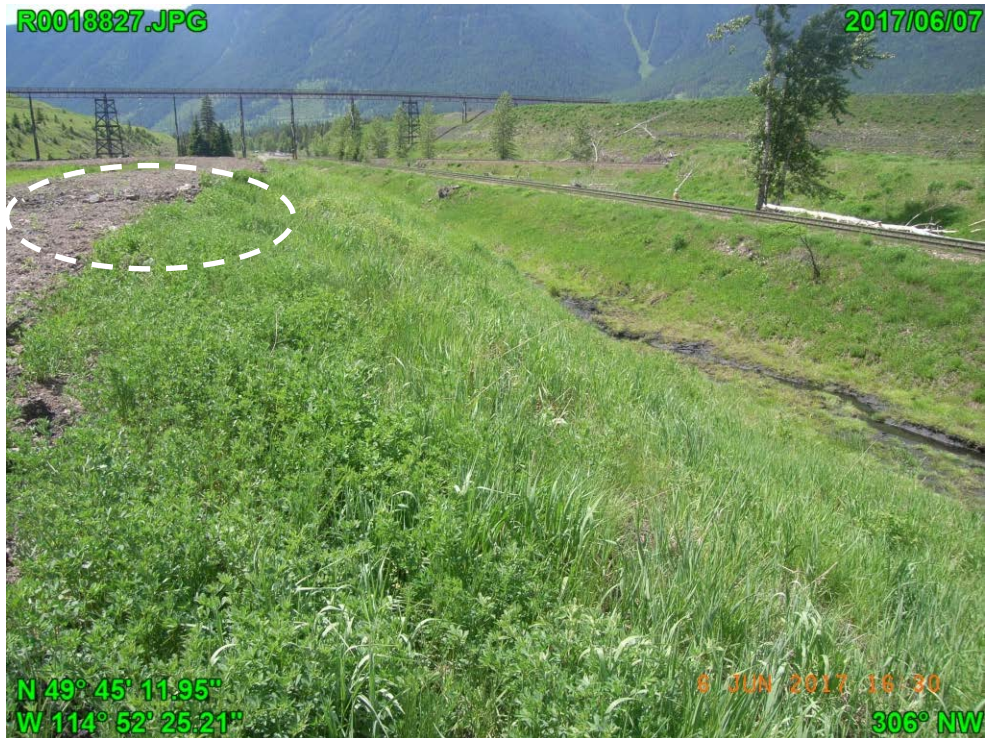
Photograph G - 16: Showing the downstream of north slope and another armored outlet further west, looking west.
