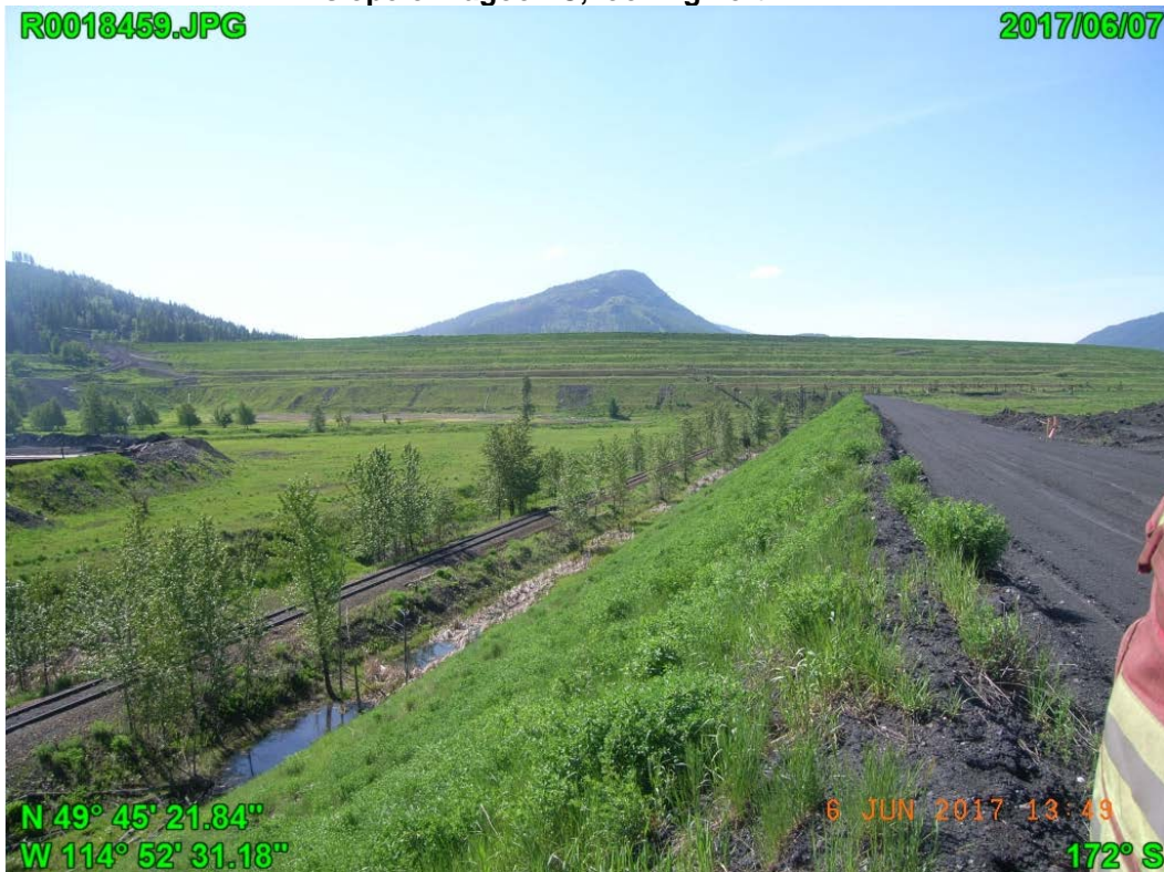
Photograph I - 6: Showing the crest and shoulder of the north end of east slope of Lagoon C, looking south.
