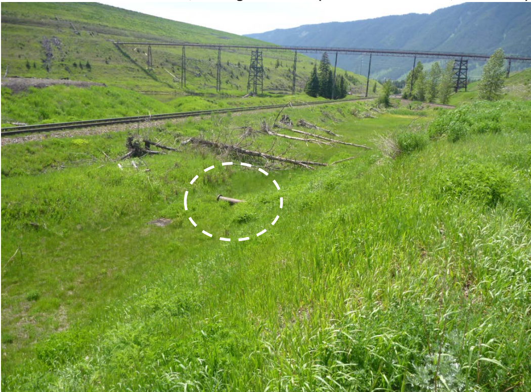
Photograph H - 12: Showing south end of Lagoon B, looking southwest. Noted the outlet steel pipe on the south slope. (Photo No. P1100764, 2017/06/07)
