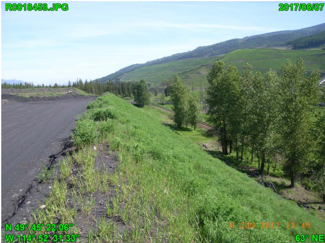
Photograph I - 5: Showing the crest and shoulder of the north end of east slope of Lagoon C, looking north.
