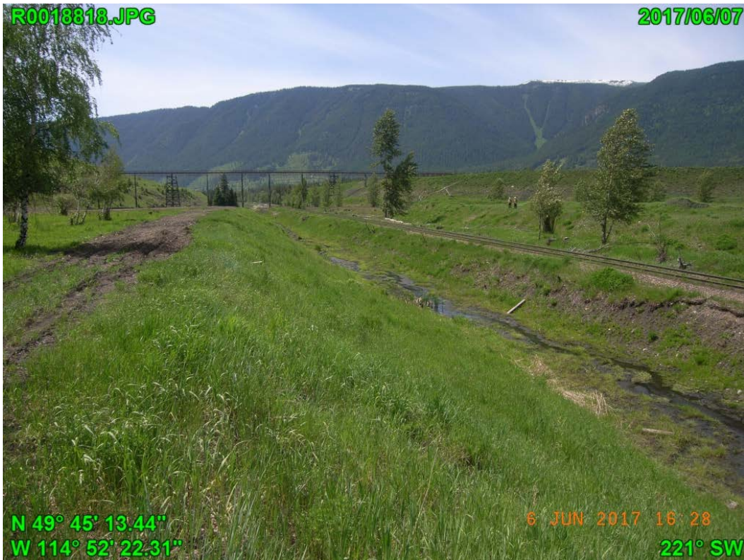
Photograph G - 13: Showing downstream slope of Lagoon A north embankment, looking southwest.
