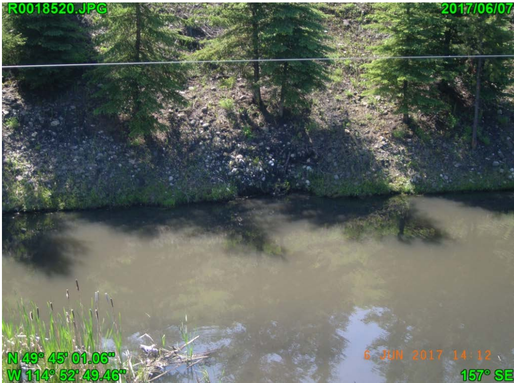
Photograph J - 17: Showing an erosion at the bank of the pond located at the toe of north slope of Lagoon D, looking south.
