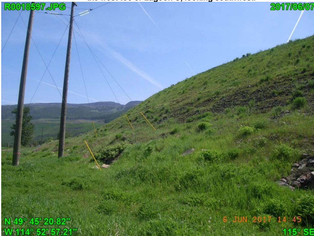
Photograph I - 24: Showing erosion on slope at northwest corner of Lagoon C, looking northeast.
