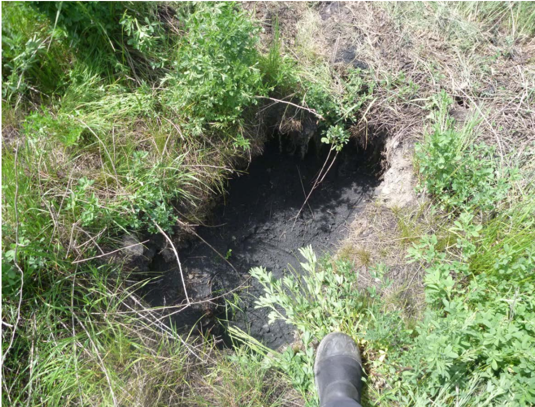
Photograph J - 27: Showing a sinkhole at south west crest of Lagoon D, looking east. (Photo P1100730, 2017/06/06).
