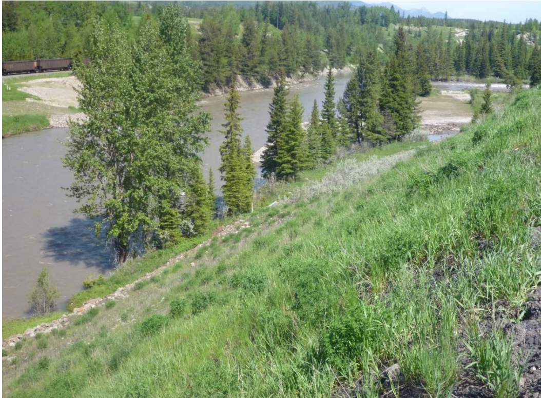
Photograph I - 19: Showing west slope and toe of Lagoon C, looking northwest. (Photo No. P1100657, 2017/06/07)
