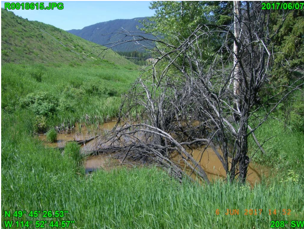
Photograph I - 27: Showing ponded water at toe of north slope of Lagoon C, looking west.
