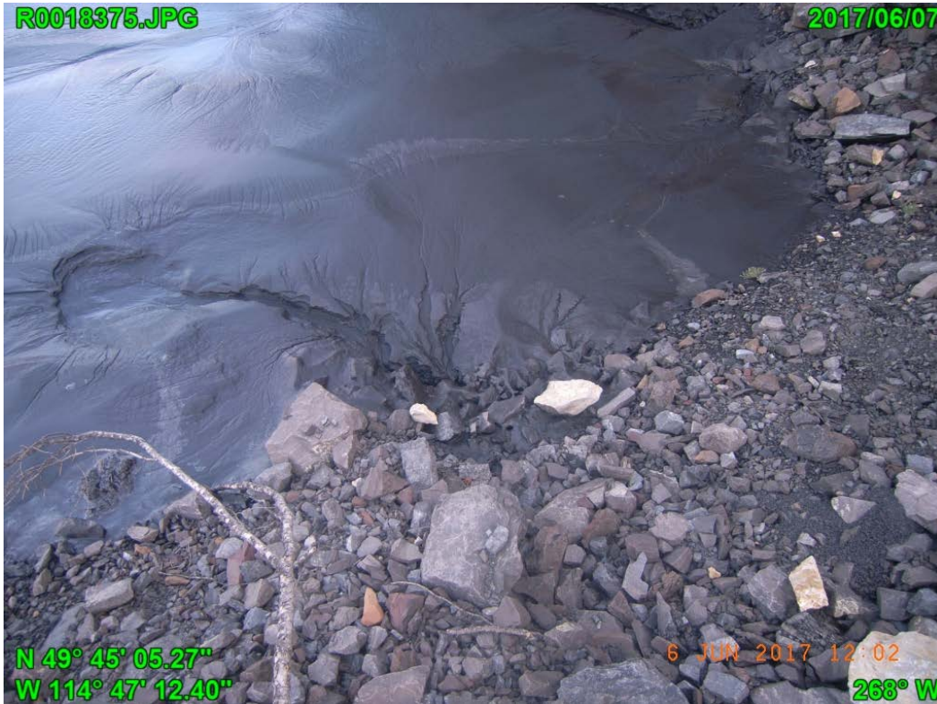
Photograph F - 15: Showing seepage at the east abutment against the 2013 raised, looking north.
