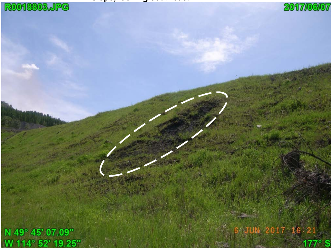
Photograph J - 12: Showing a close-view of the second seep area on the north slope, looking southeast.
