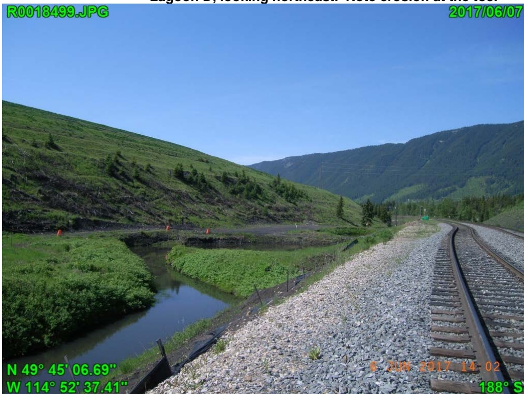
Photograph J - 16: Showing the lower north slope of Lagoon D, looking southwest. Noted Otto Pond at the toe and erosions on the slope.
