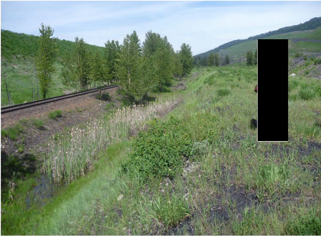
Photograph H - 5: Showing downstream slope of north end of the west embankment of Lagoon B, looking north. Noted ponded water at toe. (Photo No. P1100786, 2017/06/07)
