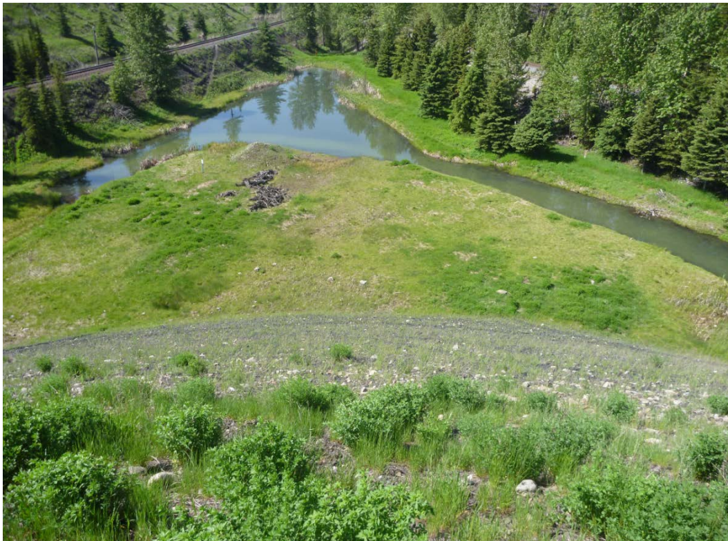
Photograph I - 14: Showing downstream toe at southwest corner of Lagoon C, looking southwest. (Photo No.P1100641, 2017/06/07)
