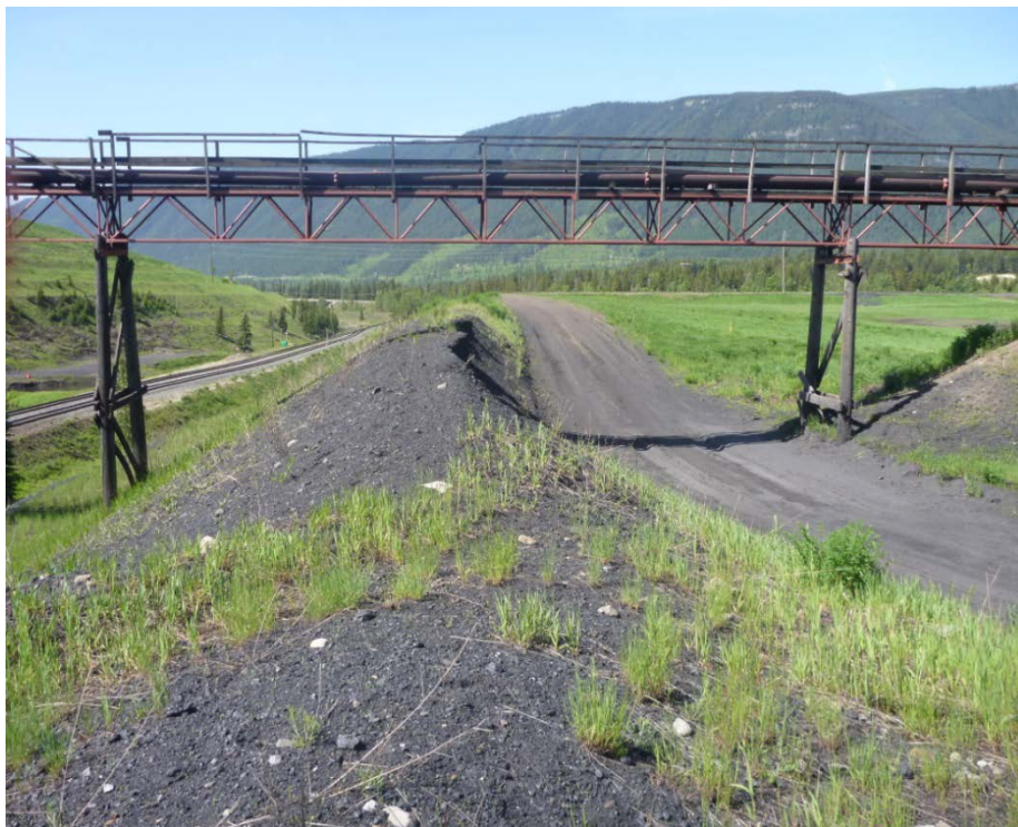
Photograph I - 12: Showing the crest and shoulder of Lagoon C south embankment, looking southwest. Noted the crest is narrow and the access road is depressed underneath the trestle. (Photo No.P1100623, 2017/06/07)
