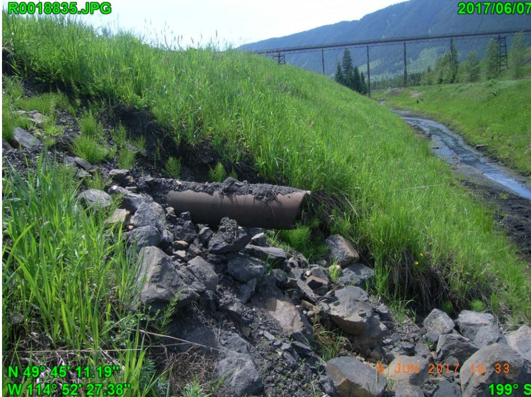
Photograph G - 19: Showing pipe flow on northwest end of Lagoon A, looking southwest.
