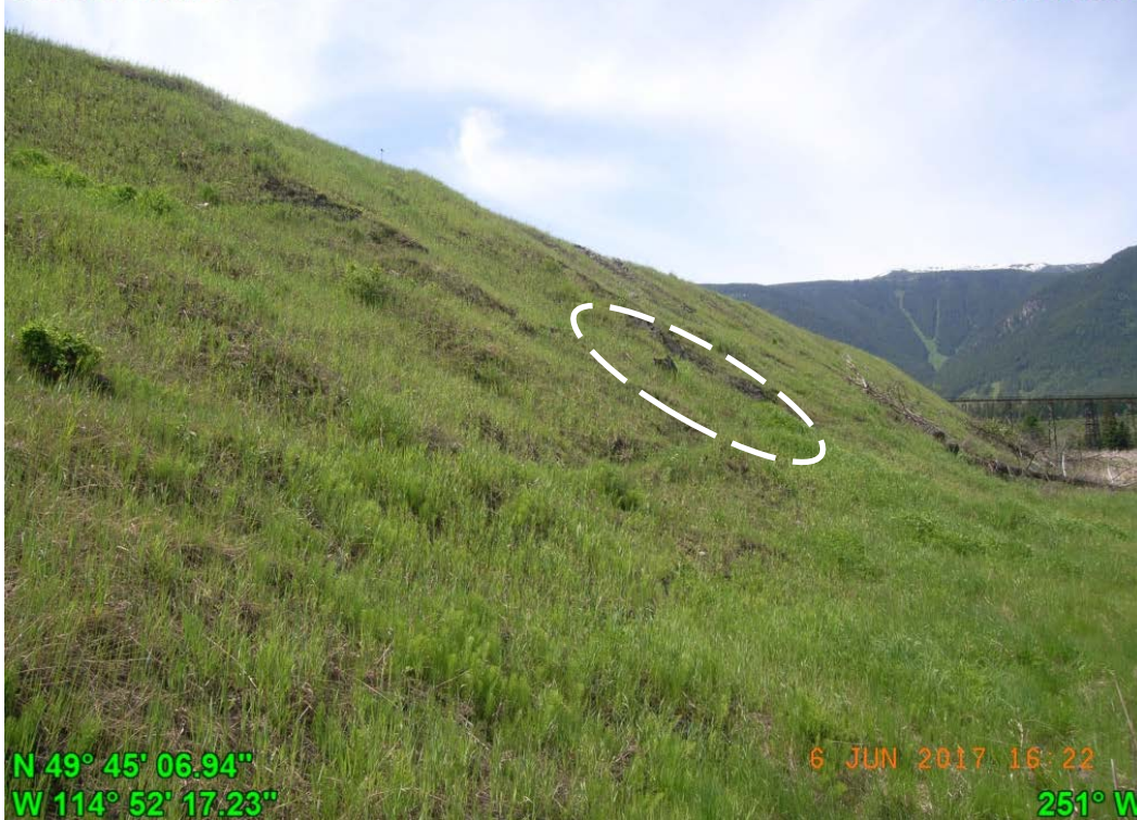
Photograph J - 10: Showing the toe and the 2 nd seep area at the east end of North toe of Lagoon D, looking west.
