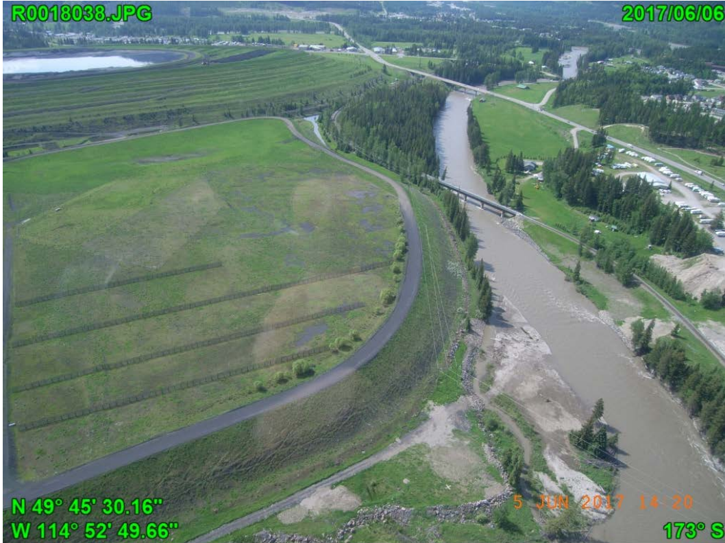
Photograph I - 17: Showing an aerial view of the west slope and toe of Lagoon C, looking south.
