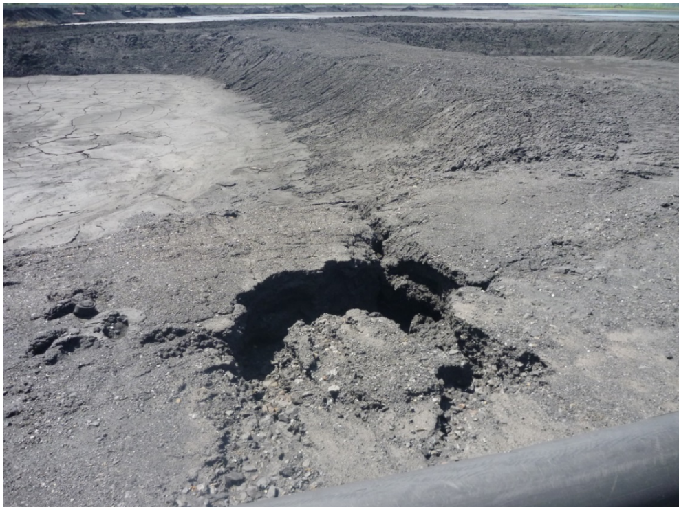
Photograph J - 8: Showing a close-view of a sinkhole within the tailings cell of Lagoon D, looking south. (Photo P1100688, 2017/06/06)
