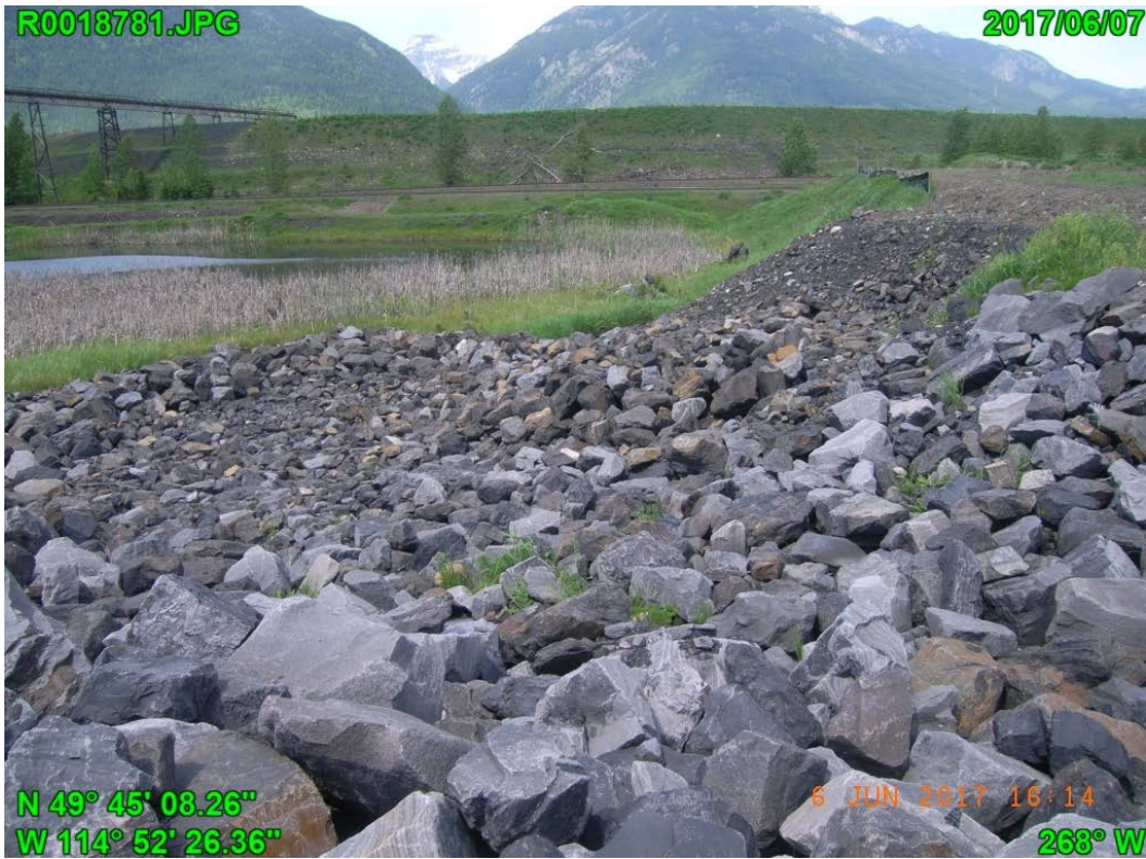
Photograph G - 7: Showing the spillway and riprap placement at downstream west slope, looking northwest.
