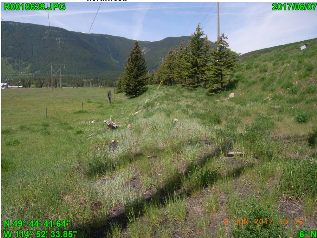
Photograph J - 30: Showing the toe of the south embankment of Lagoon D, looking west.
