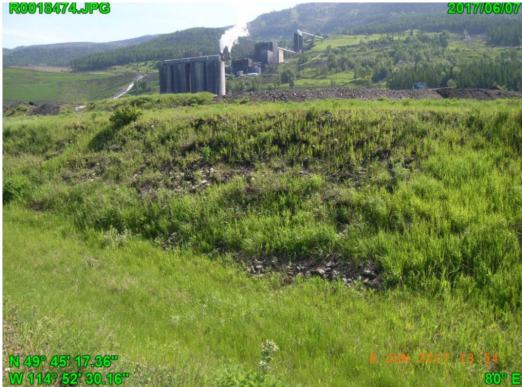
Photograph H - 7: Showing erosion on the slope of west embankment of Lagoon B, looking northeast.
