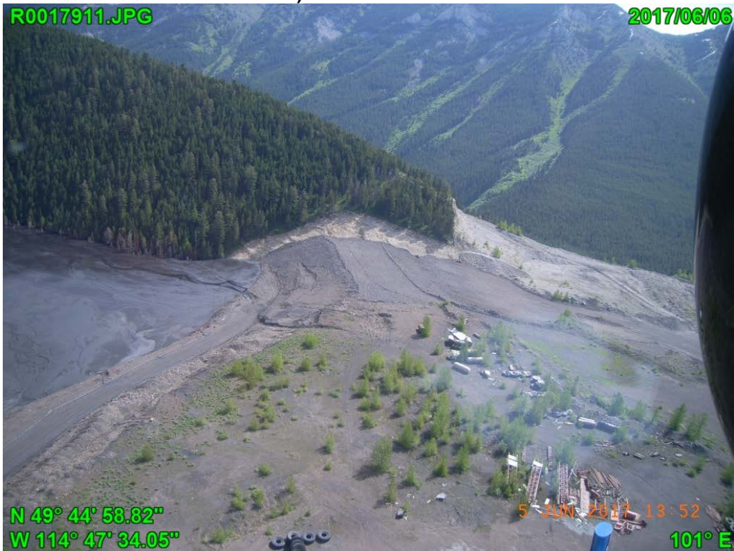
Photograph F - 14: Showing the 2013 raised area at the east abutment, looking east.
