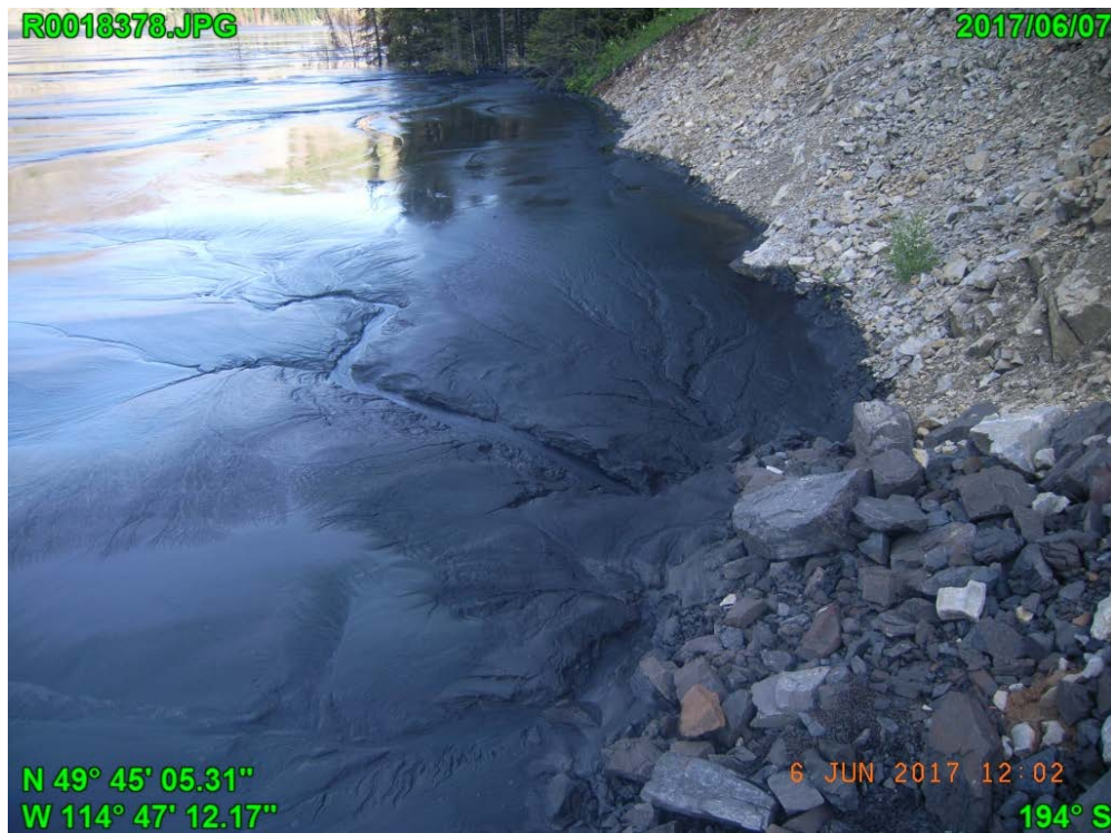
Photograph F - 16: Showing tailings beach at southeast corner of the basin, looking north. Noted seepage track on the tailings beach.
