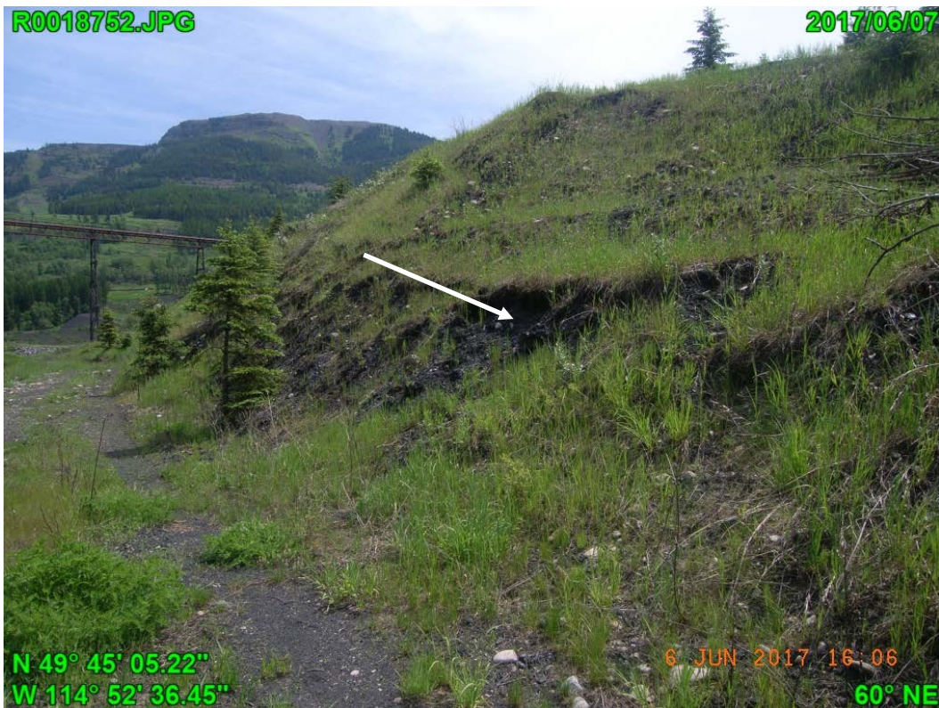
Photograph J - 15: Showing the toe and lower section of north slope of Lagoon D, looking northeast. Note erosion at the toe.
