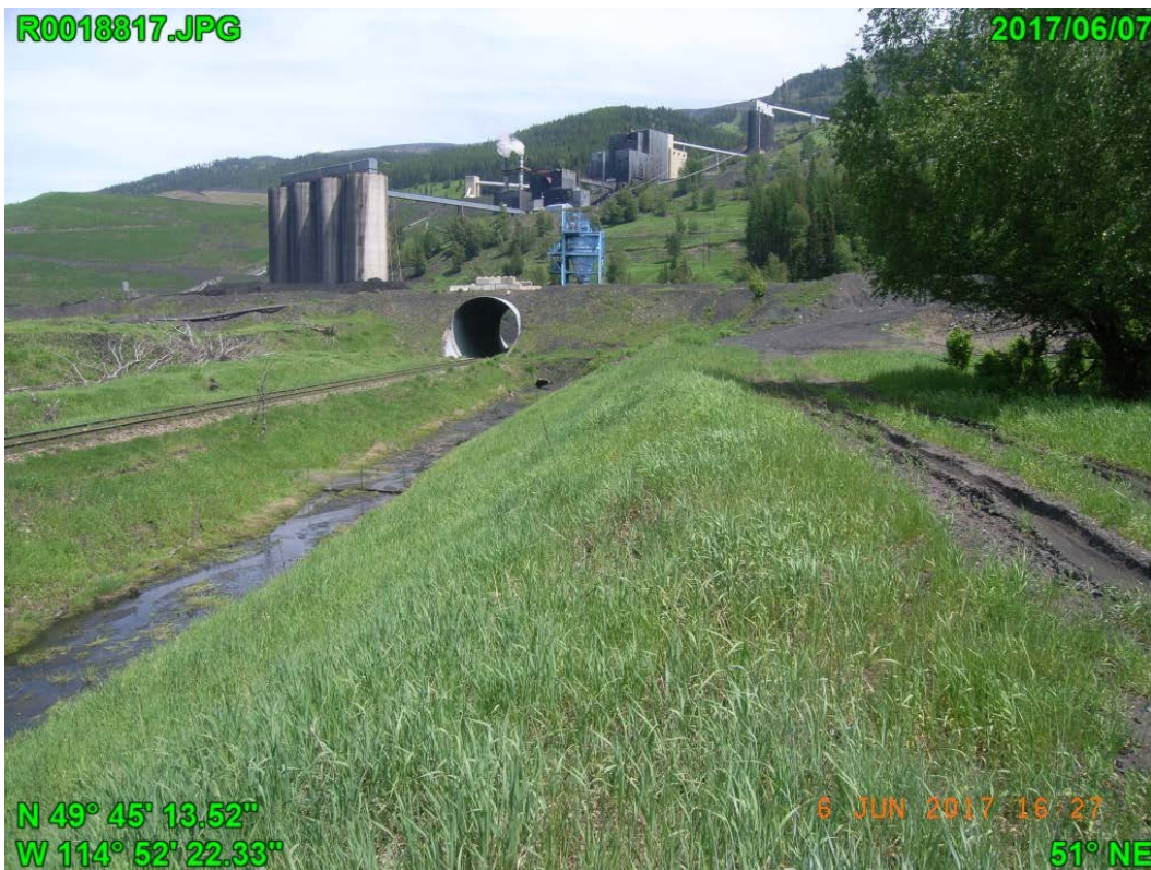
Photograph G - 12: Showing downstream slope of Lagoon A on north embankment at northeast corner, looking northeast.
