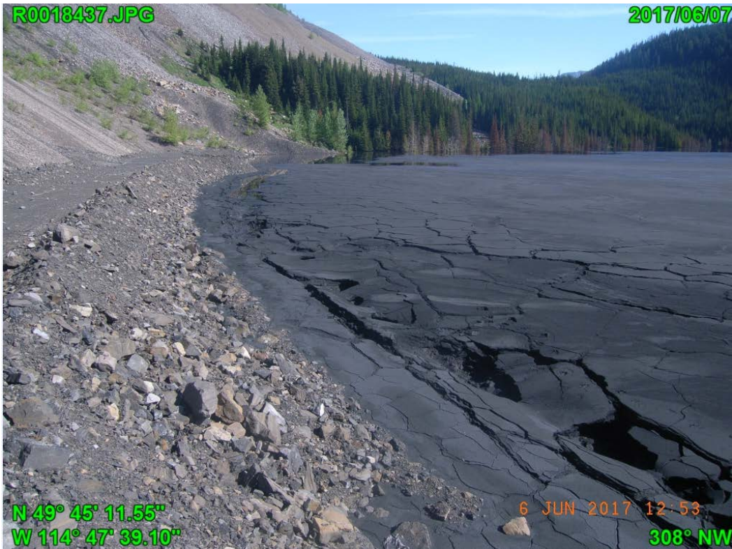
Photograph F - 7: Showing road constructed along toe of Adit dump looking northwest.
