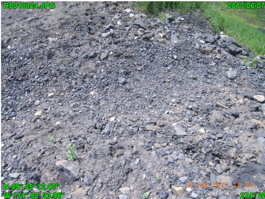
Photograph G - 15: Showing the closer view of the armored outlet on the north slope, looking west.
