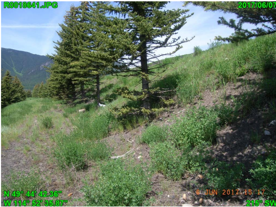
Photograph J - 29: Showing erosion on the south slope of Lagoon D, looking northwest.
