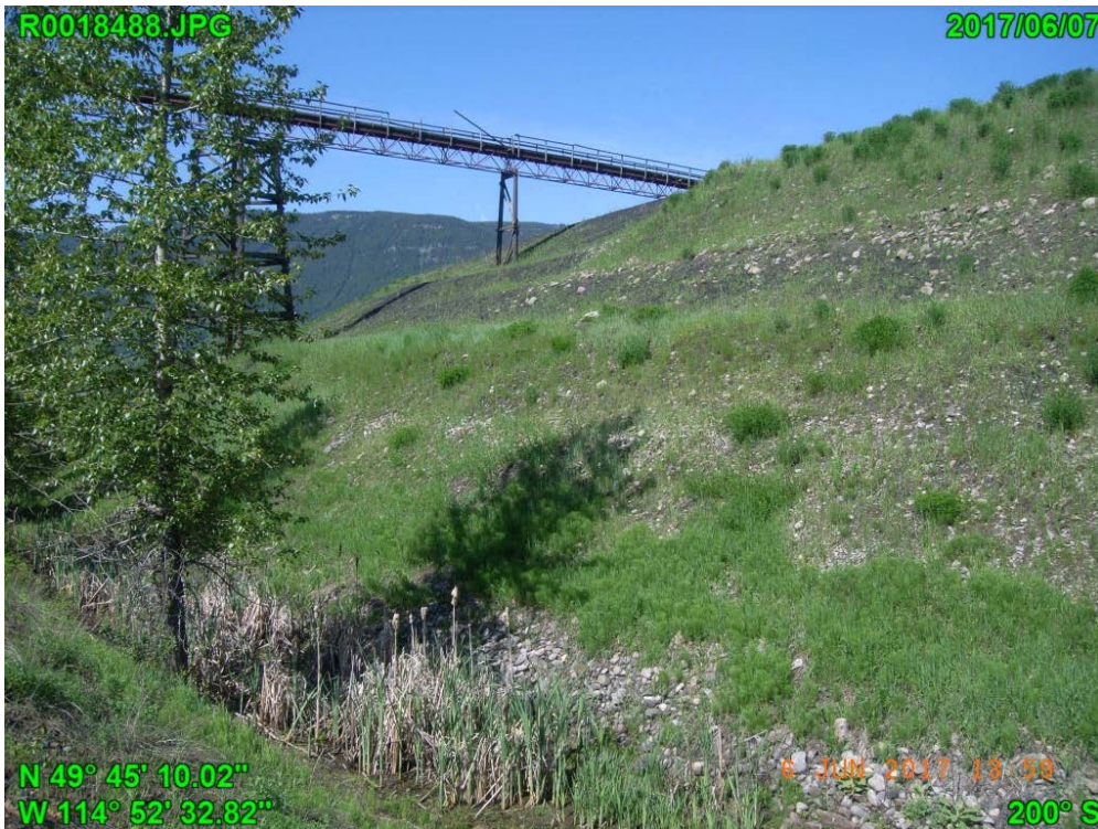
Photograph I - 11: Showing toe and downstream slope at the southeast corner of Lagoon C, looking southwest.
