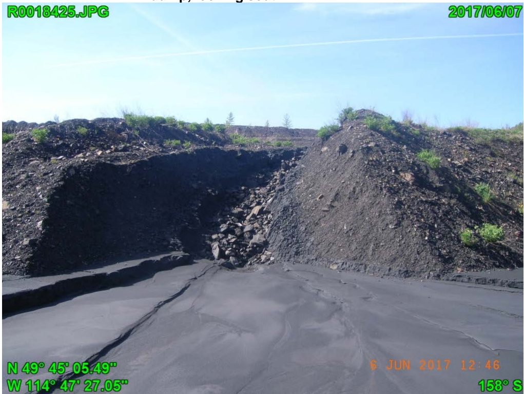
Photograph F - 12: Showing an erosion gully on upstream slope due to tailings discharged from spigot 2 pipe, looking south.
