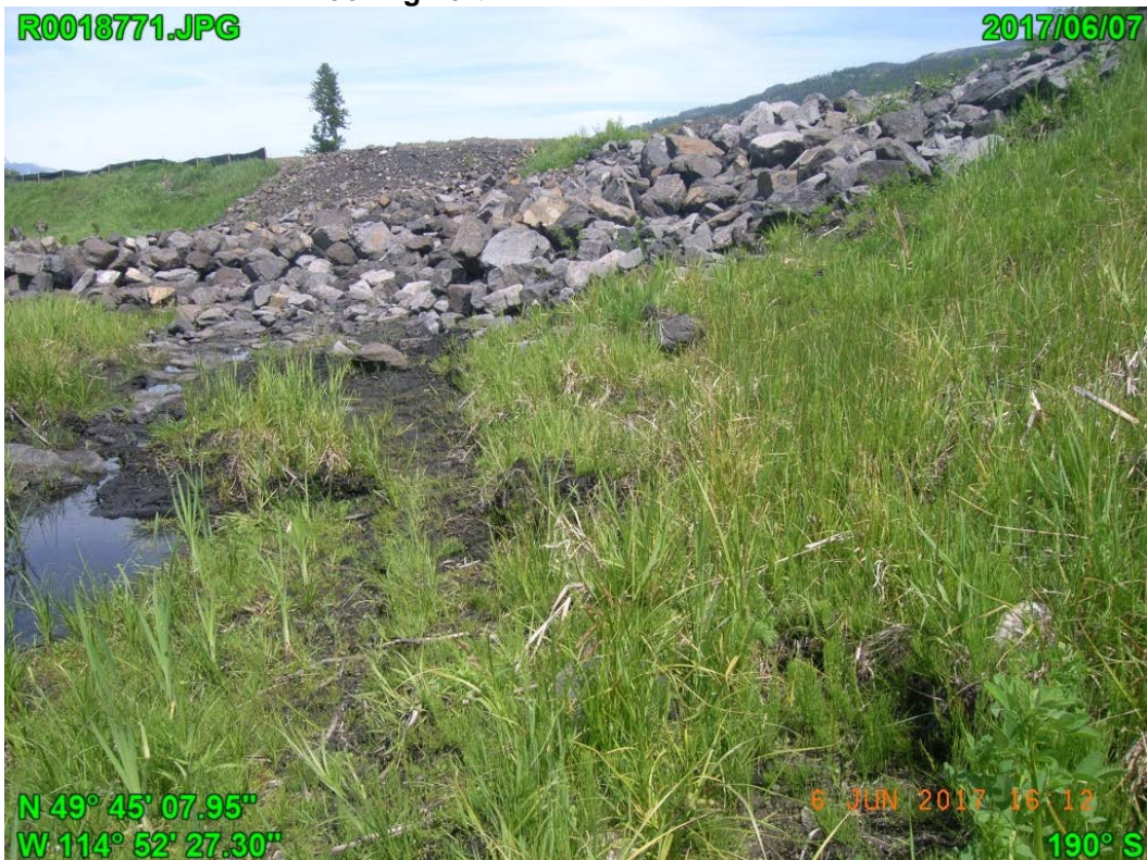
Photograph G - 6: Showing downstream of the spillway of the west face of Lagoon A, looking north.
