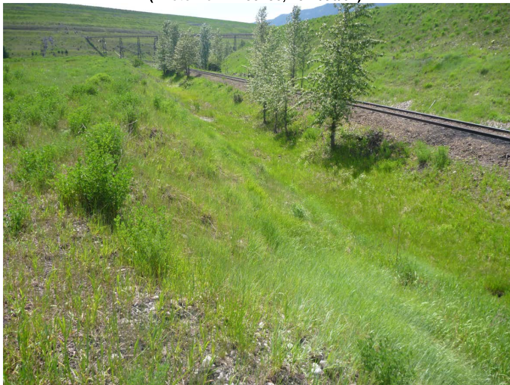
Photograph H - 6: Showing west embankment of Lagoon B, looking southwest. (Photo No. P1100784, 2017/06/07)
