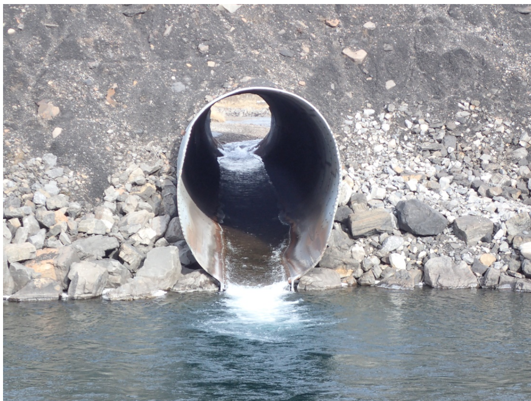
Figure 3.3.25. Multi-plate culvert on the mainstem upper Fording River illustrating fish passage characteristics.
