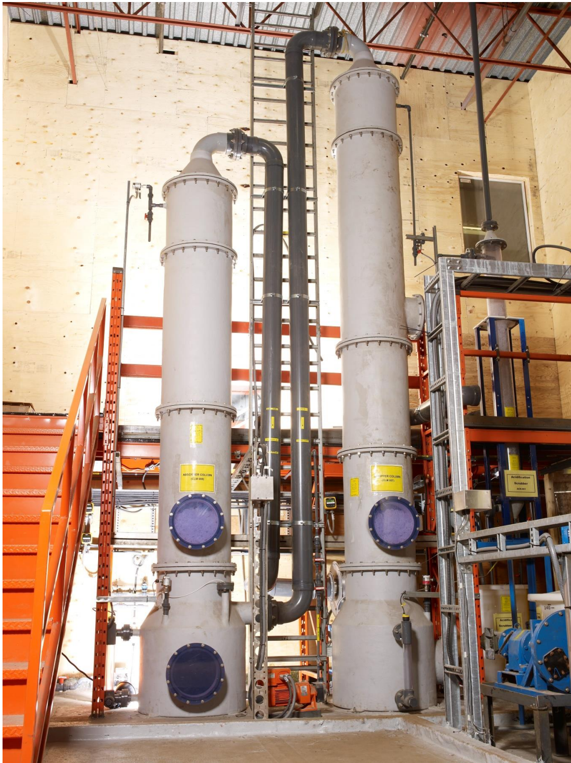
Figure 3 - Demonstration Plant AVR Circuit Absorber (right) and Stripper (left) Columns
