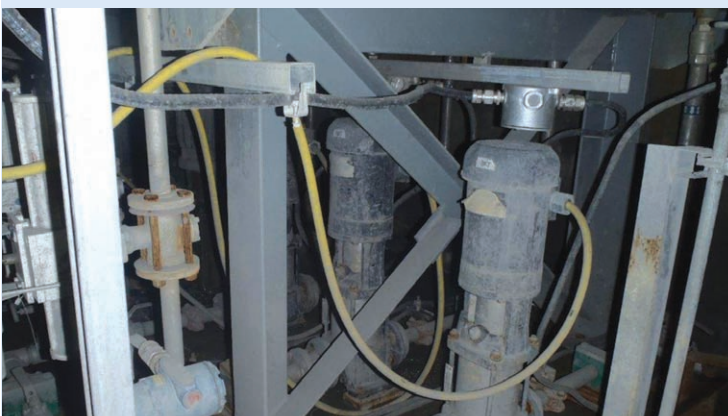
Completed cable to pump motor.
