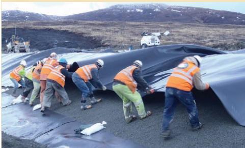
Paa River & Layfield laying liner on the West Abutment of Main Dam
