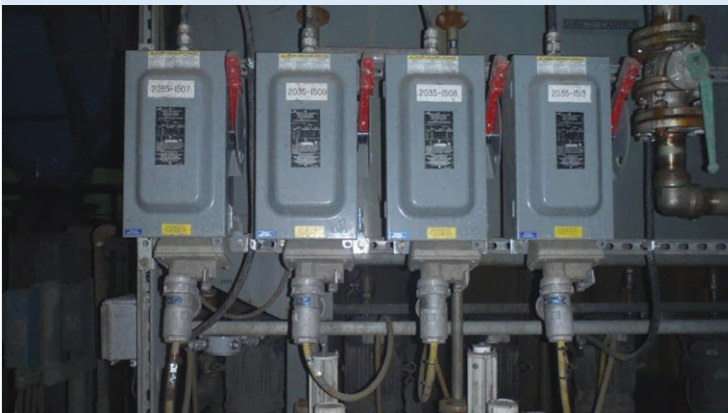
Disconnects with plug feed to pump motor.
