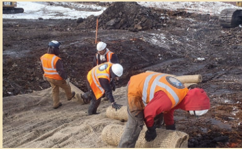
Paa River crew rolling out jute for erosion control on Sulfur Creek Diversion.
