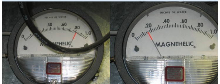
Magnetic gauge showing before and after coil cleaning data.
