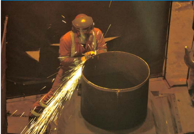
Tim Hilton, Millwright and Relief Supervisor field fitting HAPS flanges for installation.
