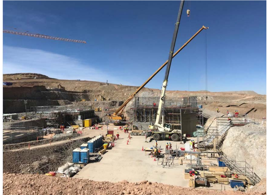
Concentrator - Grinding Area. June 2019.
