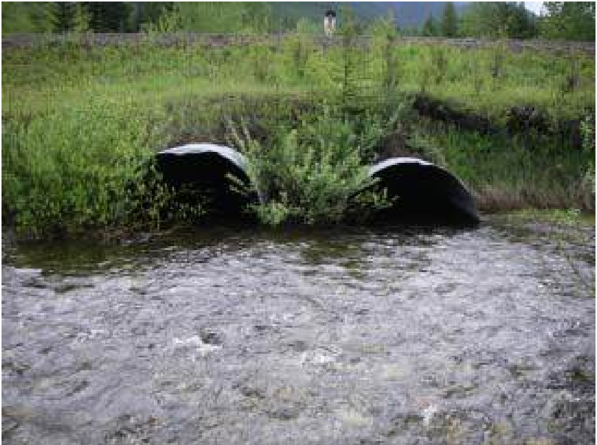
Photo 3.6: Paired culvert crossing under Fording Road in Dry Creek (Teck 2011b).
