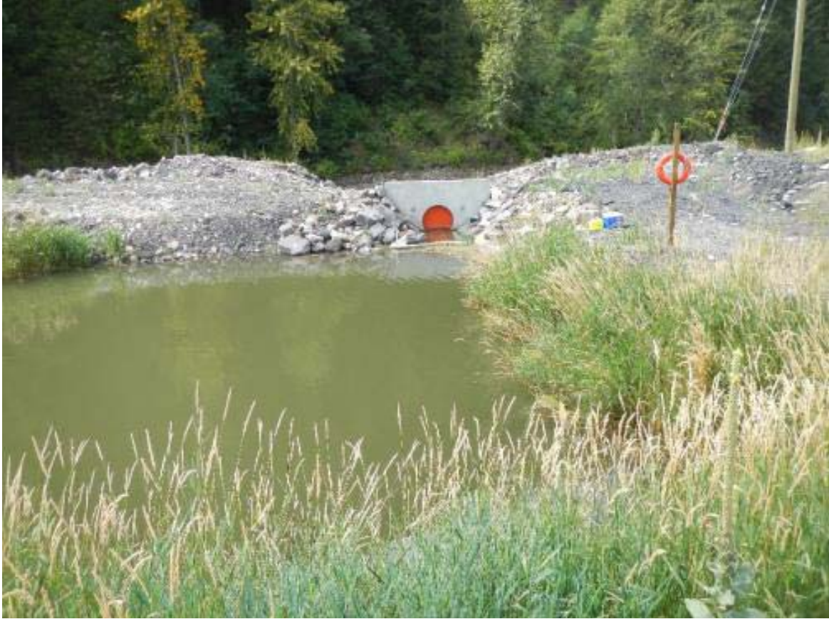
Photo 6.10: Downstream view of the concrete culvert and flap valve for Gate Creek (Lotic 2015a).
