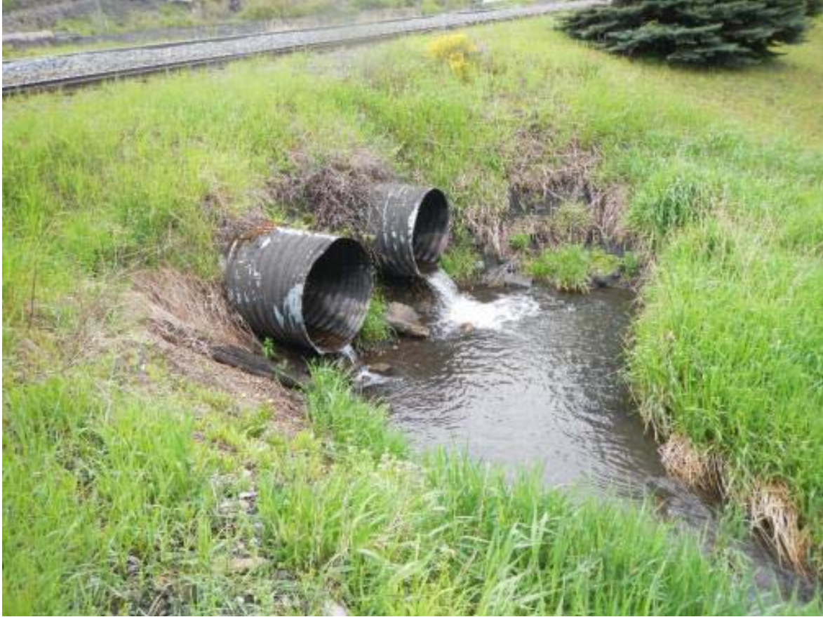
Photo 6.11: CPR double culverts in Bodie Creek (Lotic 2015a).
