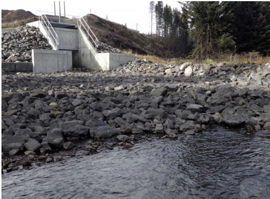
Figure 12. Looking upstream from the UFR (foreground) at Lake Mountain Creek and the fish exclusion structure on October 9, 2018.
