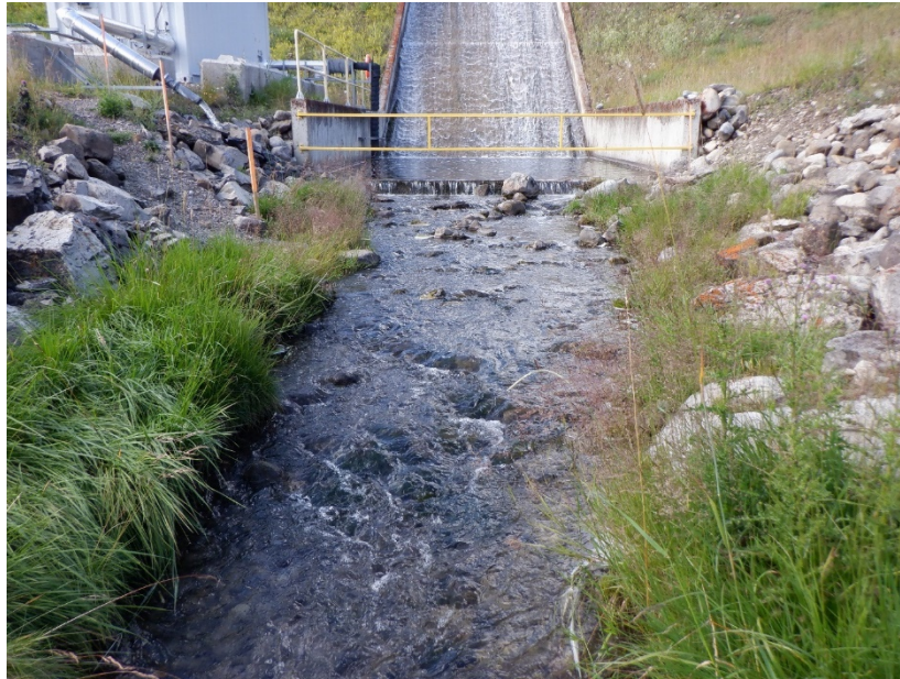
Figure 43. Looking upstream at the fish exclusion structure on Lower Greenhills Creek on August 13, 2019.
