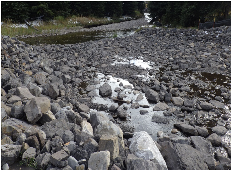
Figure 14. Looking downstream from the fish exclusion structure in Lake Mountain Creek through the rip rap channel towards the UFR on October 9, 2018.
