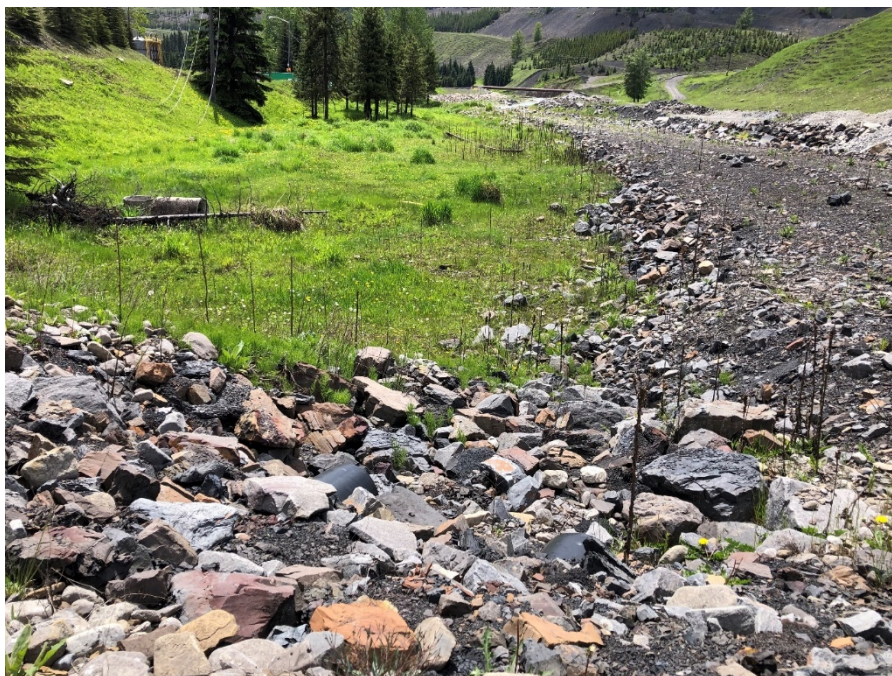
Figure 19. Discharge culverts in MS Settling Ponds Channel on June 22, 2020.
