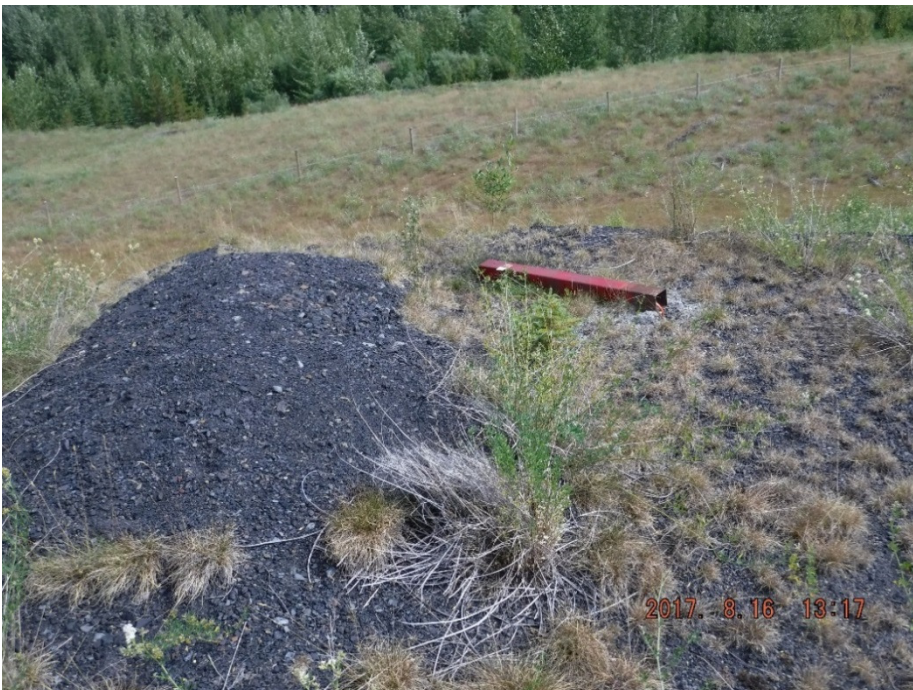
Photo II-17 Piezometer PN-3 – area was identified as unstable in 2015 DSR report; appears to be a pad constructed to facilitate drilling
