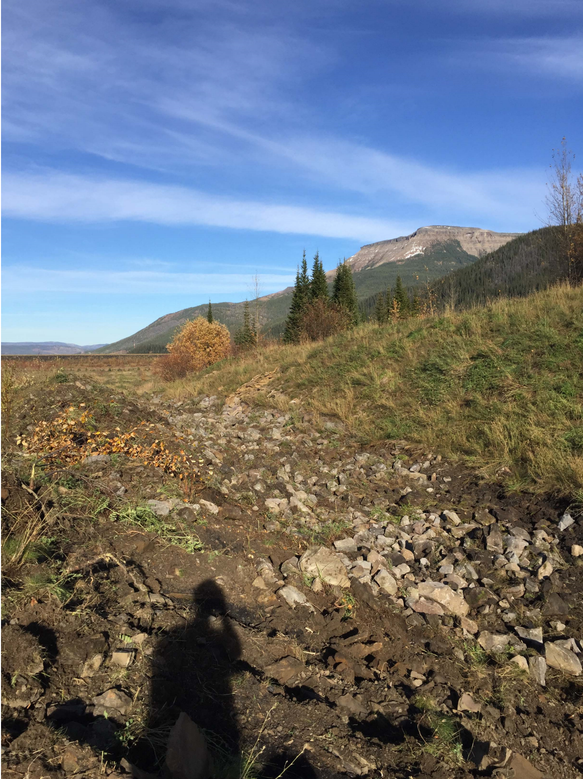
Photo II-32 Teck removed vegetation at the inlet and along the channel of spillway in October 2017 – looking northeast (near photograph location BTD-2017-21)
