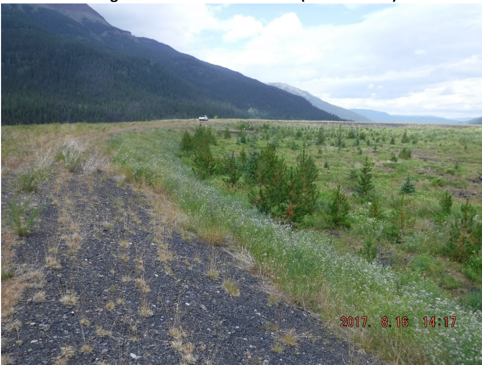
Photo II-23 Upstream slope – looking northeast. Slope is in good condition with no significant sign of erosion or movement (BTD-2017-19)
