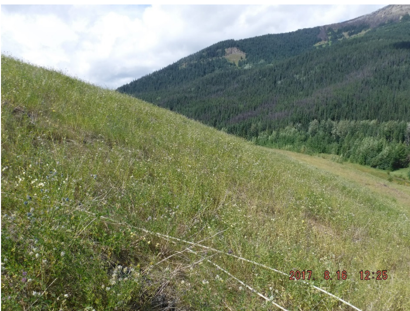
Photo II-9 Overview of the upper portion of the downstream slope – looking northwest. No sign of erosion or distress (BTD-2017-06)
