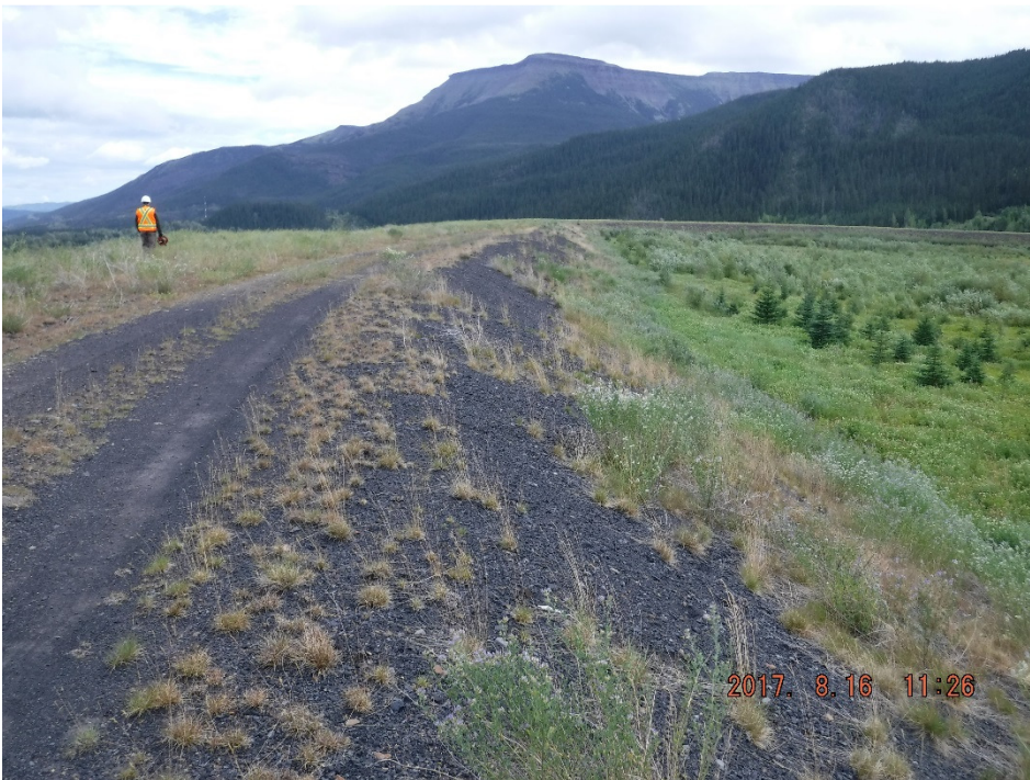
Photo II-4 BTD crest and upstream slope - looking northeast; no sign of distress (BTD-2017-03)
