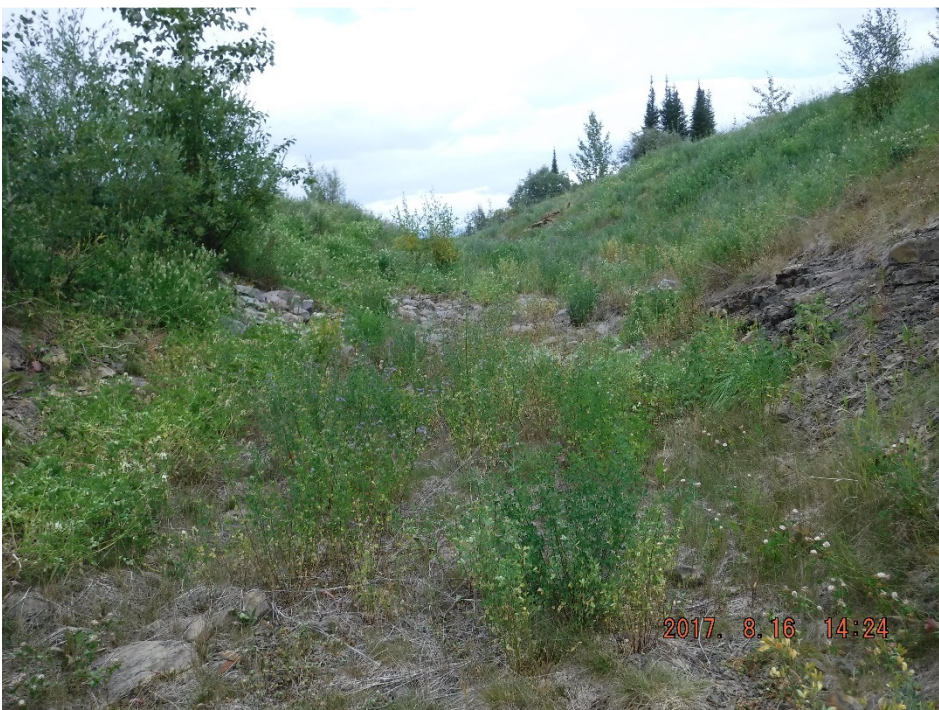
Photo II-27 Spillway inlet – looking northeast. Vegetation is well established; no major obstructions (BTD-2017-22)
