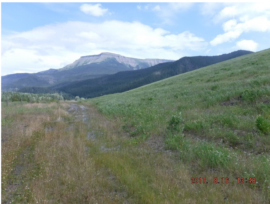
Photo II-21 Upper portion of the downstream slope – looking northeast. Slope is in good condition with no significant sign of erosion or movement (BTD-2017-17)
