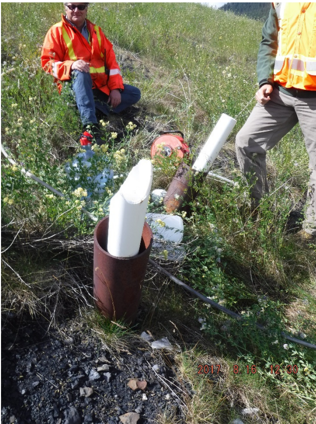
Photo II-8 Standpipe piezometers PA-1 and PA-2. PA-1 top of casing requires repair.
