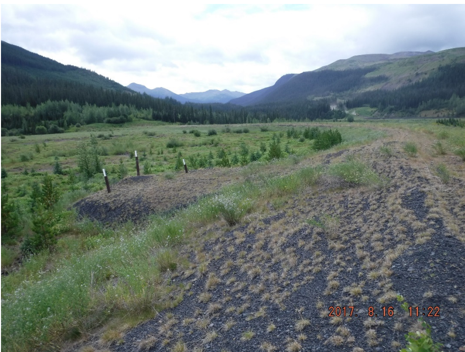
Photo II-3 Overview of upstream slope - looking southwest. Slope is in good condition and no sign of distress (BTD-2017-02)
