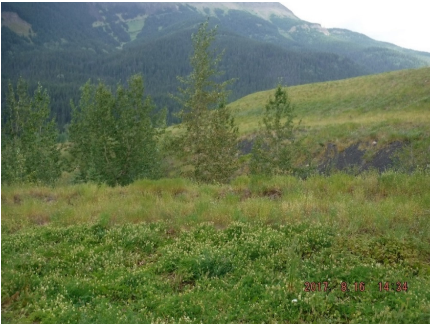
Photo II-31 Toe of the dam along west slope is approximately 1.5H:1V – possibly used as an end dump prior to closure. The slope appears to be stable with no significant sign of erosion or movement (BTD-2017-25)
