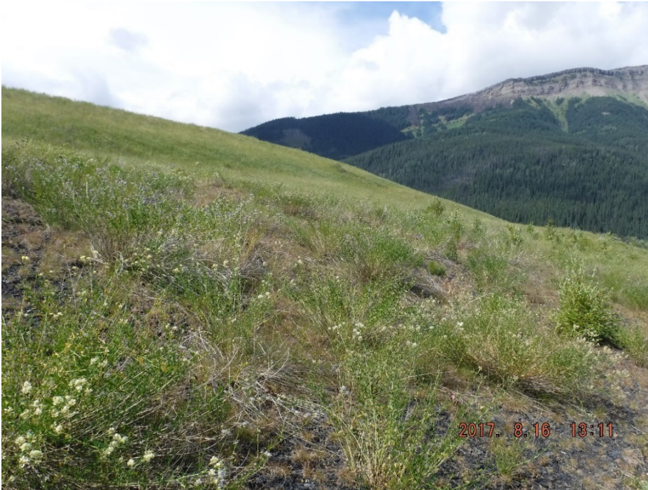
Photo II-16 Overview of the lower portion of the downstream slope – looking northwest. Slope is in good condition with no significant sign of erosion or movement (BTD-2017-13)
