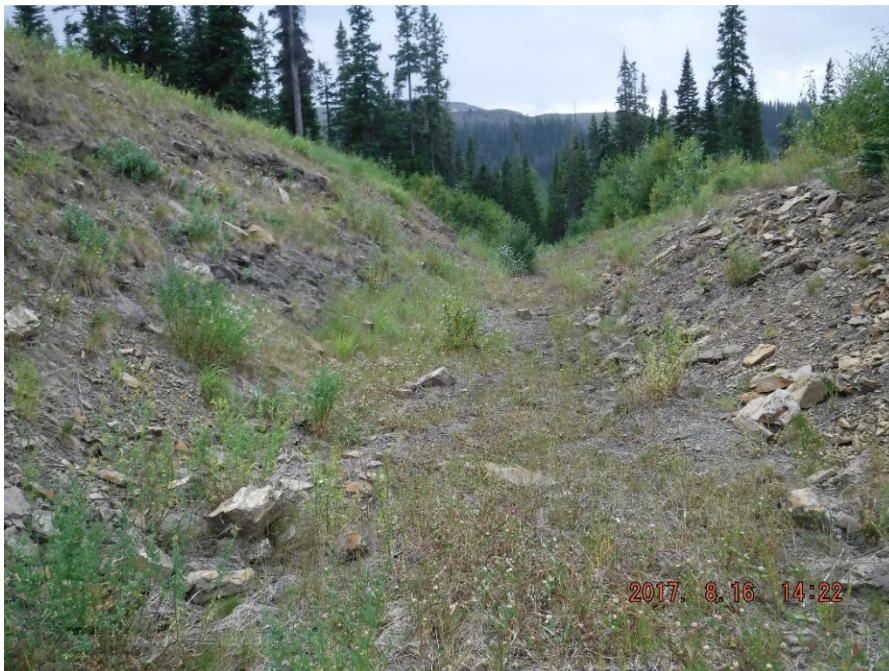
Photo II-25 Spillway channel - looking downstream where channel transitions from riprap lined (invert and right bank) and bedrock (left bank) to channel being entirely in bedrock (BTD-2017-21)
