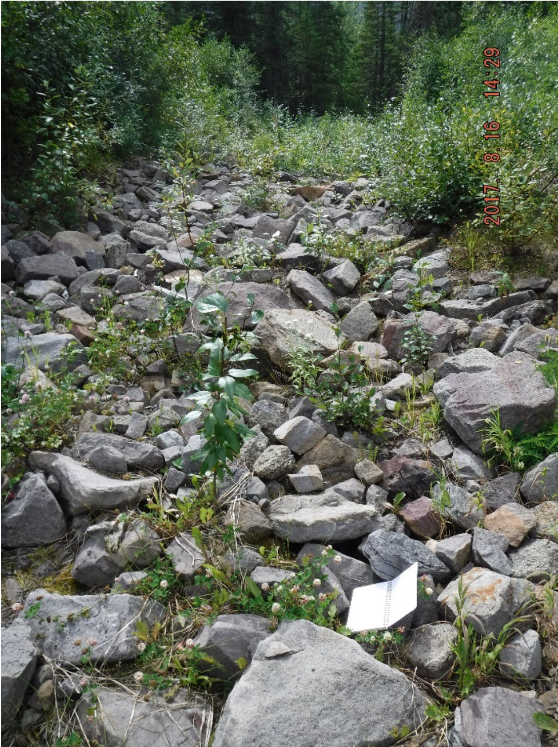
Photo II-29 Spillway channel looking downstream after transition from bedrock to riprap. Channel is armoured with riprap on the invert and side slopes (BTD-2017-23)
