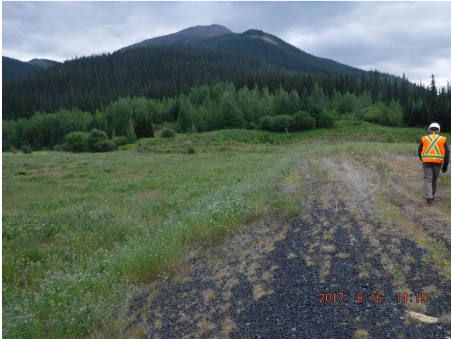
Photo II-24 Upstream slope – looking southeast. Tailings surface elevation is approximately 2 m lower than the crest elevation (BTD-2017-20)
