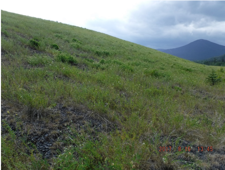
Photo II-20 Upper portion of the downstream slope – looking southwest. Slope is in good condition with no significant sign of erosion or movement (BTD-2017-16)
