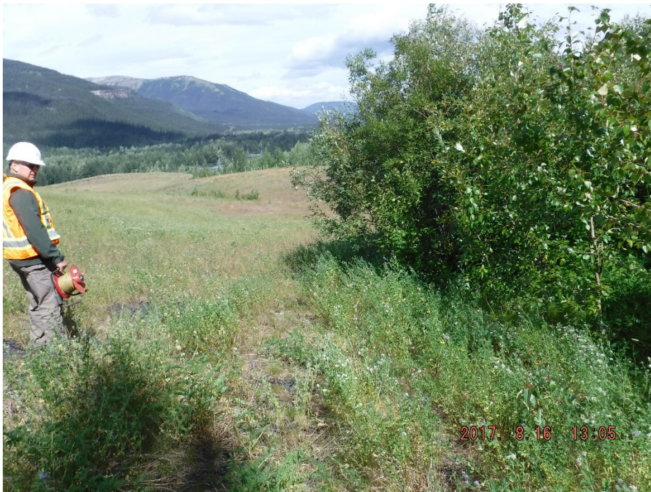
Photo II-13 Looking northeast along the downstream slope and east abutment contact – vegetation is well established (BTD-2017-10)
