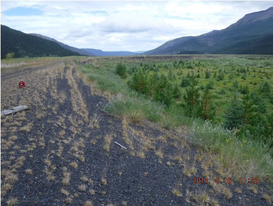
Photo II-2 Overview of upstream slope - looking northeast. Slope is in good condition and no sign of distress (BTD-2017-02)
