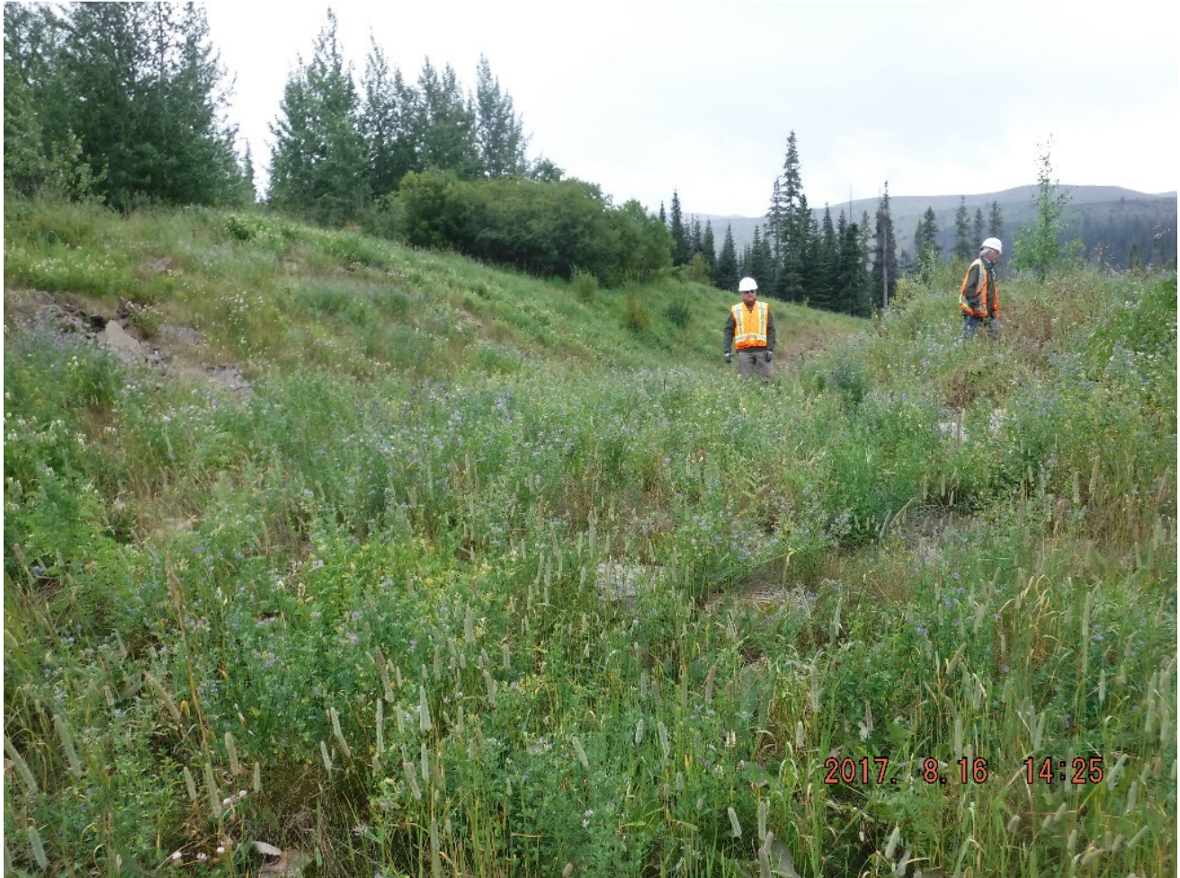
Photo II-28 Spillway inlet – looking southwest. Vegetation is well established; no major obstruction (BTD-2017-22)
