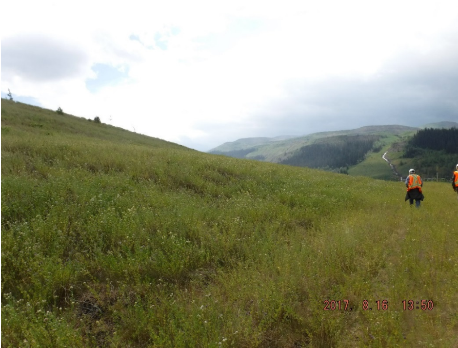
Photo II-22 Downstream slope – looking southwest. Slope is in good condition with no significant sign of erosion or movement (BTD-2017-18)
