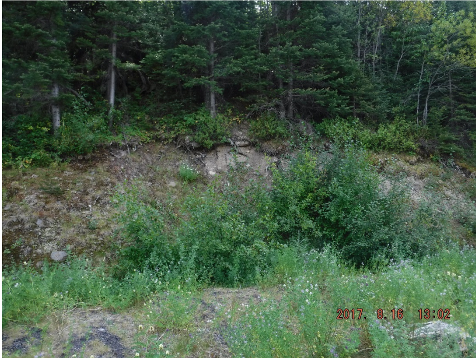
Photo II-12 Over view of BTD east abutment – more vegetation than 2016 (BTD-2017-09)
