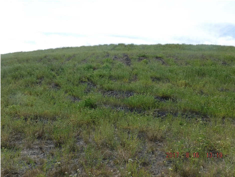
Photo II-18 Overview of the upper portion of the downstream slope – possible slope break observed likely due to normal soil erosion and rilling (BTD-2017-14)
