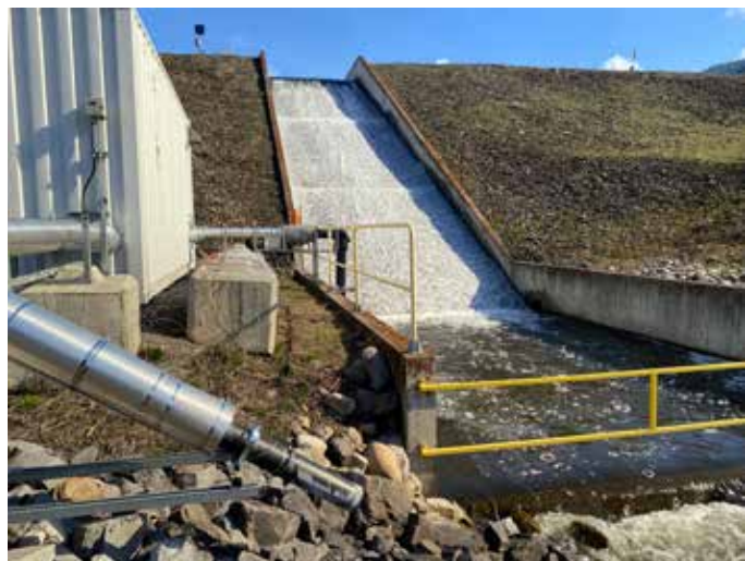
Antiscalant facility at lower Greenhills Creek.
