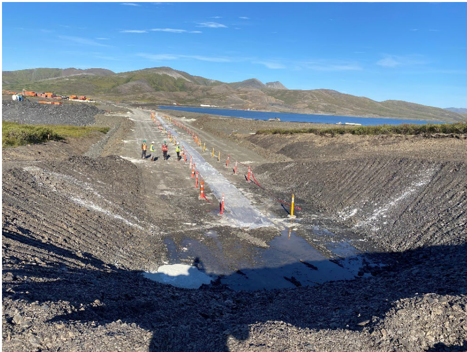
Photo 22: East Abutment and Standing Water from Seep
