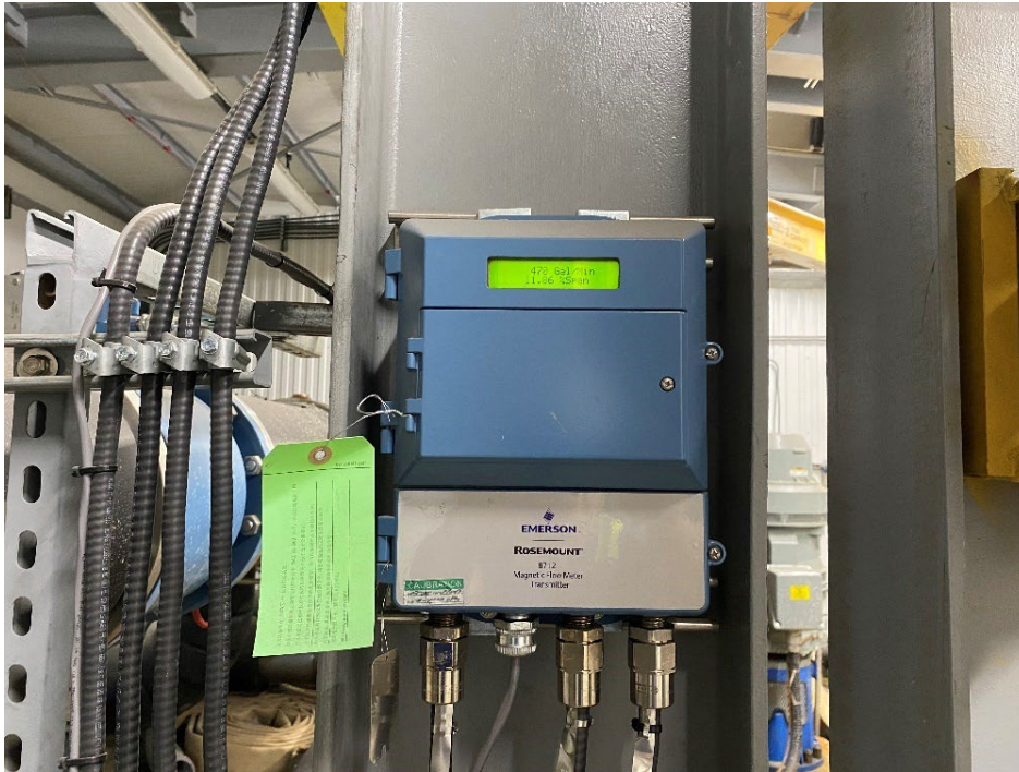
Photo 13: Flow Meter Inside of Pumphouse
