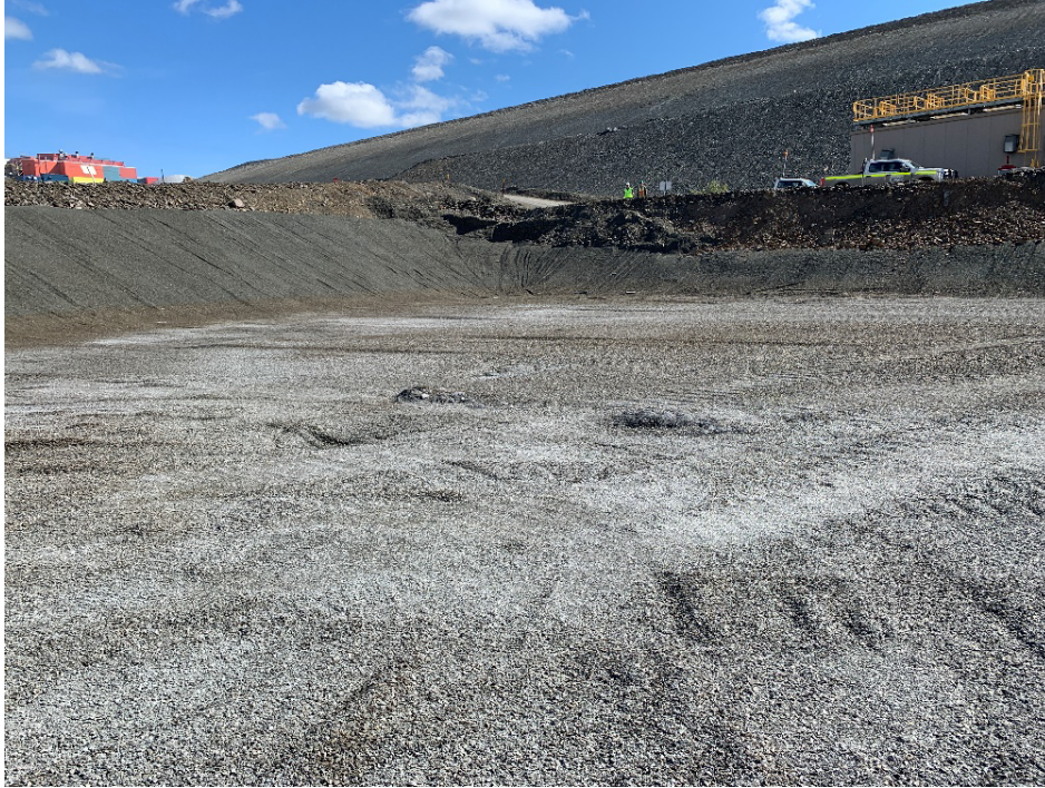
Photo 9: Divots in Seepage Collection Pond Cover Soil
