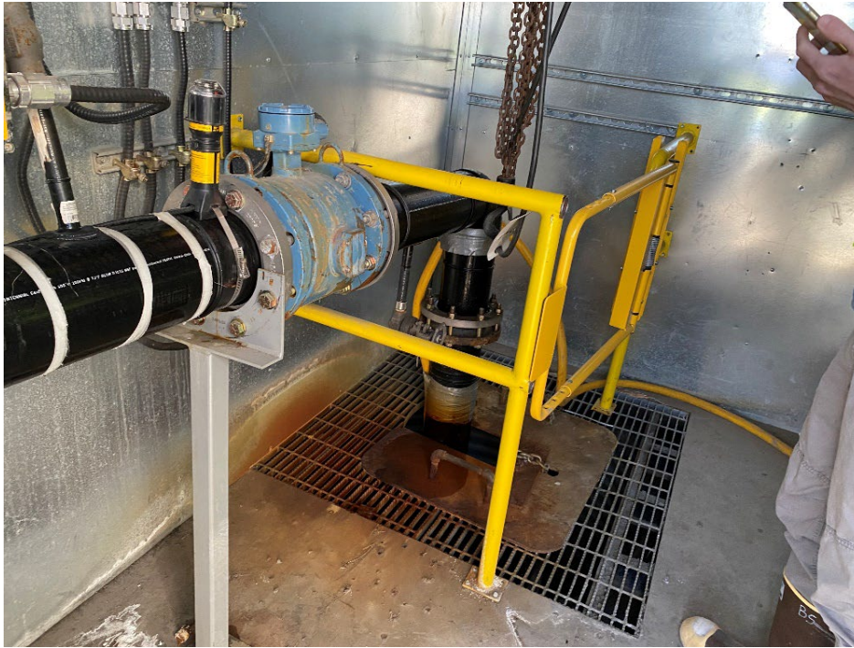
Photo 13: Sump Pump Pipe and Flow Meter Inside Pumphouse
