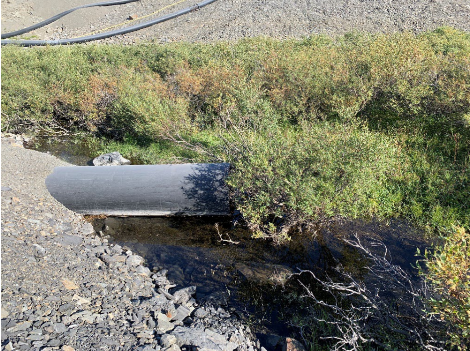
Photo 24: Close Up of Upper Bons Creek Culvert Inlet Downstream of Back Dam
