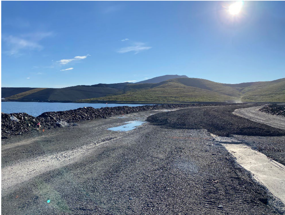
Photo 16: Dam Crest, Cut-off Wall, and Initial Lift of Insulation Layer Fill near Station 28+00
