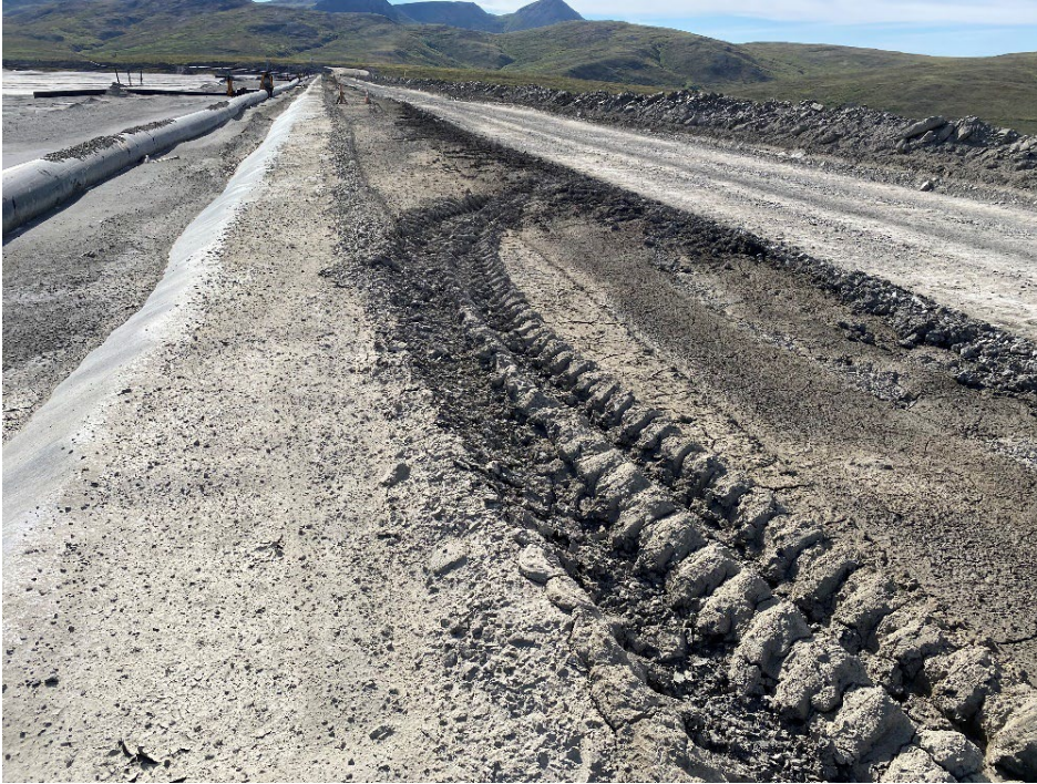
Photo 3: Equipment Tire Tracks near Geomembrane Liner at Embankment Crest
