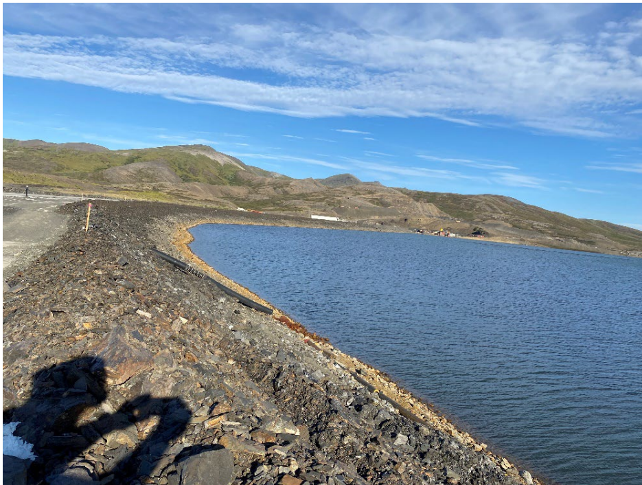
Photo 14: Sump Pump Discharge Pipe and Upstream Slope near Station 27+00
