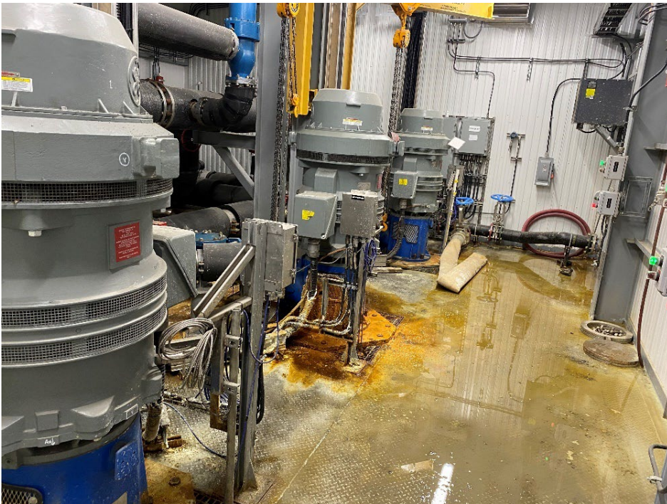
Photo 12: Turbine Pumps inside of Pumphouse
