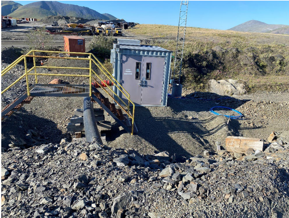
Photo 12: Sump Pumphouse and Discharge Pipe near Station 26+50
