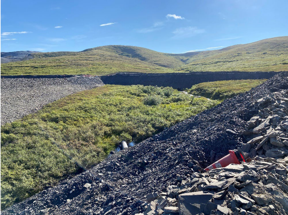
Photo 23: New Transportation Corridor and Upper Bons Creek Culverts Downstream of Back Dam
