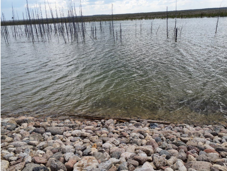
Photo II-19 North Dyke – looking south at the 2021 riprap and the trees in the pond
