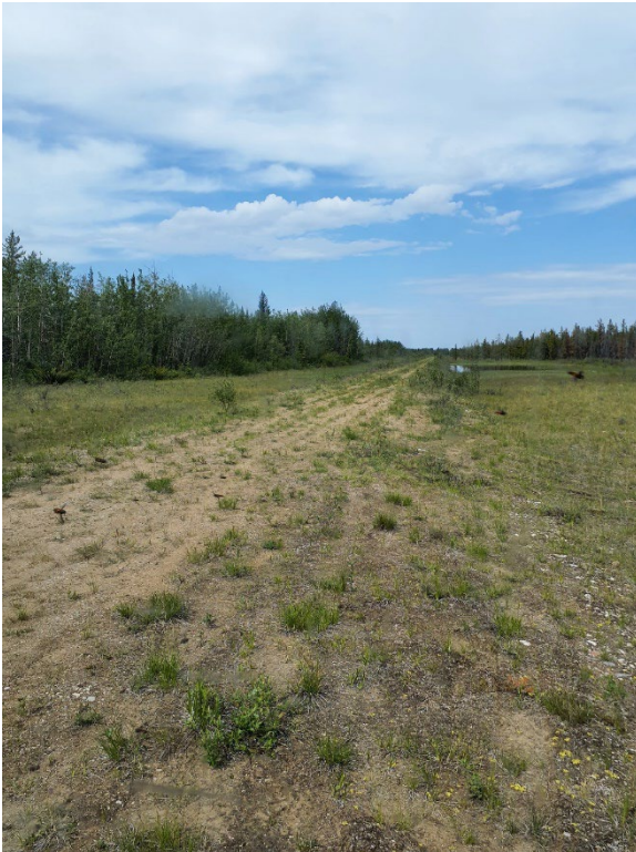
Photo II-22 East Dyke – looking north at the downstream slope and at the permanent pond located at the downstream toe
