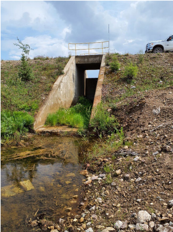
Photo II-25 Main Pond Spillway – looking south into the spillway and at the material at the outlet
