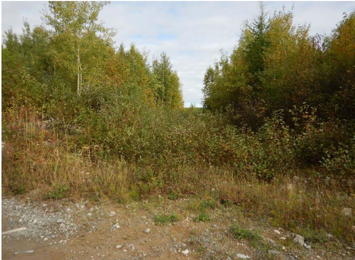
Photo 5 :Emergency spillway located between Dams 1D and 1E was in good condition but exhibited significant vegetation growth. Vegetation in the downstream channel was cleared later in 2022, after this inspection.
