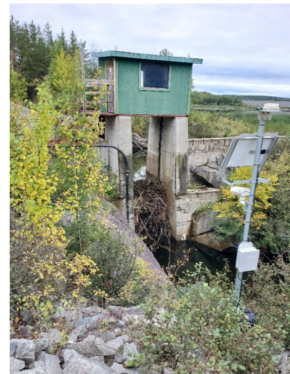
Photo 12 : Dam 4B main spillway – accumulation of debris showing beaver activity in the spillway. It is noted that this debris was removed later in 2022, subsequent to the site inspection.
