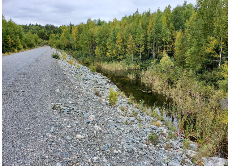
Photo 9 : Dam 2A – View of the water accumulation at the toe of the dyke, essentially unchanged since 2021.
