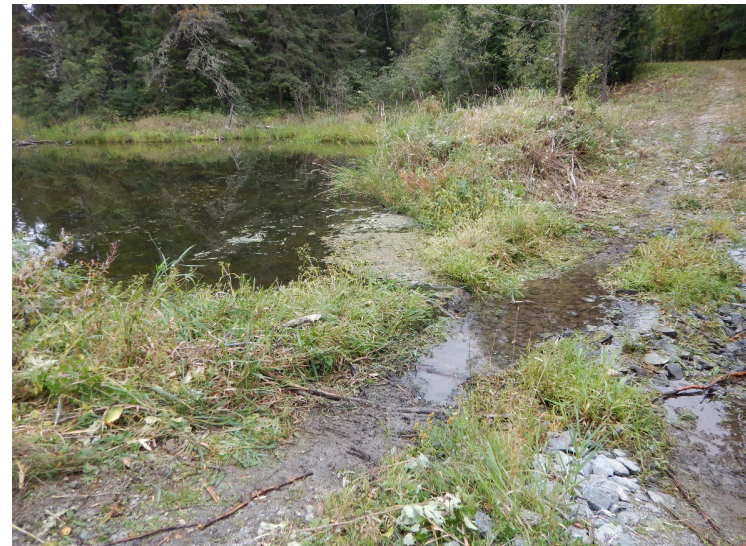
Photo 15 : Foot of dam 4B. Beaver blockage of 2021 removed, with no recurrence of the blockage at the time of 2022 inspection.
