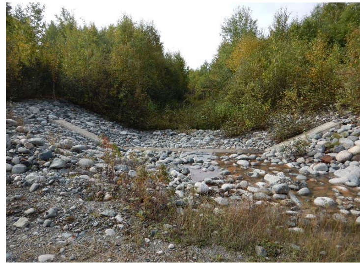
Photo 4 : Emergency spillway located between Dams 1D and 1E was in good condition but exhibited significant vegetation growth. Vegetation in the upstream channel was cleared later in 2022, after this inspection.
