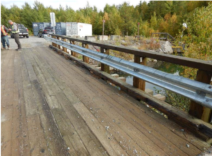
Photo 6 : Access bridge close to the TSF spillway. Bridge appears in good condition, although the edge blocks appear to be suffering some scraping, presumably by snow removal equipment.
