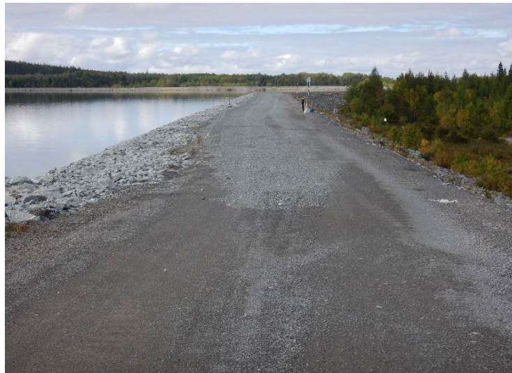
Photo 2 : Dam 1C - Rip rap was recently replaced and traffic gravel was placed on the crest.
