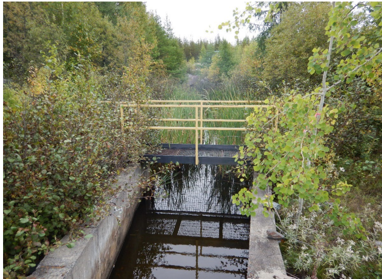
Photo 13 : Dam 4B – Downstream view of the spillway. Outflow channel from the spillway to the Parshall flume contains significant vegetation
