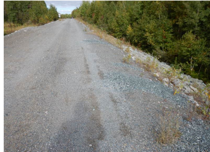
Photo 7 : Crest erosion was nominal, with conditions similar to 2021 when repair was performed.
