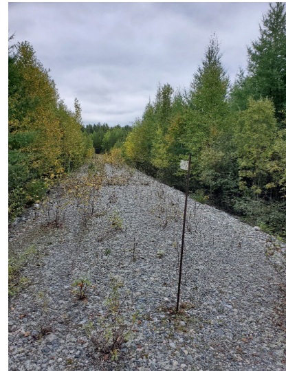
Photo 11 : Dam 4A which does not currently retain water. Note: limited vegetation on slopes and ridge.
