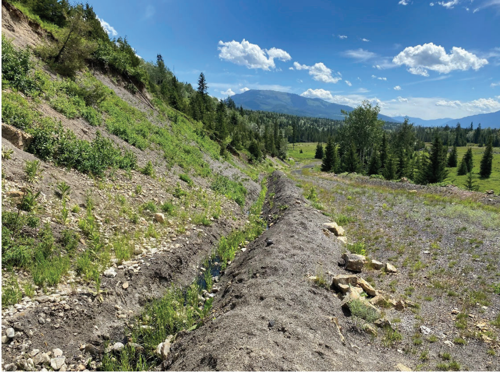
Photo 40. Ditch on upstream side of the abandoned mine access road, looking southeast
