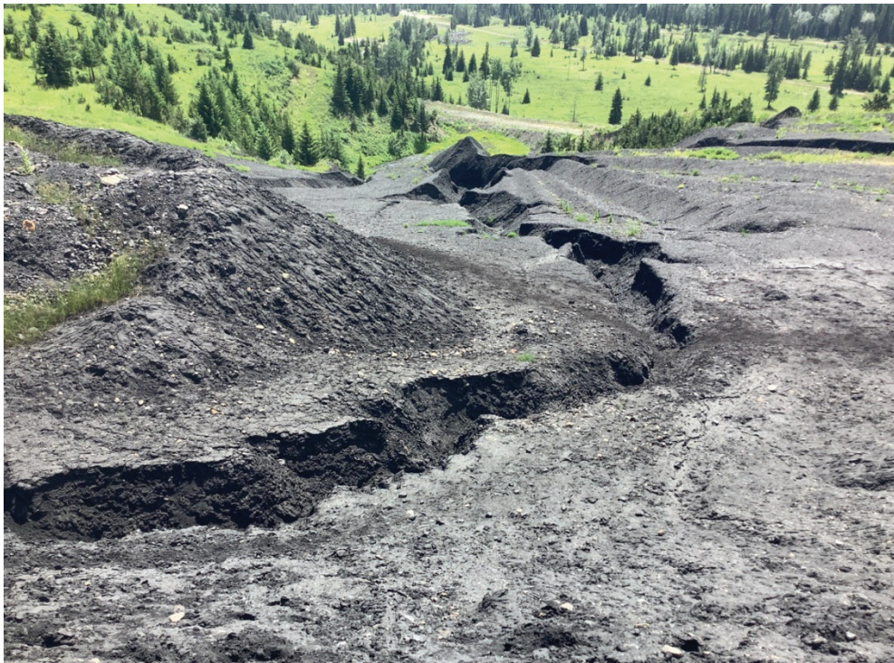
Photo 49. Erosion gullies at the toe of the Lower Bench, looking southwest
