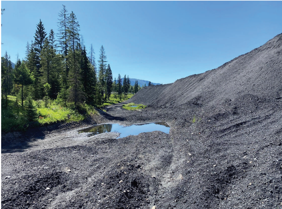
Photo 38. Water pooling along the downstream toe along eastern extents of the ERX, looking south
