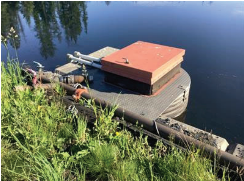
Photo 68. Stilling well containing water level sensors in Pond C, looking north
