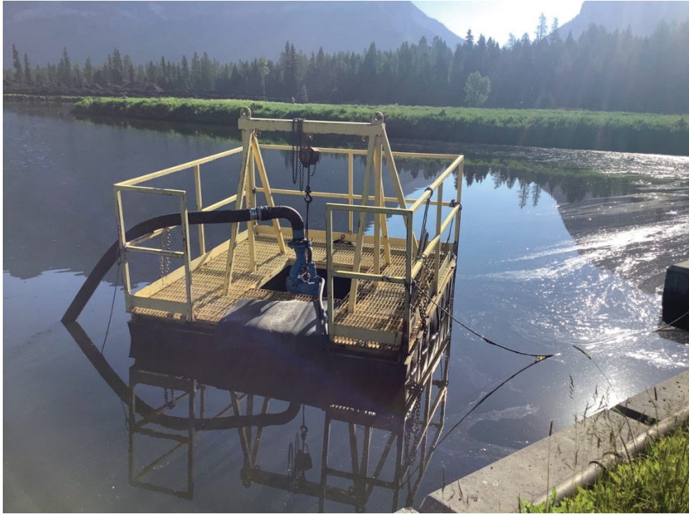
Photo 67. Reclaim pump and barge in Pond C, looking northwest
