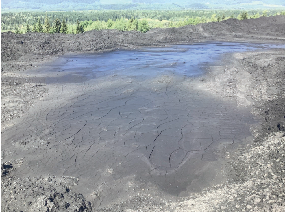
Photo 19. Evidence of water pooling on the 1270 m bench, looking southwest
