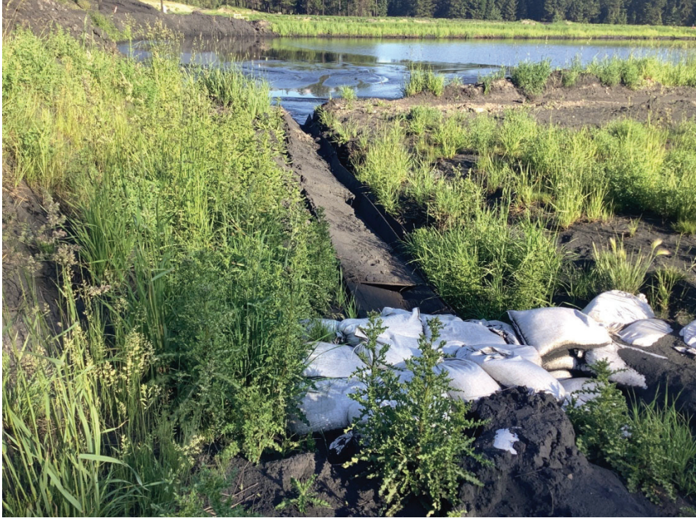
Photo 63. Box culvert containing discharge pipe between Pond A and Pond B, looking west
