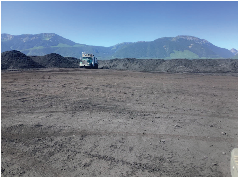
Photo 32. Hydro-vac material being deposited near the crest of the 1300 m bench, looking southwest
