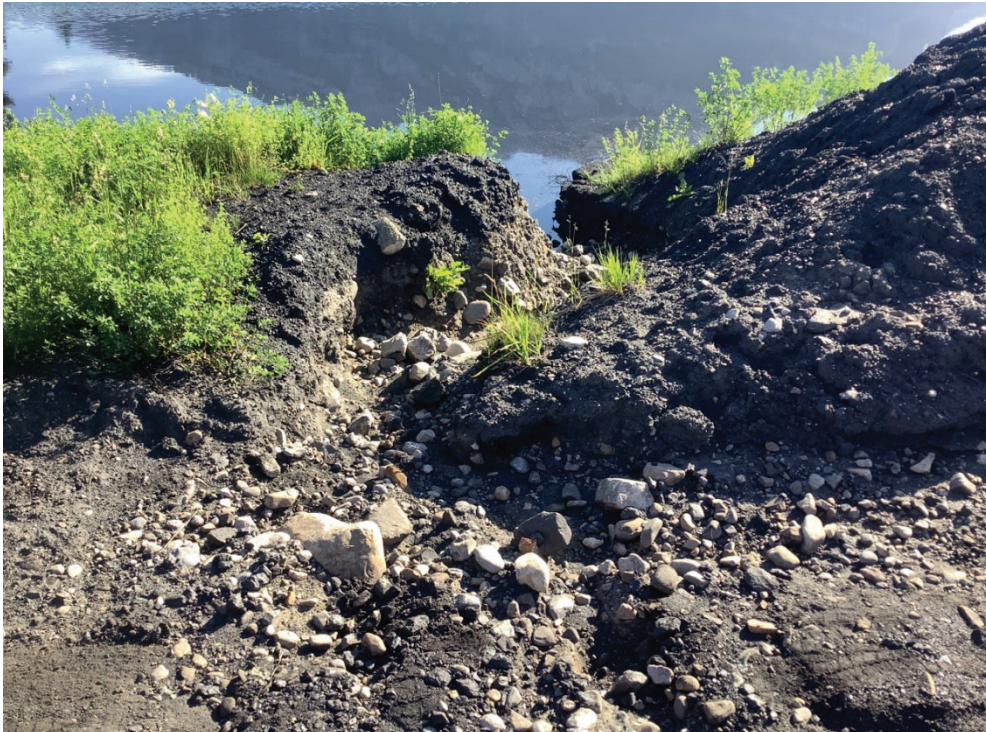
Photo 70. Erosion along the upstream slope of the Pond C, looking northwest
