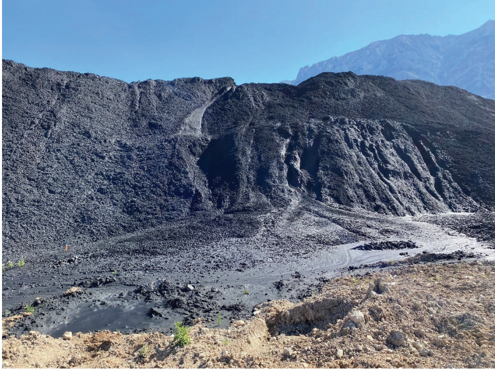
Photo 15. June 14, 2022 washout location, looking northeast
