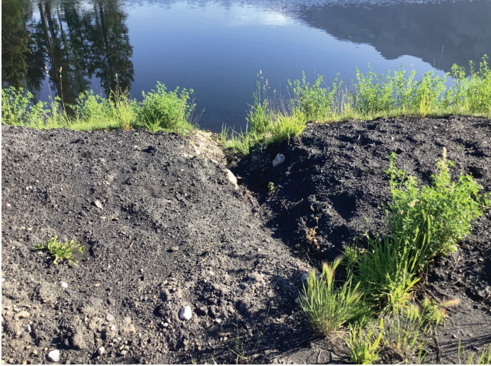
Photo 69. Erosion along the upstream slope of the Pond C, looking northwest
