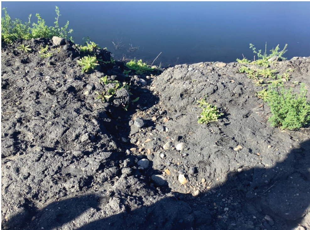
Photo 78. Erosion along the upstream slope of the Pond C, looking southwest
