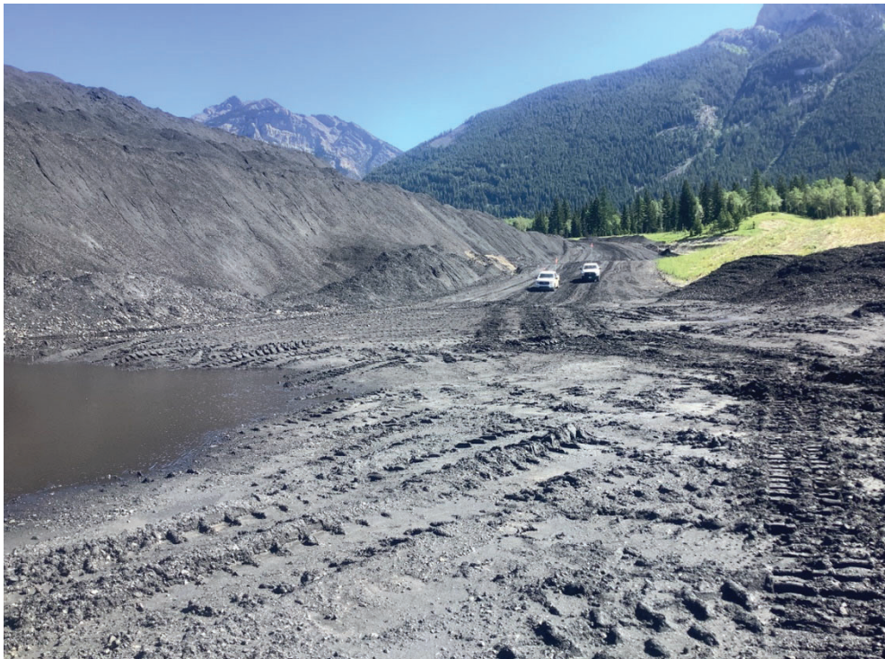
Photo 22. Infiltration sump along toe of the 1285 m bench, looking northeast
