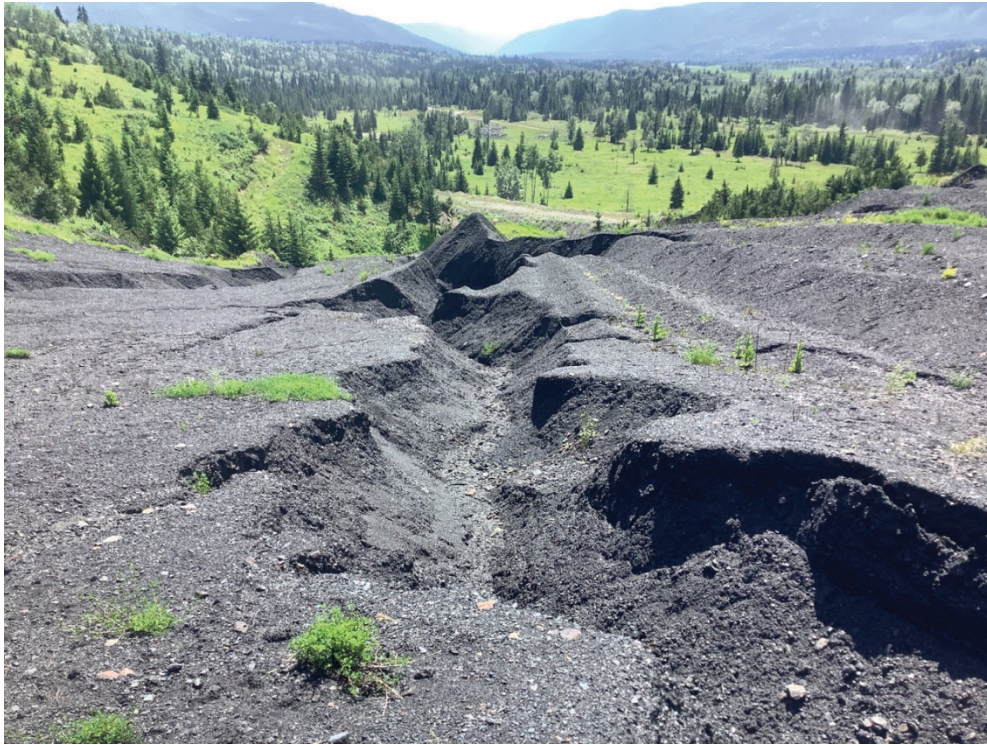
Photo 48. Erosion gullies at the toe of the Lower Bench, looking south
