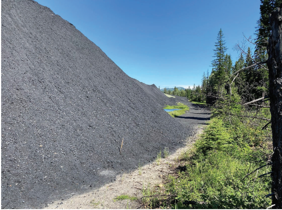
Photo 37. Water pooling along the downstream toe along eastern extents of the ERX, looking north
