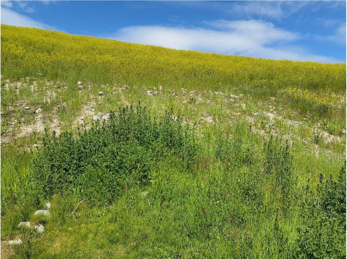
Photo I-A-8 Place where outlet of culvert below starter dam should be located. Culvert outlet was not seen which suggests it is now buried, likely during reclamation. No issues of concern were observed in area. (TRJ-2022-06)
