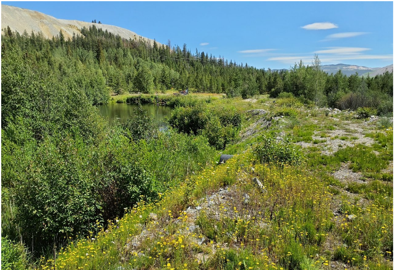
Photo I-C-1 Overview of Lower Trojan Dam crest from right abutment. Crest is uneven and appears to be sloped (rises from left abutment to right abutment) (TRJ-2022-09)
