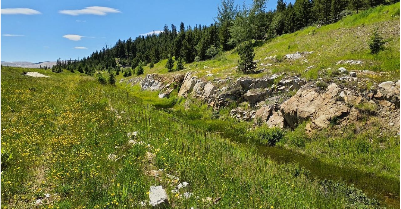
Photo I-A-6 Upper segment of spillway downstream of approach channel, looking toward southwest (top) and looking toward northeast (bottom). HVC provided a photograph to show that vegetation was cleared after site visit. (TRJ-2022-04)
