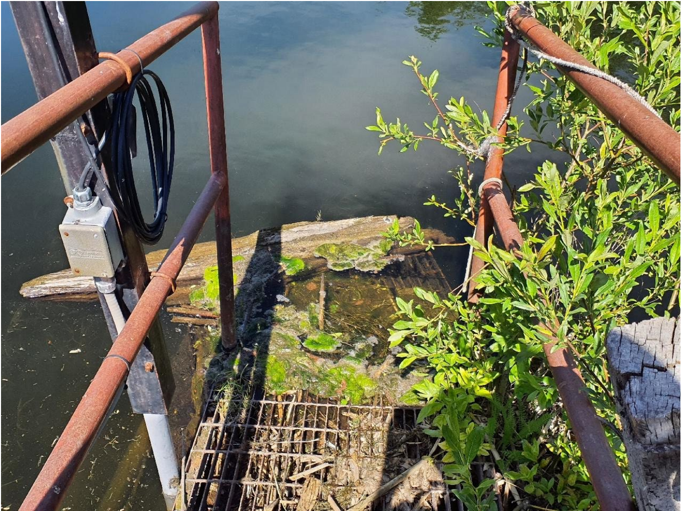
Photo I-C-8 Low-Level Outlet inlet. During the site visit HVC cleared vegetation accumulated on the LLO intake as a routine maintenance task. Subsequent to the site visit, HVC repositioned the debris boom so it was protecting the intake of LLO which is also a routine task. (TRJ-2022-12)
