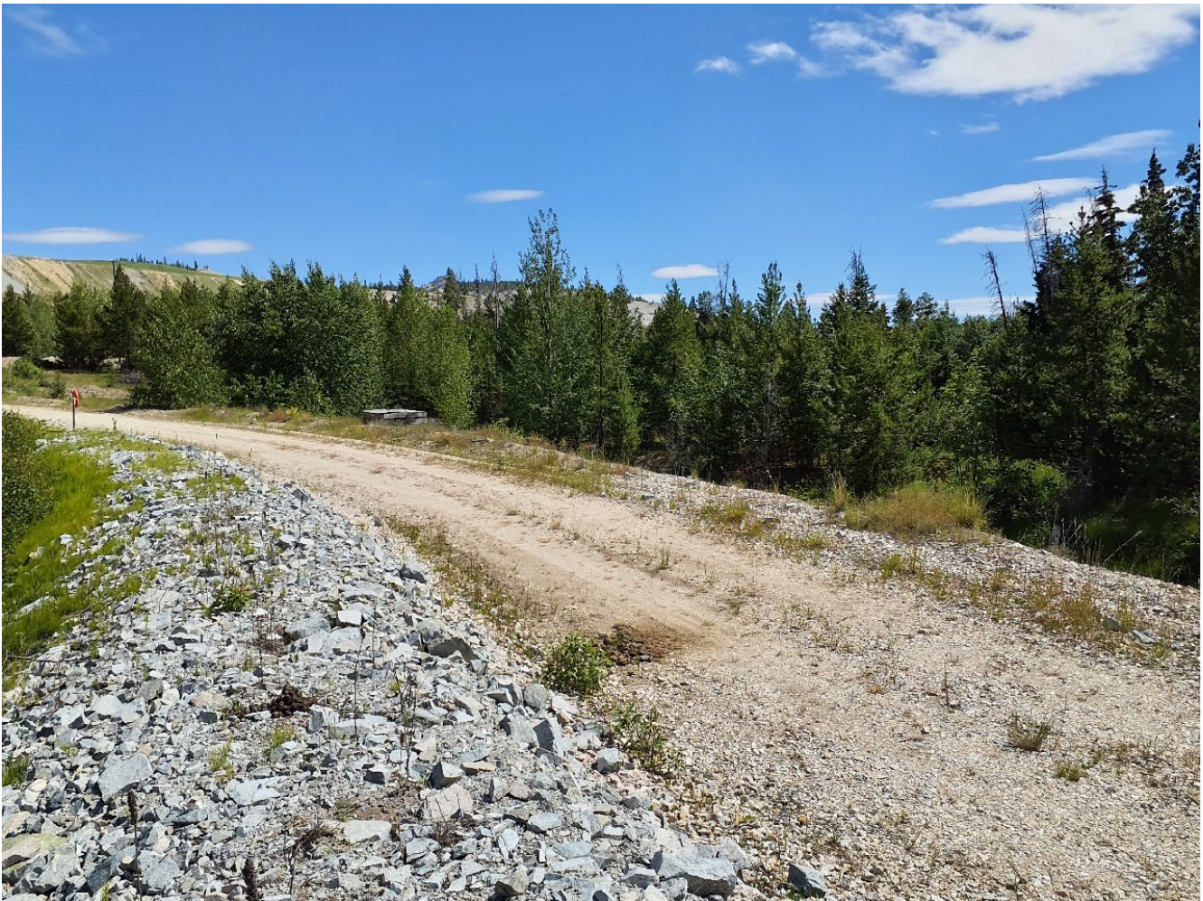
Photo I-B-1 Overview of R4 Seepage Pond Dam crest and downstream slope looking towards left abutment (TRJ-2022-07)
