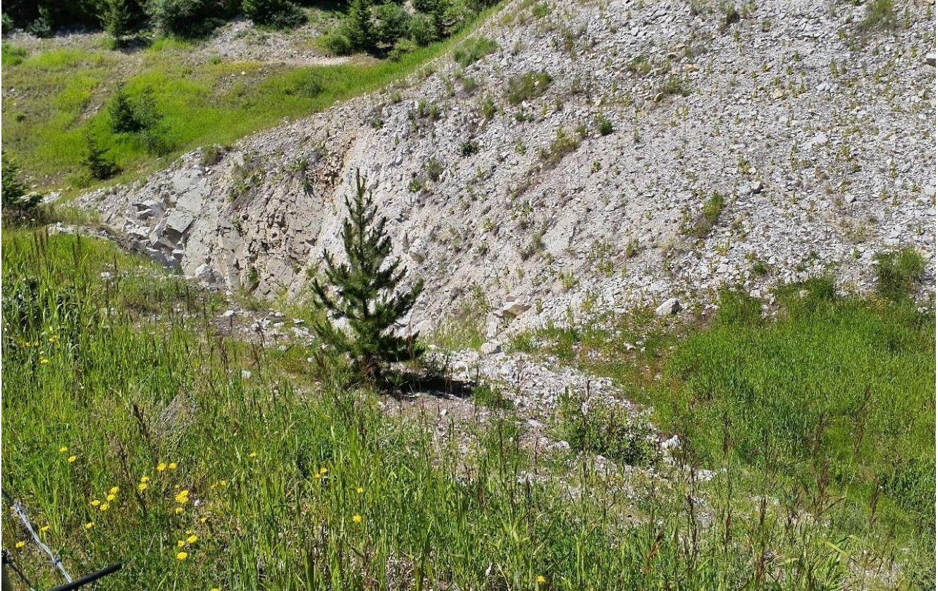
Photo I-A-7 Overview of spillway channel downstream of rock chute, near transition to riprap segment, looking toward south (top) and looking north (bottom). (TRJ-2022-05)
