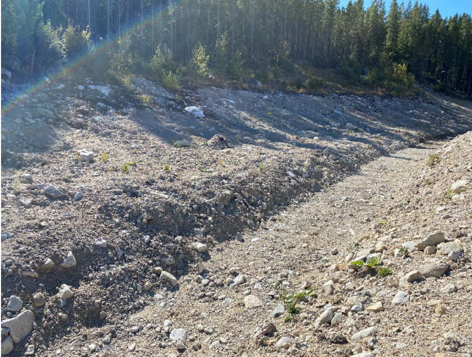
Photo I-B-15 Mystery Creek diversion excavated to replace decommissioned Mystery Creek culvert. In November 2022, as recommended by EoR, HVC installed a geomembrane liner over the segment of ditch excavated in fill (shown in photo) to reduce seepage losses. (HH-2022-06)
