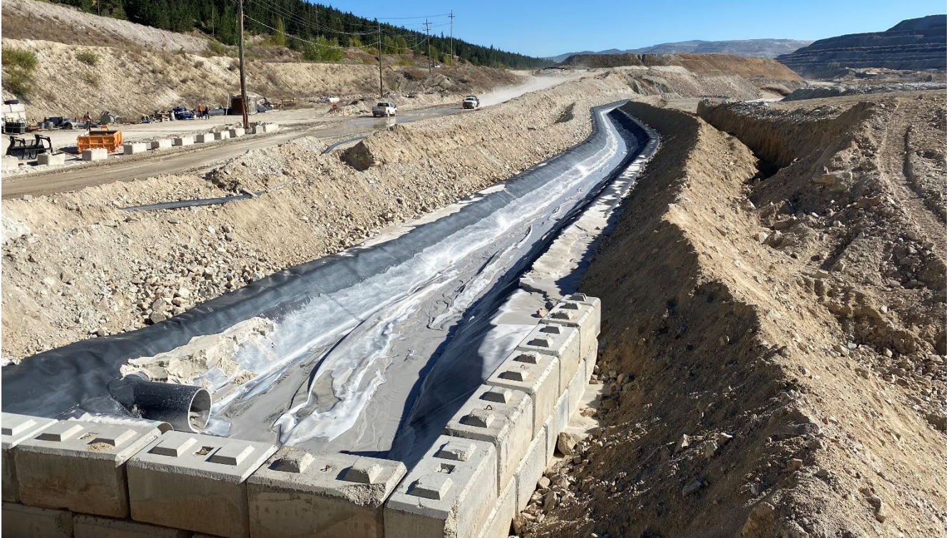
Photo I-B-14 Upstream segment of the replacement discharge channel, built in 2022, to convey overflow from HH Pumphouse to 24 Mile TSF. (HH-2022-07)
