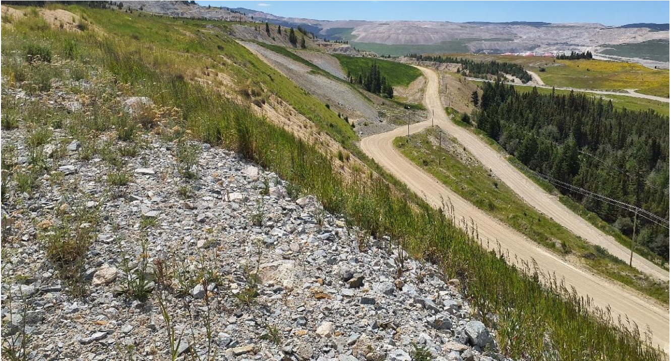
Photo I-A-4 Overview of downstream slope and toe area and of previously documented erosion area. Cracking remains filled, indicating area has been inactive (BTH-2022-04)
