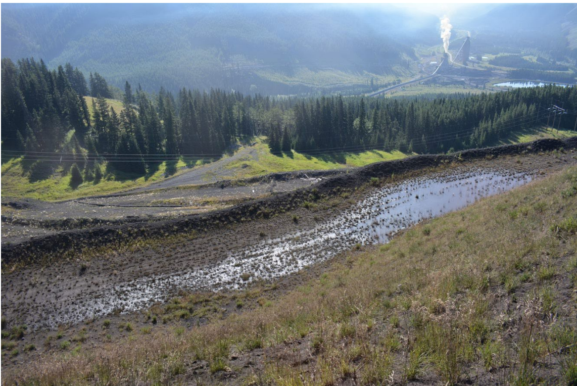
Photograph 34: Site C CCR Facility – Surface Water Ponding on Intermediate Bench Above Bench with Observed Cracking, Looking south, 30 August 2022
