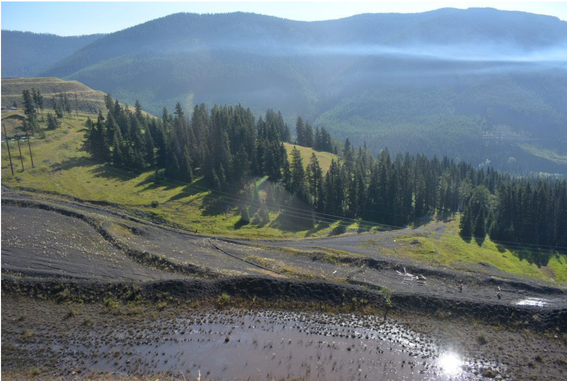
Photograph 35: Site C CCR Facility – Surface Water Ponding on Intermediate Bench Above Bench with Observed Cracking, Looking southeast, 30 August 2022
