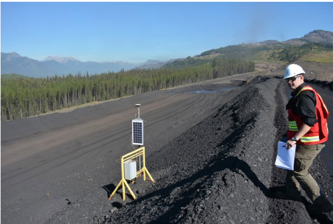
Photograph 22: West Tailings Dam – Downstream Slope and Vibrating Wire Piezometer; Looking North, 30 August 2022
