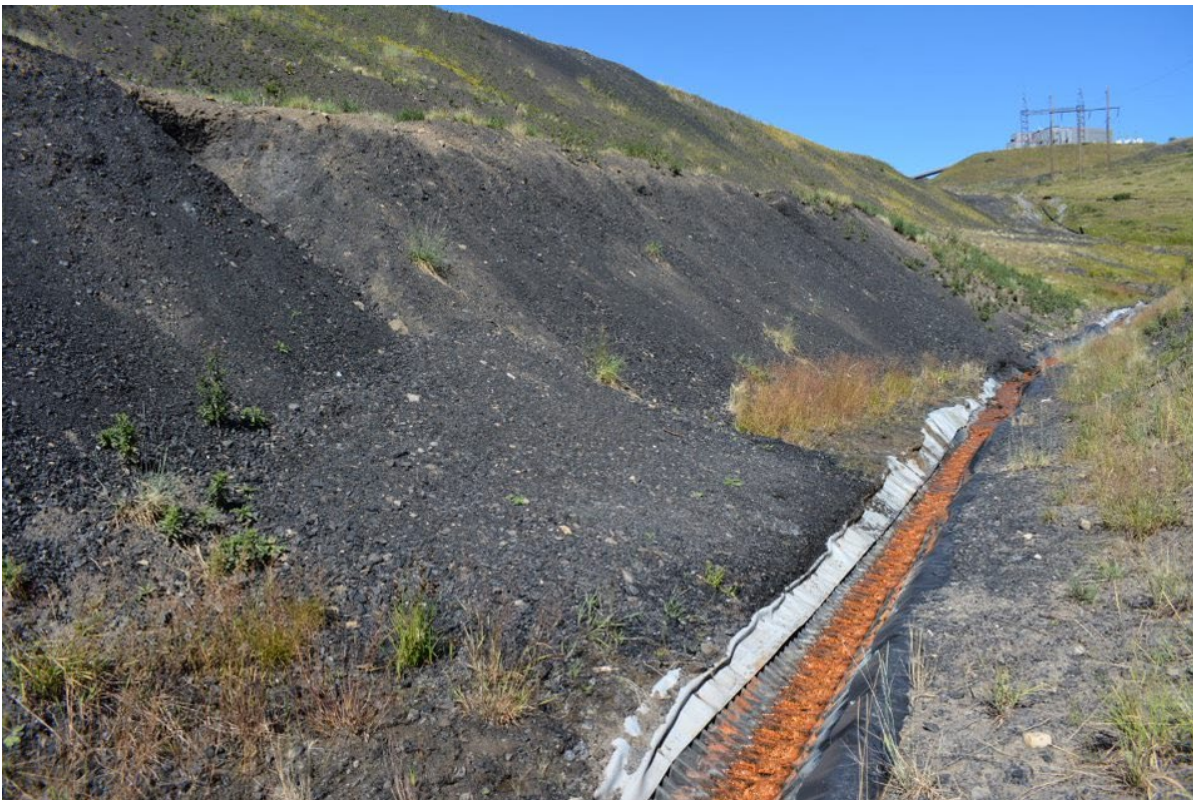
Photograph 30: Site C CCR Facility – Smart Drain at Toe, Looking Northeast, 30 August 2022
