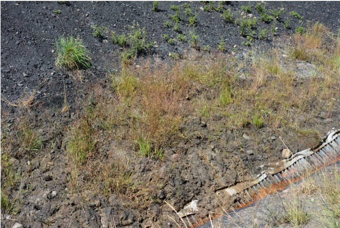
Photograph 31: Site C CCR Facility – Partial sloughing into Smart Drain at Weir Inlet, Looking North, 30 August 2022
