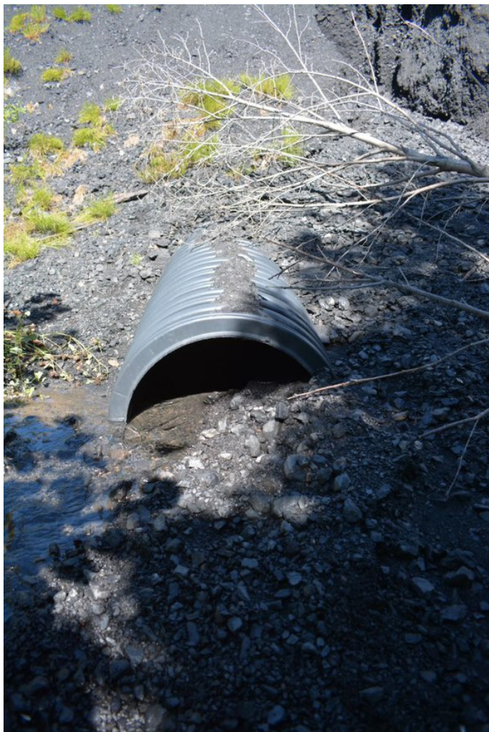
Photograph 23: Site E CCR Facility – Partially Obstructed Surface Water Culvert, Looking North, 31 August 2022
