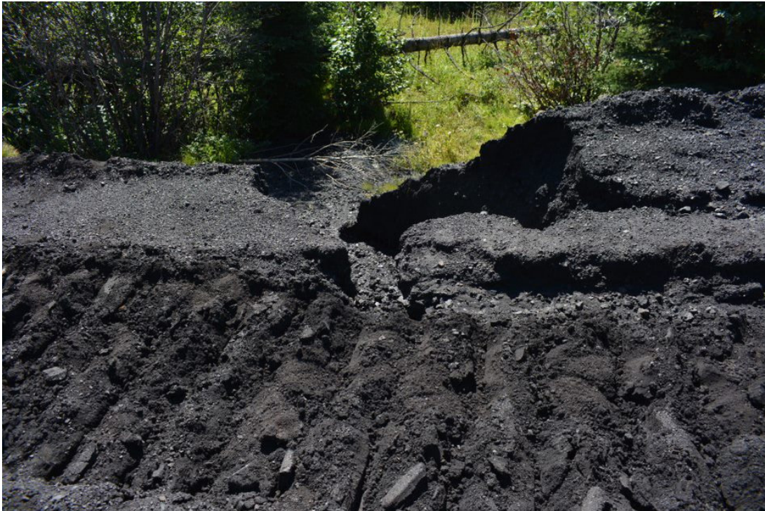
Photograph 22: Site E CCR Facility - Erosion adjacent to the Surface Water Culvert, Looking South, 31 August 2022
