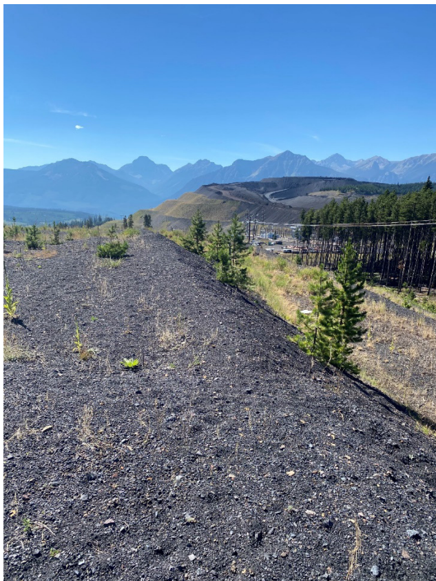
Photograph 6: Site A CCR Facility – Downstream Slope; Looking Southwest (Site C & D CCR Facilities in background), 30 August 2022
