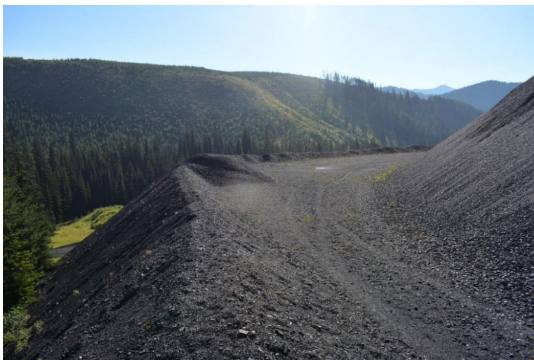
Photograph 16: Site B CCR Facility North and East Extension Lower Bench, Looking East, 31 August 2022
