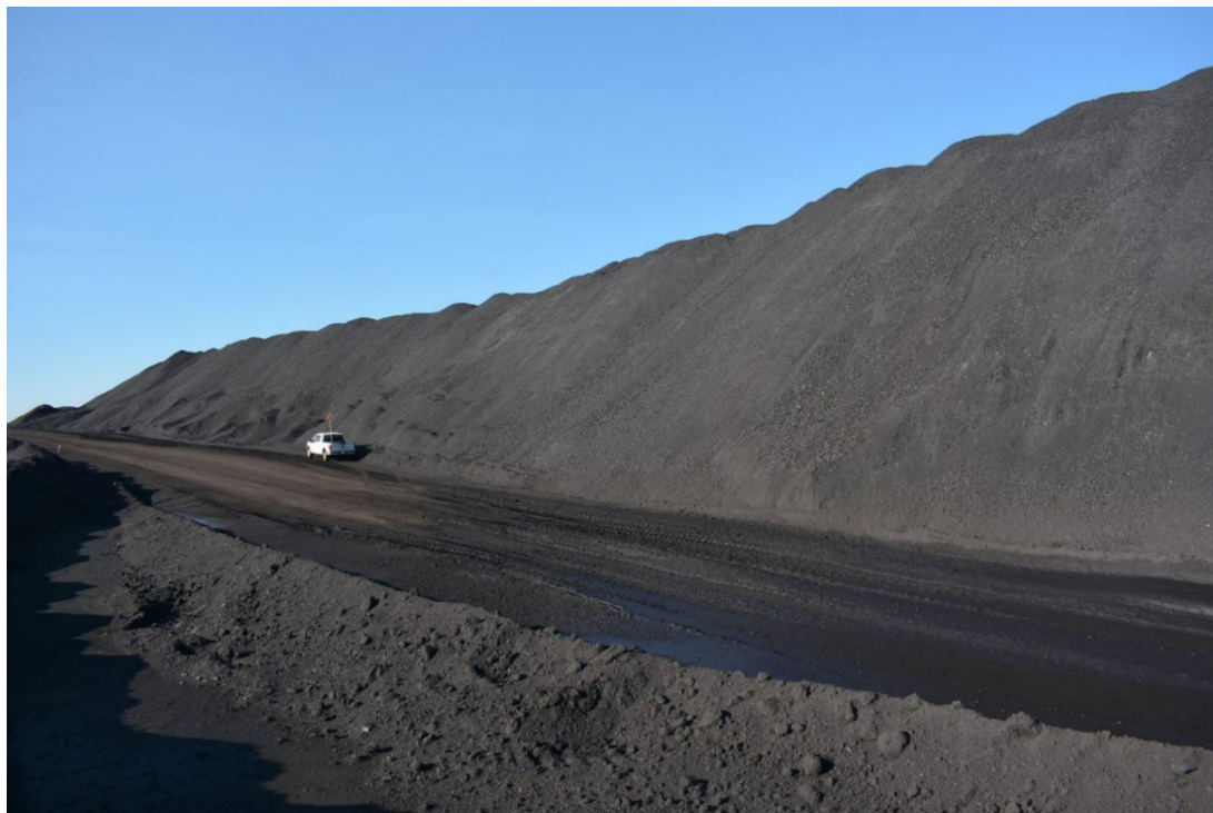
Photograph 11: Site B CCR Facility – Repaired Erosion Area on east side of haul road, Looking Southeast, 31 August 2022
