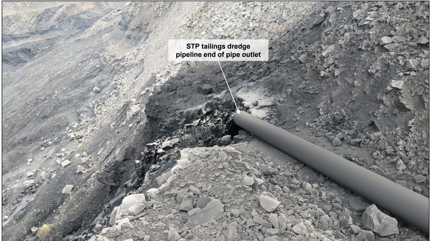
Discharge of tailings from the South Tailings Pond at the tailings dredge pipeline end of the pipe outlet into the Turnbull TSF, looking southeast.
