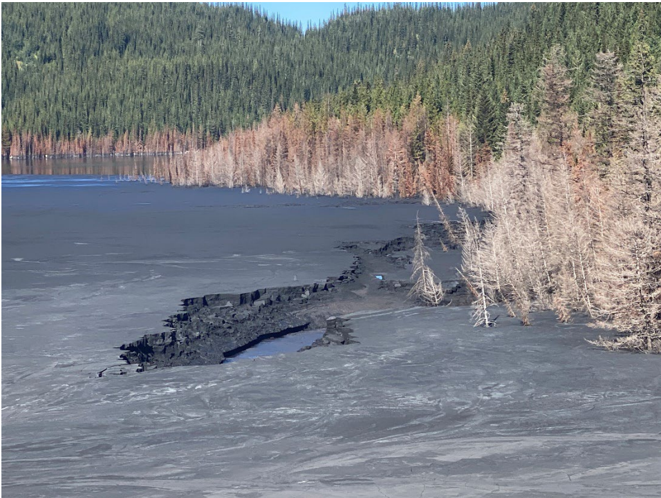
Photo IW-18 WFTF receding incised channel. (Looking north – Taken 21 September 2022)
