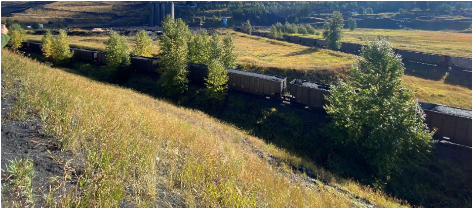
Photo IB-5 Lagoon B crest and surface typical conditions. (Looking SE, from Lagoon C crest – Taken 20 September 2022)
