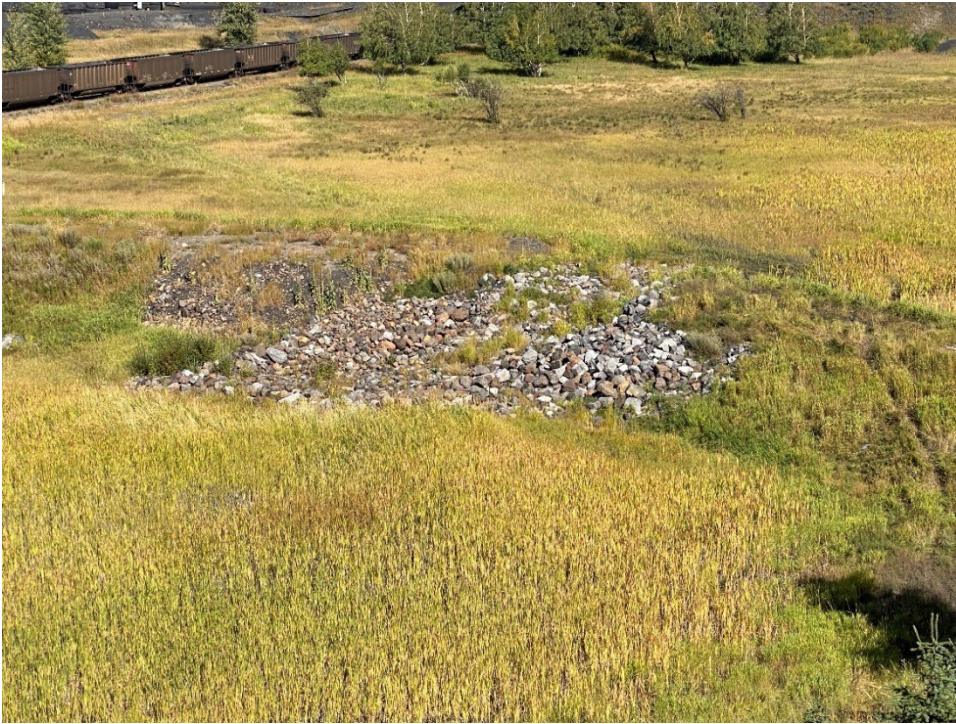
Photo IA-3 Lagoon A crest and spillway riprap. (From Lagoon D, looking NE – Taken 20 September 2022)
