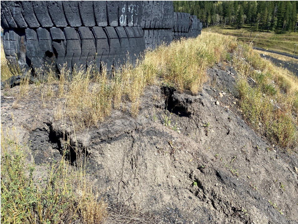
Photo ID-16 Lagoon D minor crest erosion. (Looking NE – Taken 20 September 2022)
