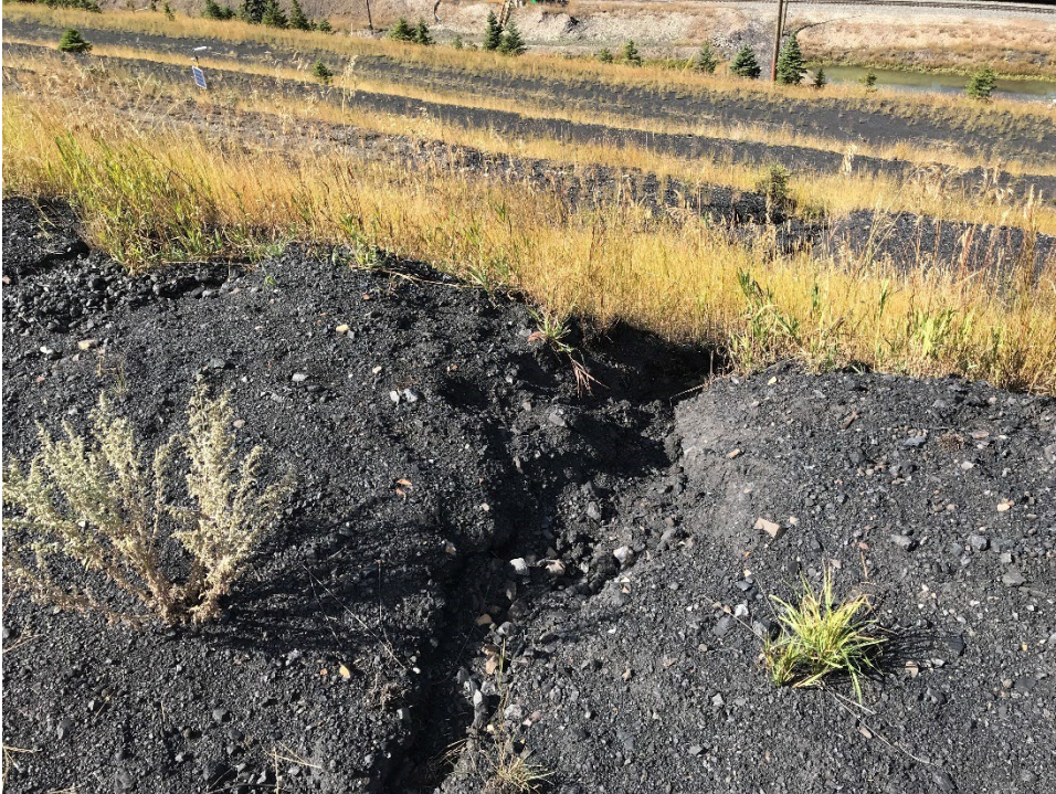
Photo ID-15 Lagoon D minor bench minor erosion. (Looking NW – Taken 20 September 2022)
