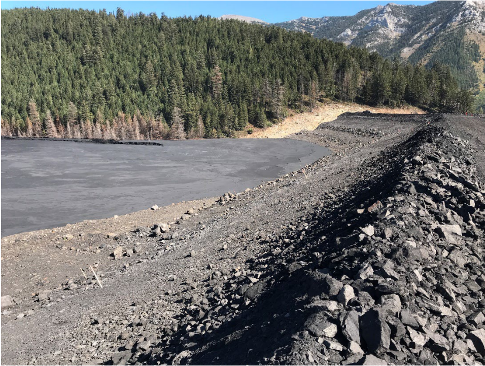
Photo IW-7 WFTF embankment tailings contact and typical upstream slope. (Looking east – Taken 21 September 2022)
