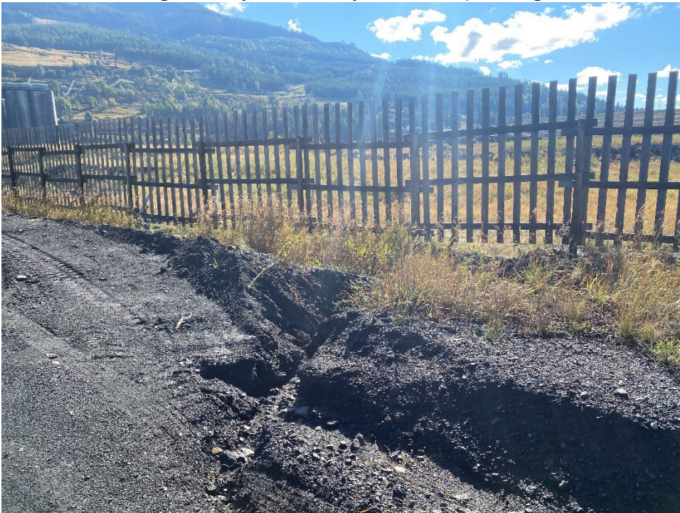
Photo IC-10 Lagoon C upstream slope erosion. (Looking SE – Taken 20 September 2022)
