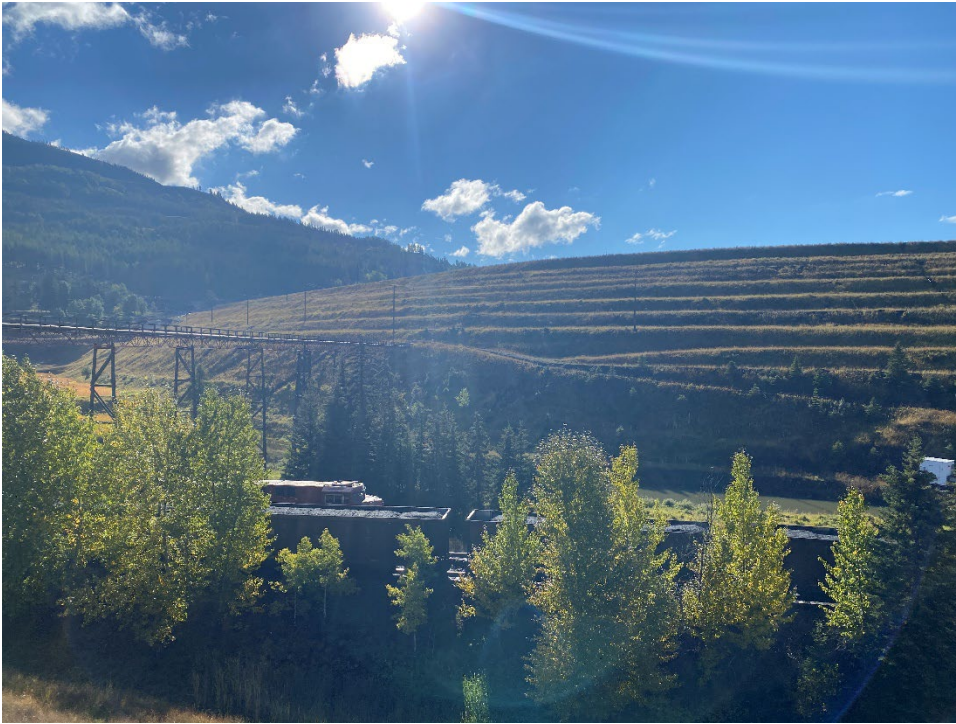
Photo ID-3 Lagoon D decant pond transfer pipeline trestle and embankment. (Looking SE, from Lagoon C crest – Taken 20 September 2022)
