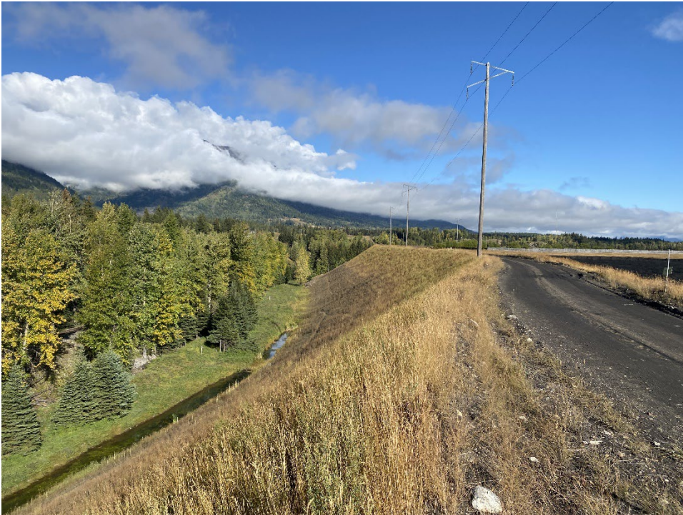
Photo IC-6 Lagoon C crest and downstream slope typical conditions. (Looking north – Taken 20 September 2022)
