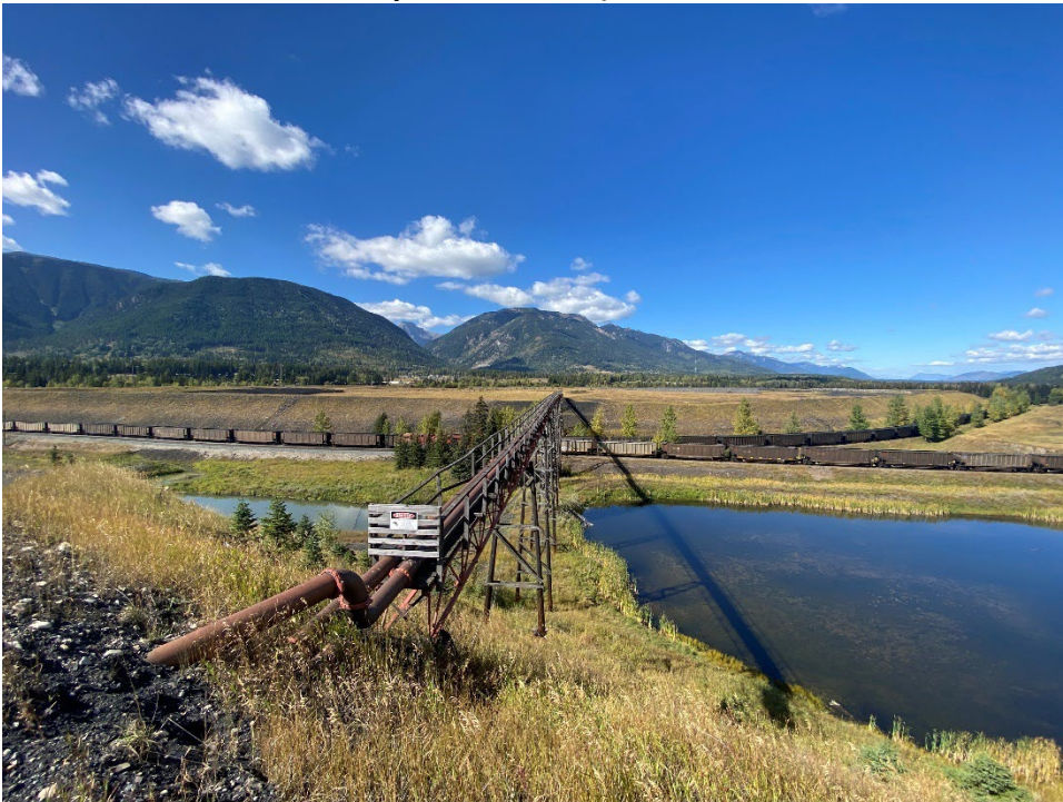
Photo ID-4 Lagoon D decant pond transfer pipeline and trestle. (Looking NW, from Lagoon D – Taken 20 September 2022)
