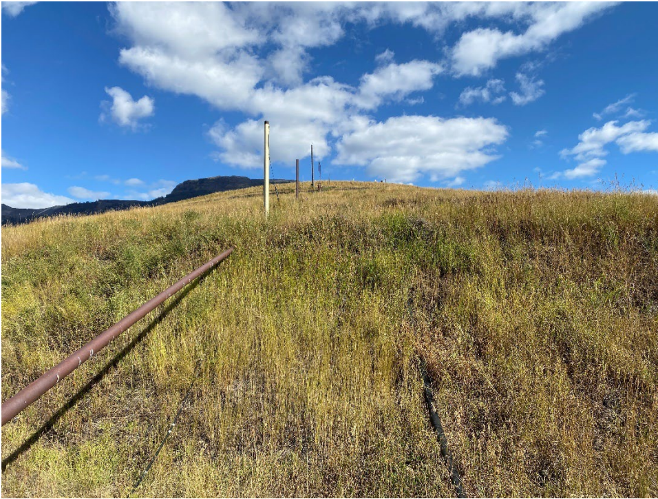
Photo ID-9 Lagoon D decant pipeline and embankment slope. (Looking east – Taken 20 September 2022)
