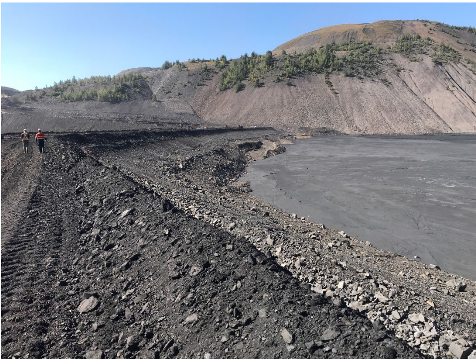
Photo IW-8 WFTF embankment tailings contact and typical upstream slope. (Looking west – Taken 21 September 2022)
