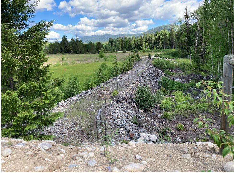
Photo 13: South TSF – Cell 3 Embankment Crest, Downstream Slope and Toe Area, Looking South from Cell 4. Jun 22, 2022
