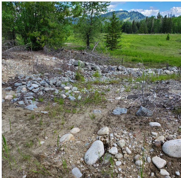
Photo 8: South TSF –Spillway from Cell 5 to Cell 4, Looking Northwest at Cell 5. Jun 22, 2022
