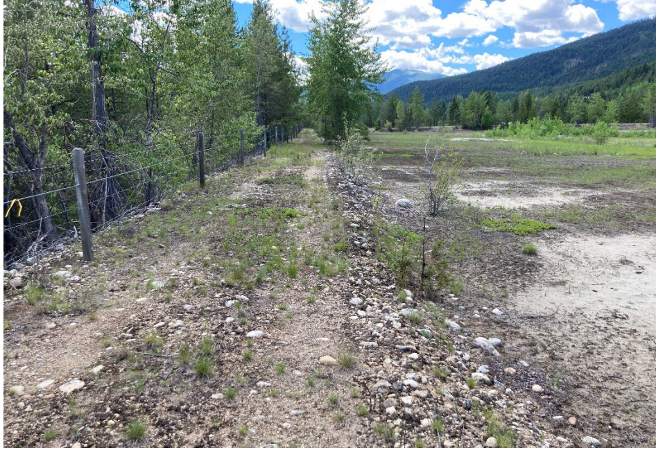
Photo 21: North TSF –Cell 6 East Embankment Crest and Upstream Tailings, Looking South. Jun 22, 2022
