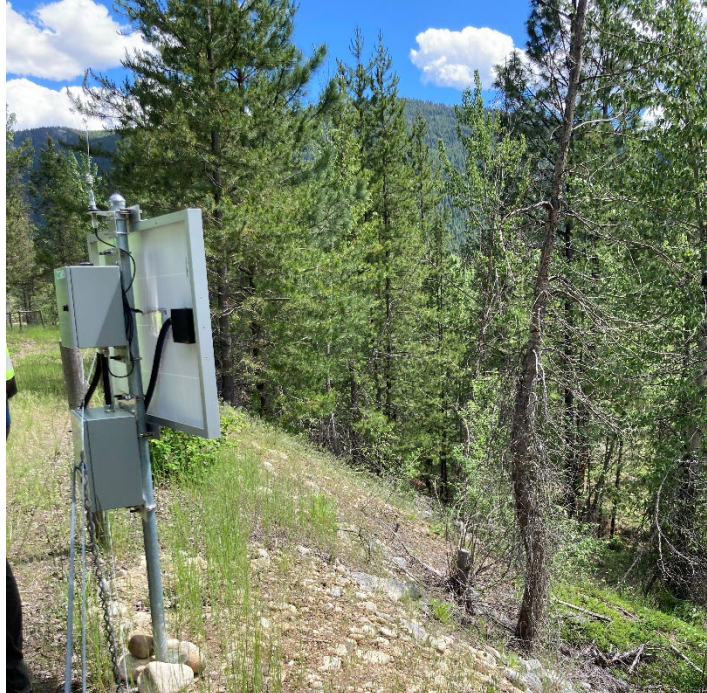
Photo 25: North TSF –Cell 7 South Embankment Downstream Slope near Signal Repeater, Looking East. Jun 22, 2022
