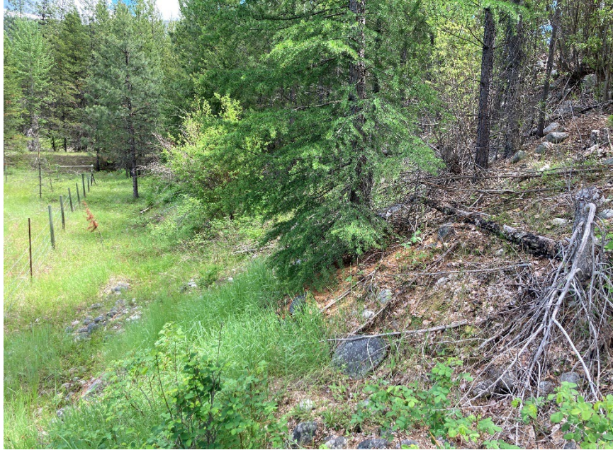
Photo 29: North TSF –Cell 7 North Embankment Downstream Slope and Toe, Looking East. August 19, 2021
