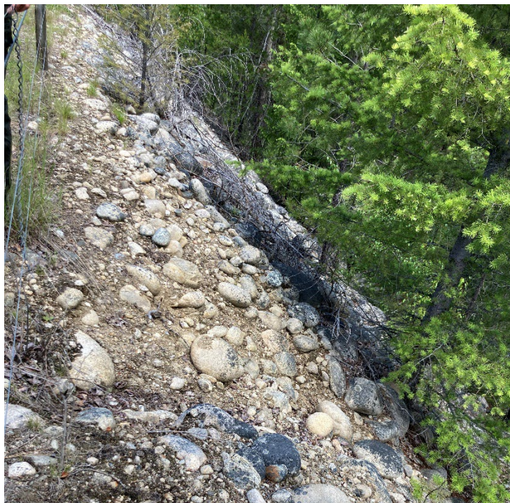
Photo 20: North TSF –Cell 6 East Embankment Downstream Slope Minor Surface Erosion, Jun 22, 2022
