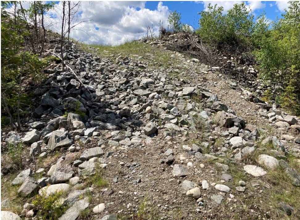
Photo 12: South TSF –View of Spillway Between Cell 3 and Cell 4, Looking South from Cell 3. Jun 22, 2022
