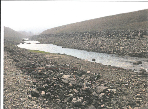
Photo 3: Looking downstream at NTP riprap (far bank) covered by gravel (approx. Sta. 0+340 to 0+450)
