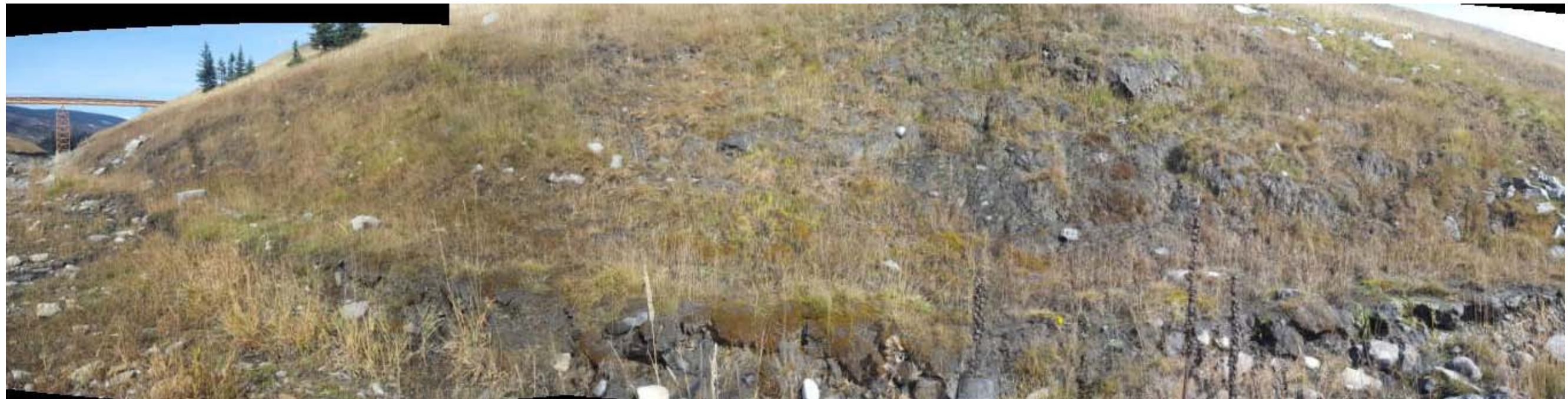
Photograph 40: STP West Dam, seepage along the downstream toe, looking northeast. 4 October 2017.
