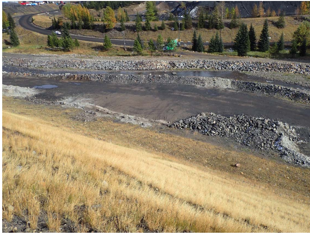
Photograph 8: NTP dam downstream slope and toe with riprap staging area, looking east. 4 October 2017.
