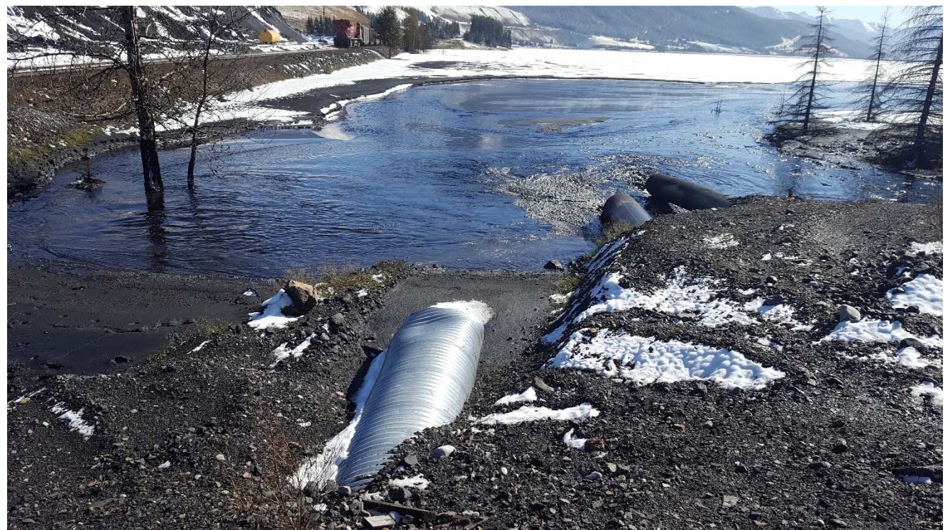
Photograph 56: STP north abutment, outlet of tailings pipe and water return pipe, looking southeast. 3 October 2017.
