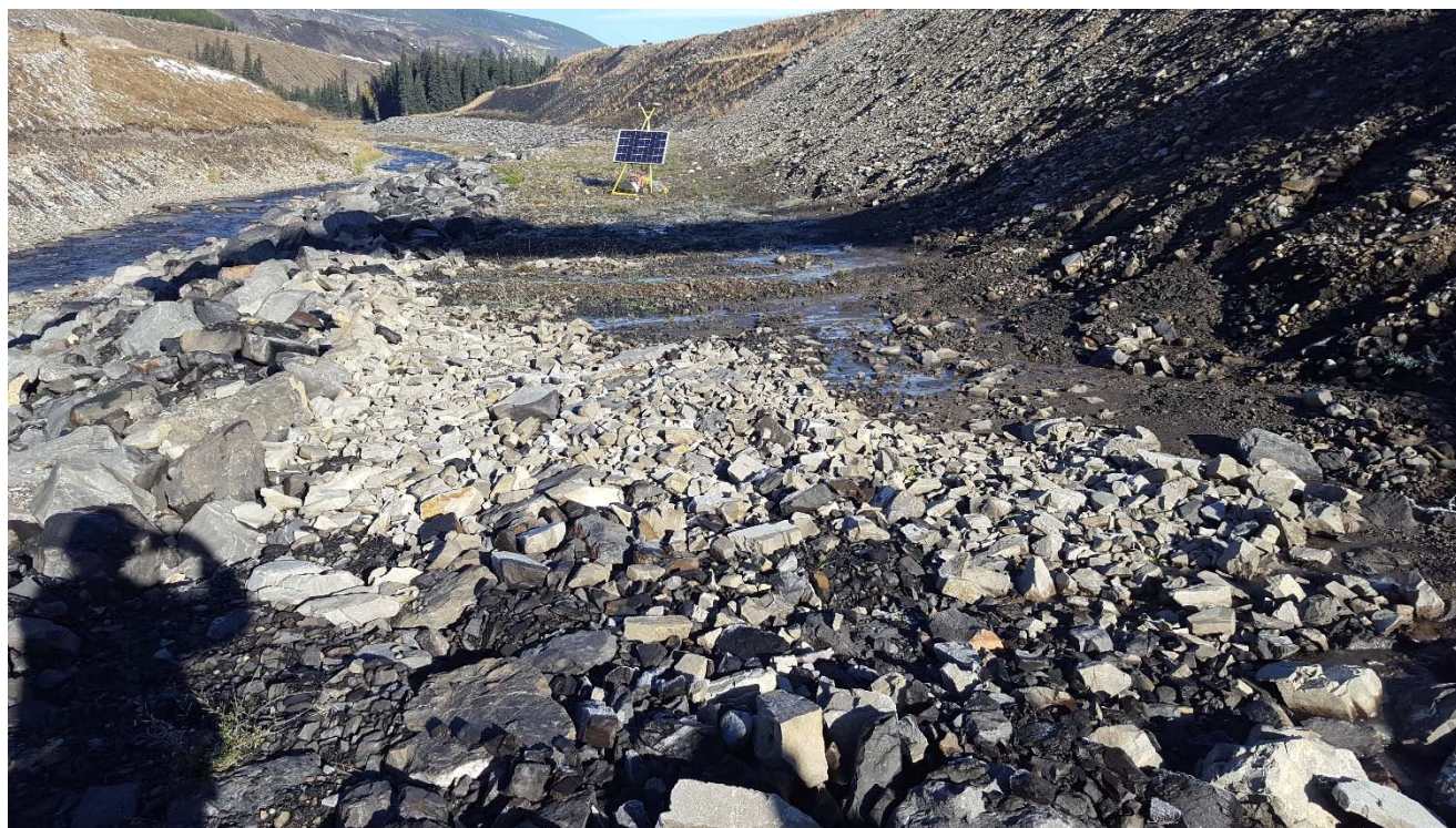
Photograph 43: STP West Dam, seepage at riprap at downstream toe, looking northwest. 4 October 2017.
