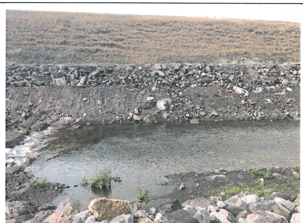
Photo 4: NTP riprap (far bank) with 2013 riprap covered by gravel on lower slope and 2016 riprap exposed on upper slope (approx. Sta. 0+500)
