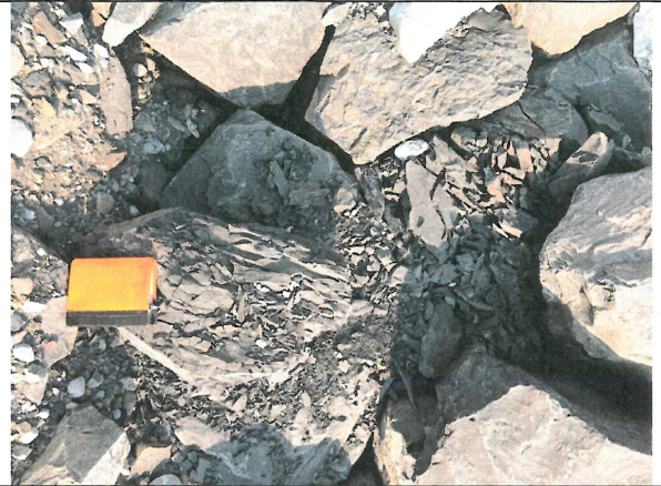
Photo 10: Riprap degradation due to weathering on a surface of a piece of riprap
