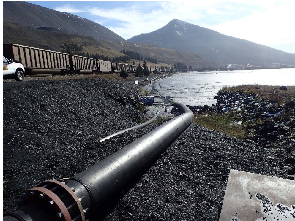
Photograph 23: STP buttress adjacent to railway line, twin culvert outlets from Blackmore Creek, and dredge pipeline to the Turnbull South Tailings Storage Facility, looking southeast. 4 October 2017.
