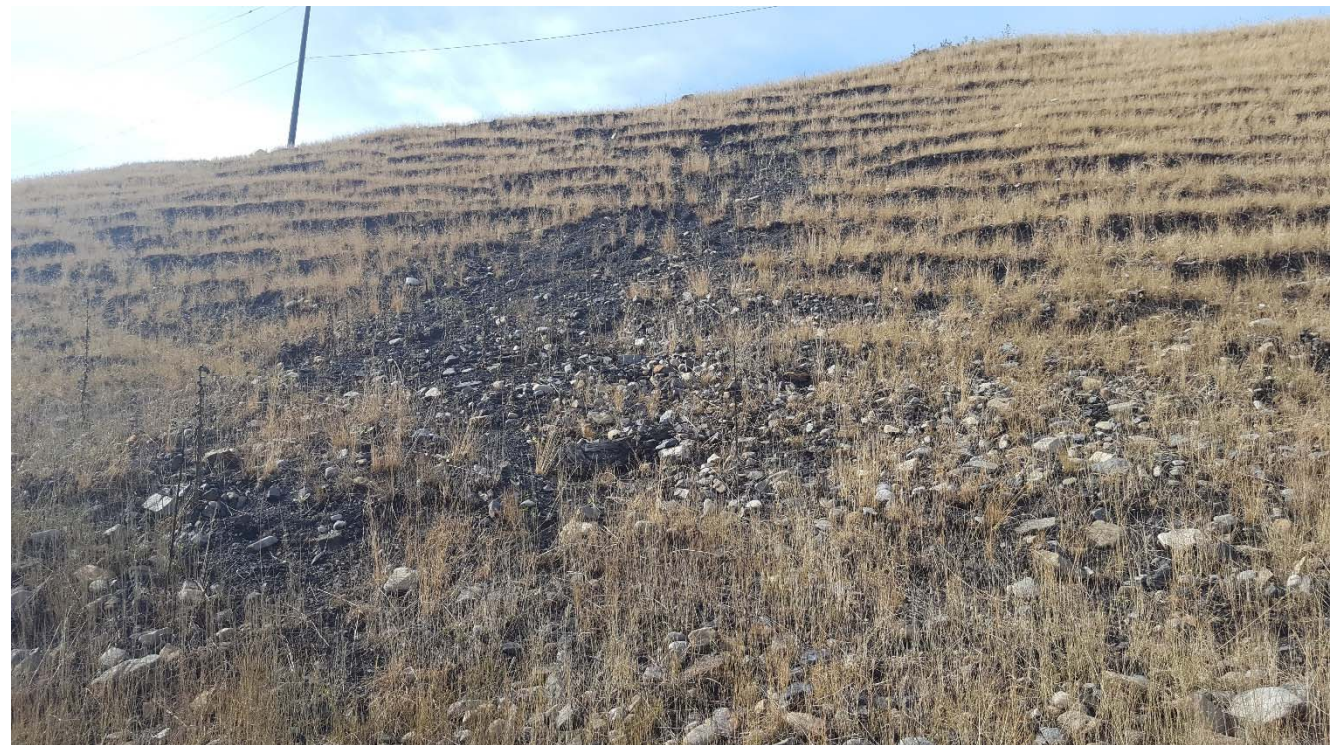
Photograph 7: NTP dam downstream slope with stepped erosion, looking northwest. 4 October 2017.
