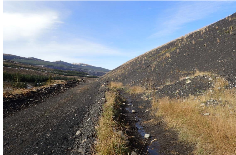
Photograph 37: STP West Dam, access road used for riprap haulage, ditch re-established along bench, looking northwest. 4 October 2017.
