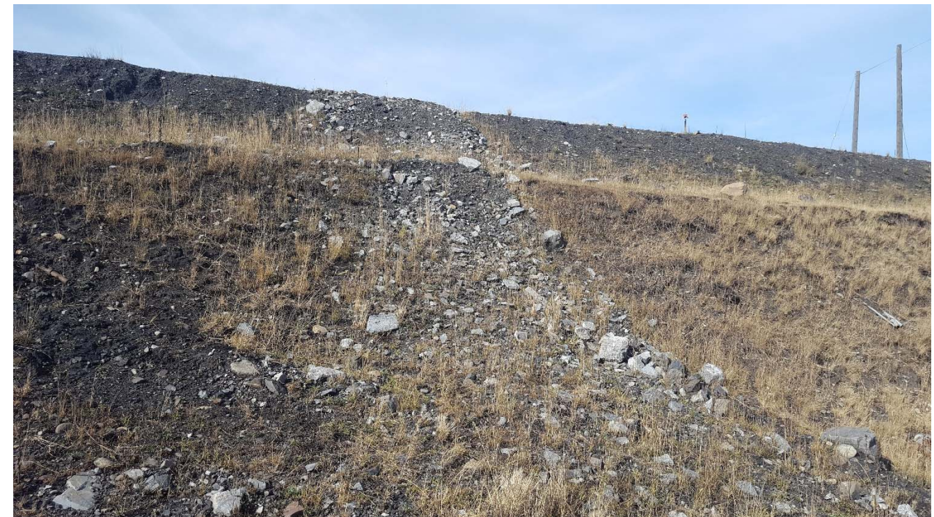
Photograph 3: NTP dam downstream slope at south abutment with filled erosion channel, looking northwest. 4 October 2017.
