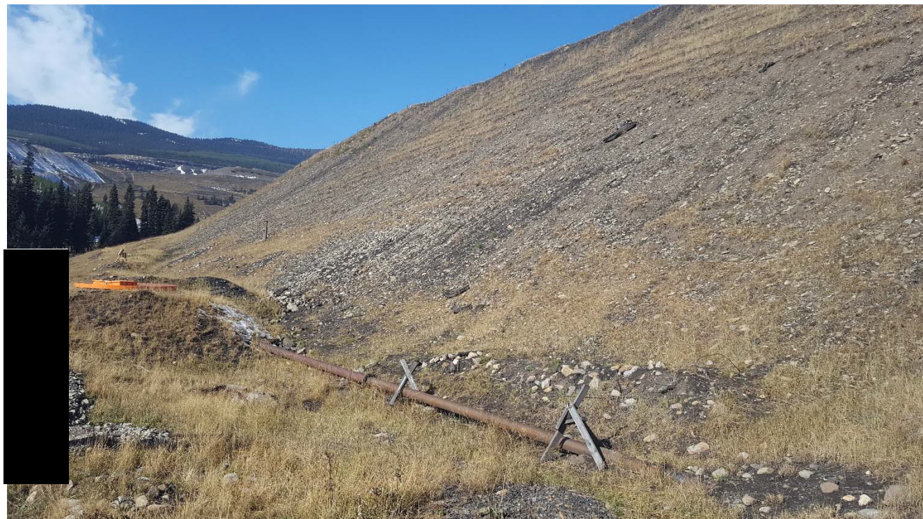
Photograph 32: STP Main Dam, downstream slope and toe at seepage return well, looking west. 4 October 2017.
