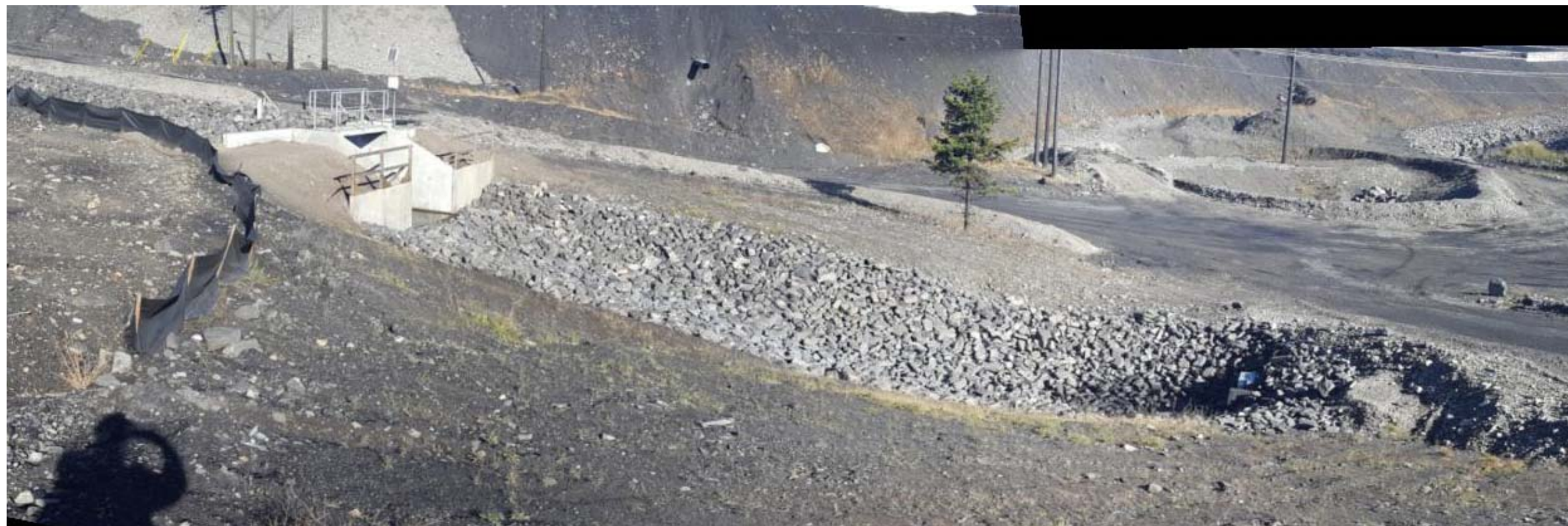
Photograph 20: Liverpool Pond outlet north of NTP, fish control structure, looking north. 5 October 2017.
