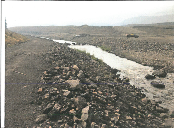
Photo 1: Looking downstream at NTP riprap (far bank) covered by gravel (approx. Sta. 0+100 to 0+200)
