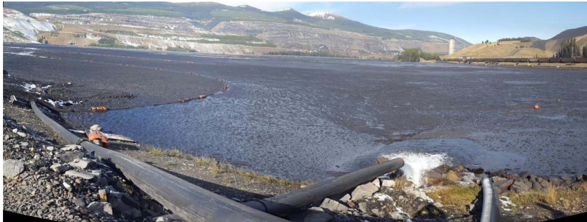
Photograph 27: STP south abutment till blanket area, makeup water lines from Kilmarnock Ponds with riprap protection on blanket, looking northwest. 4 October 2017.
