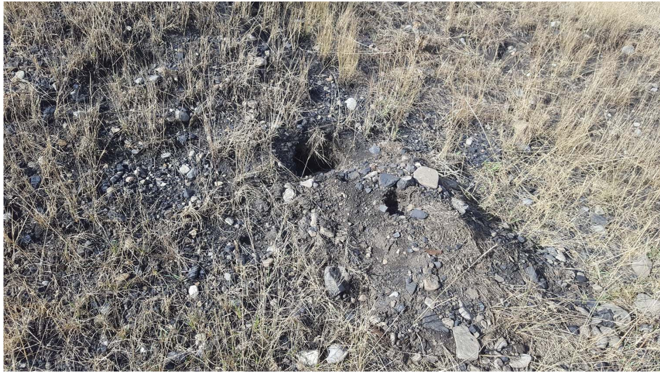
Photograph 4: NTP downstream toe, animal burrows near south abutment, looking northwest. 4 October 2017.
