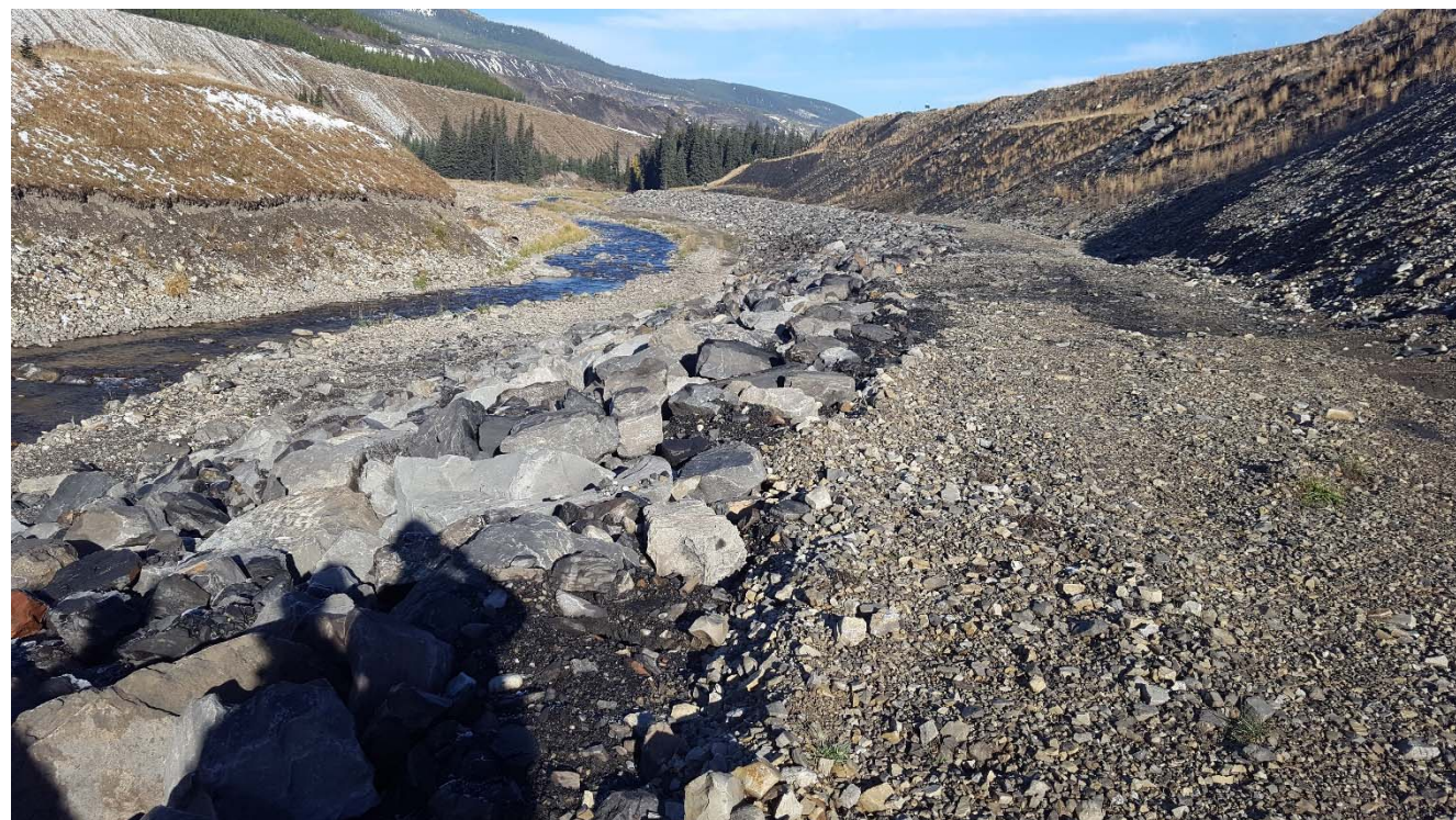
Photograph 47: STP West Dam, riprap placed at toe of dam for erosion protection from Fording River, looking northwest. 4 October 2017.
