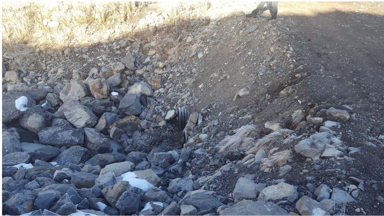
Photograph 49: STP West Dam, twin culverts beneath access road at toe, looking east. 4 October 2017.
