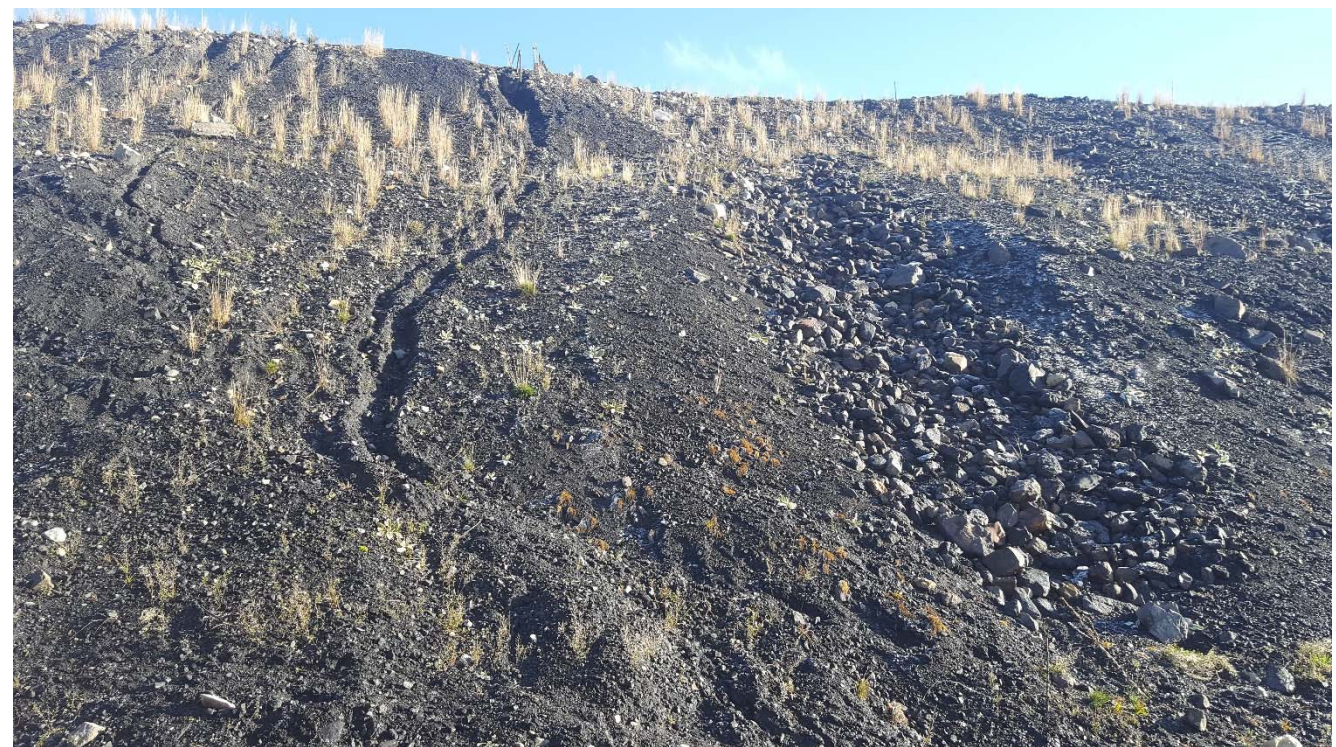
Photograph 48: STP West Dam, erosion gully and infilled depression, looking northeast. 4 October 2017.
