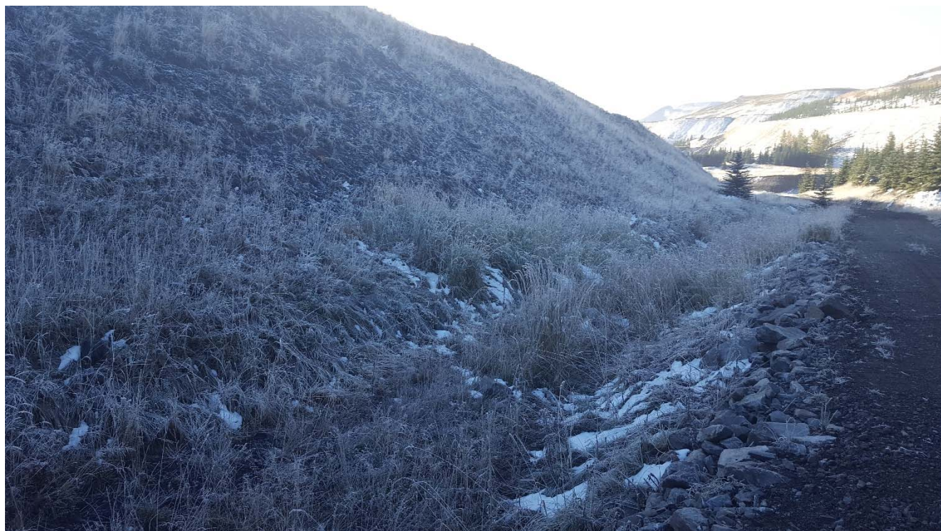
Photograph 51: STP West Dam downstream slope with vegetation and ditch at downstream toe, looking south. 4 October 2017.
