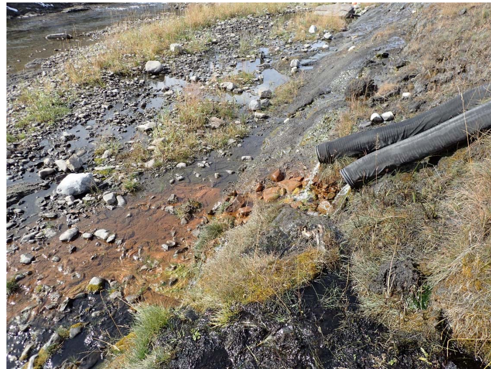
Photograph 39: STP West Dam, major seepage point at the downstream slope toe (Stn. 1+000). Seepage collection pipes monitor flow. Note discolouration. The flow rate at the time of inspection was approximately 3 L/sec from both pipes. Looking northwest. 4 October 2017.
