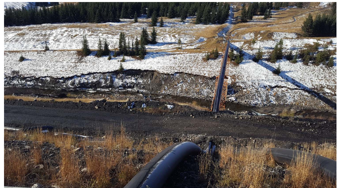
Photograph 44: STP unused dredge line to 2P-3P Tailings Storage Area on pipe bridge, looking southwest. 4 October 2017.
