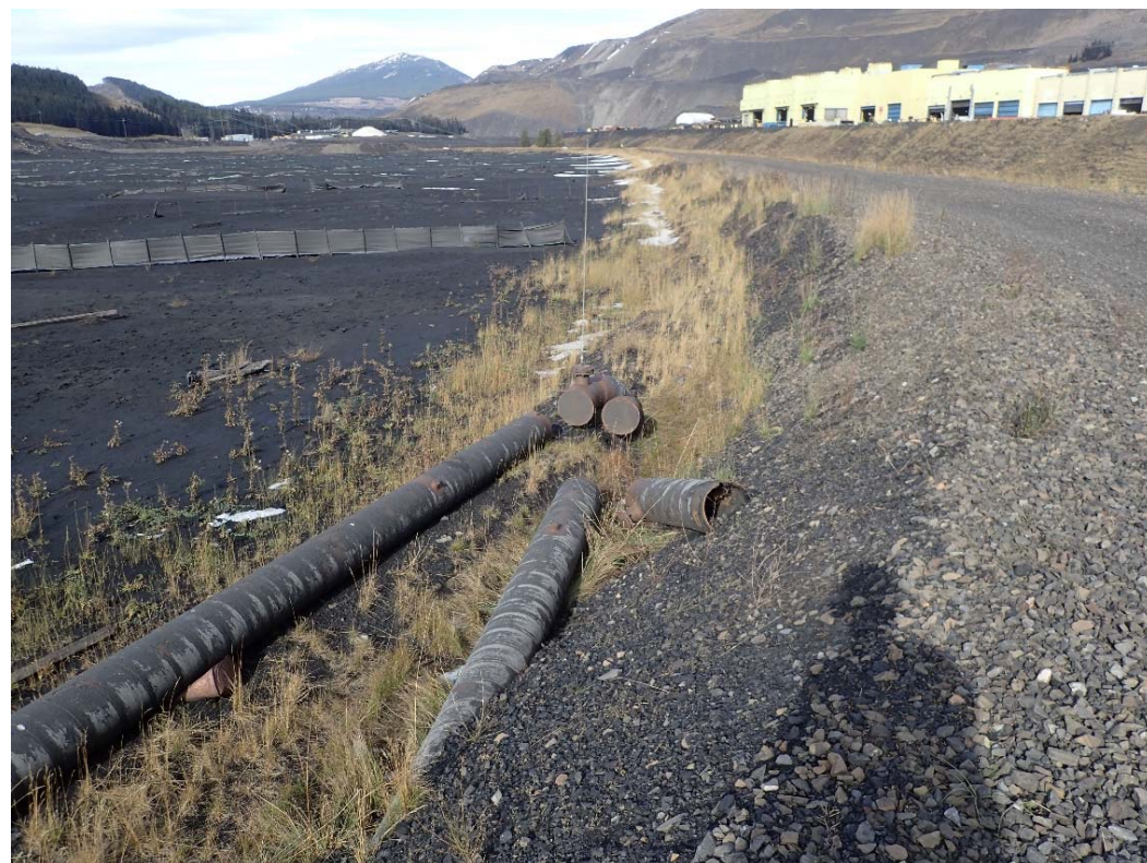
Photograph 13 : NTP unused dual reclaim pipes on upstream slope and crossing under crest, looking north. 4 October 2017.
