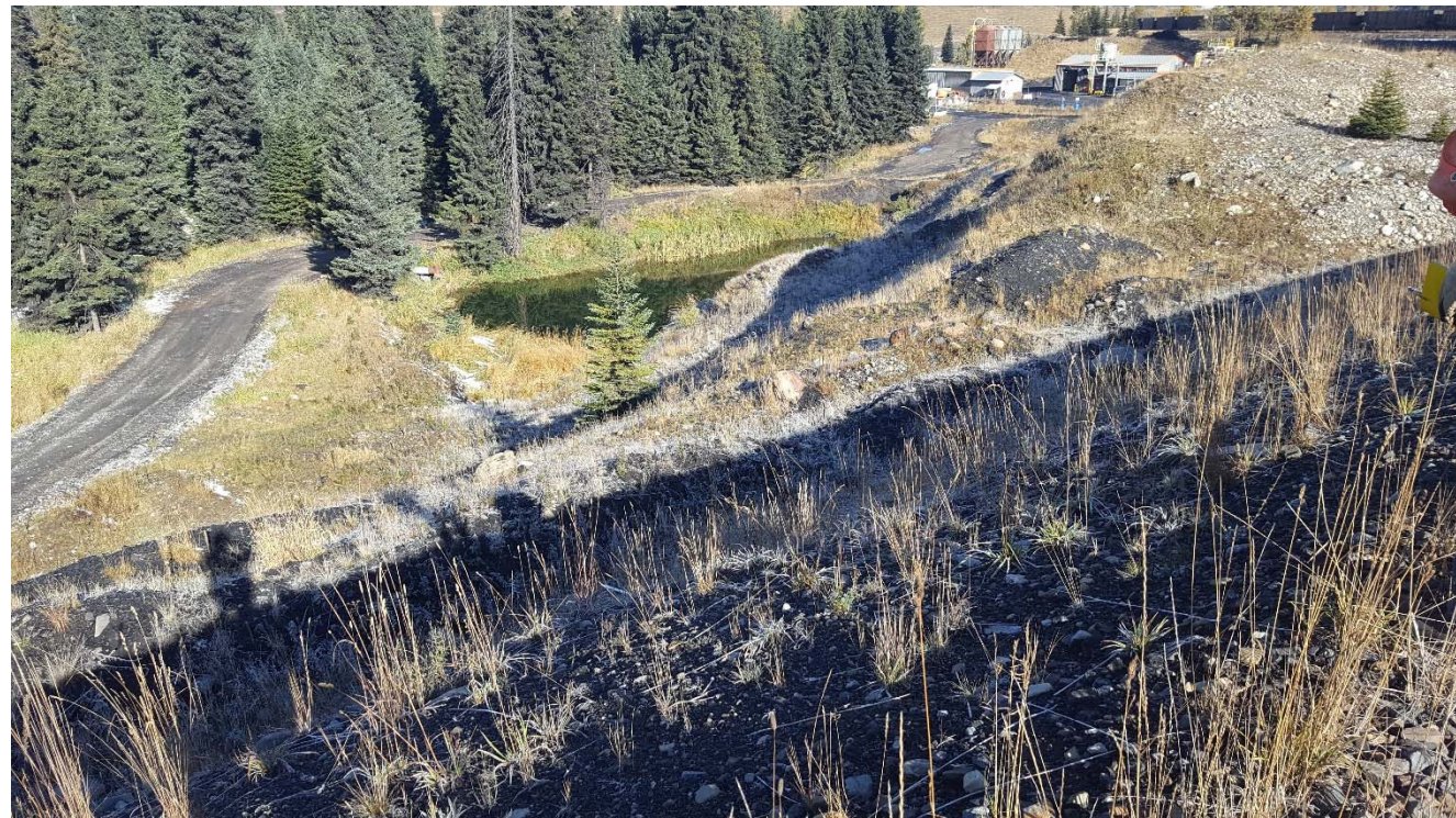
Photograph 53: STP West Dam, pond at downstream toe near Stn.-0+050, looking northwest. 4 October 2017.
