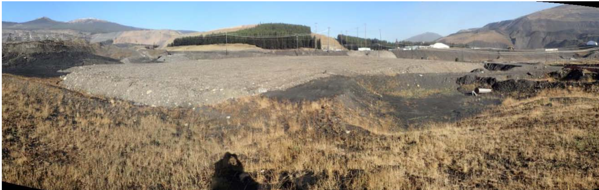
Photograph 17: NTP near north abutment, dozed till material and unused steel tailings pipe, looking north. 5 October 2017.
