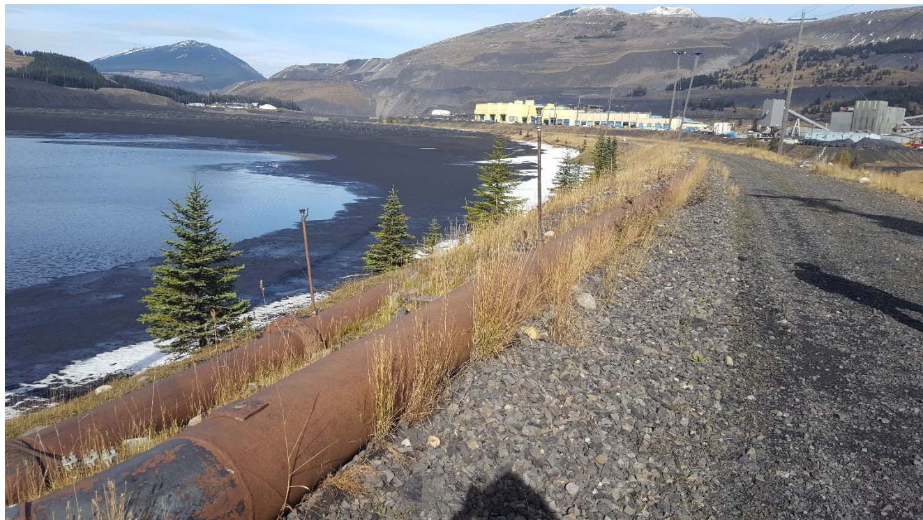
Photograph 6: NTP dam upstream slope with small trees and vegetation growing, and unused reclaim pipes, looking northeast. 4 October 2017.
