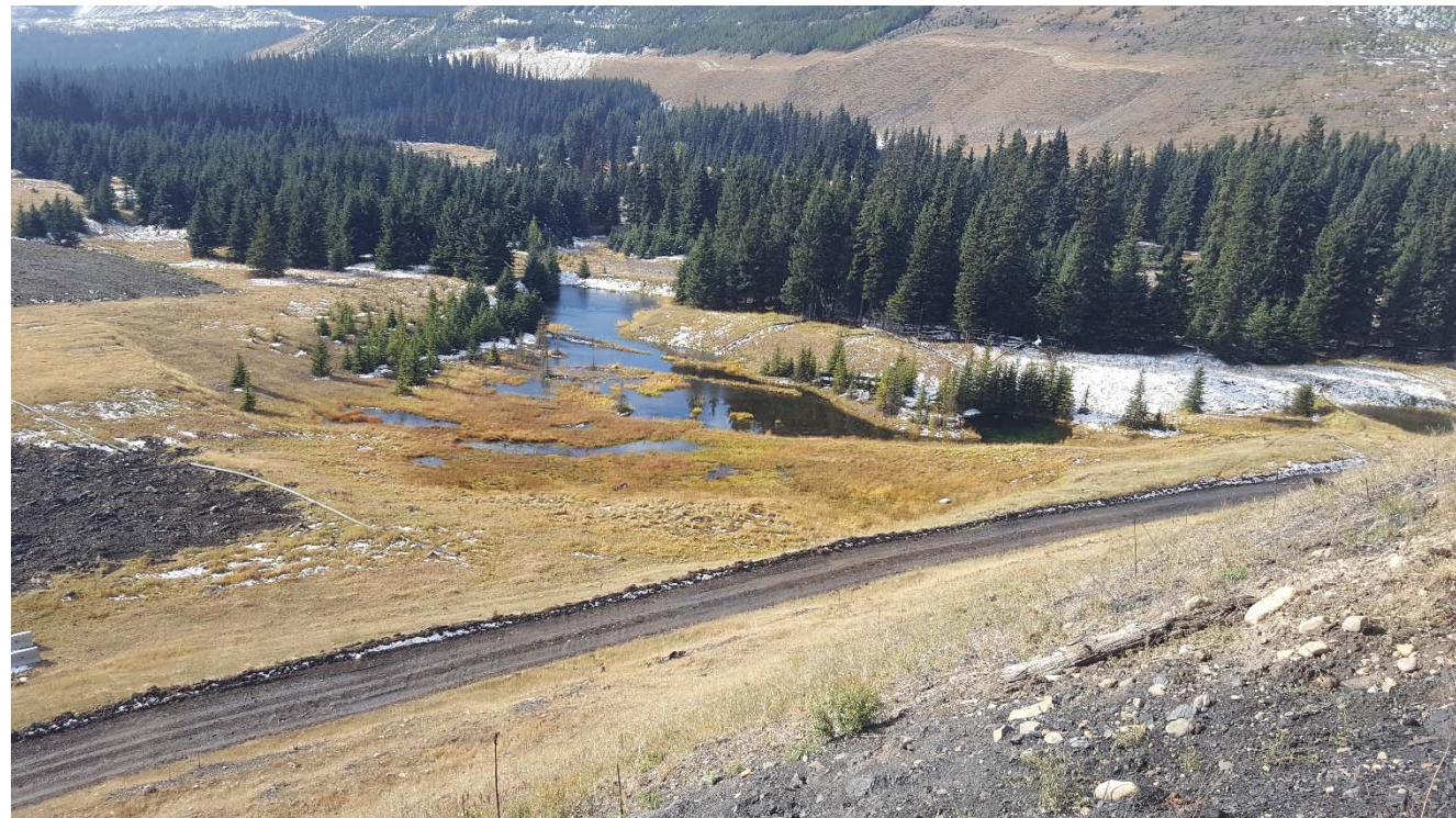
Photograph 34: STP Main Dam, persistent ponding downstream of toe in old river channel, looking southwest. 4 October 2017.
