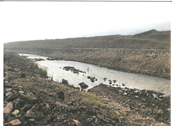
Photo 2: Looking downstream at NTP riprap (far bank) covered by gravel (approx. Sta. 0+200 to 0+320)
