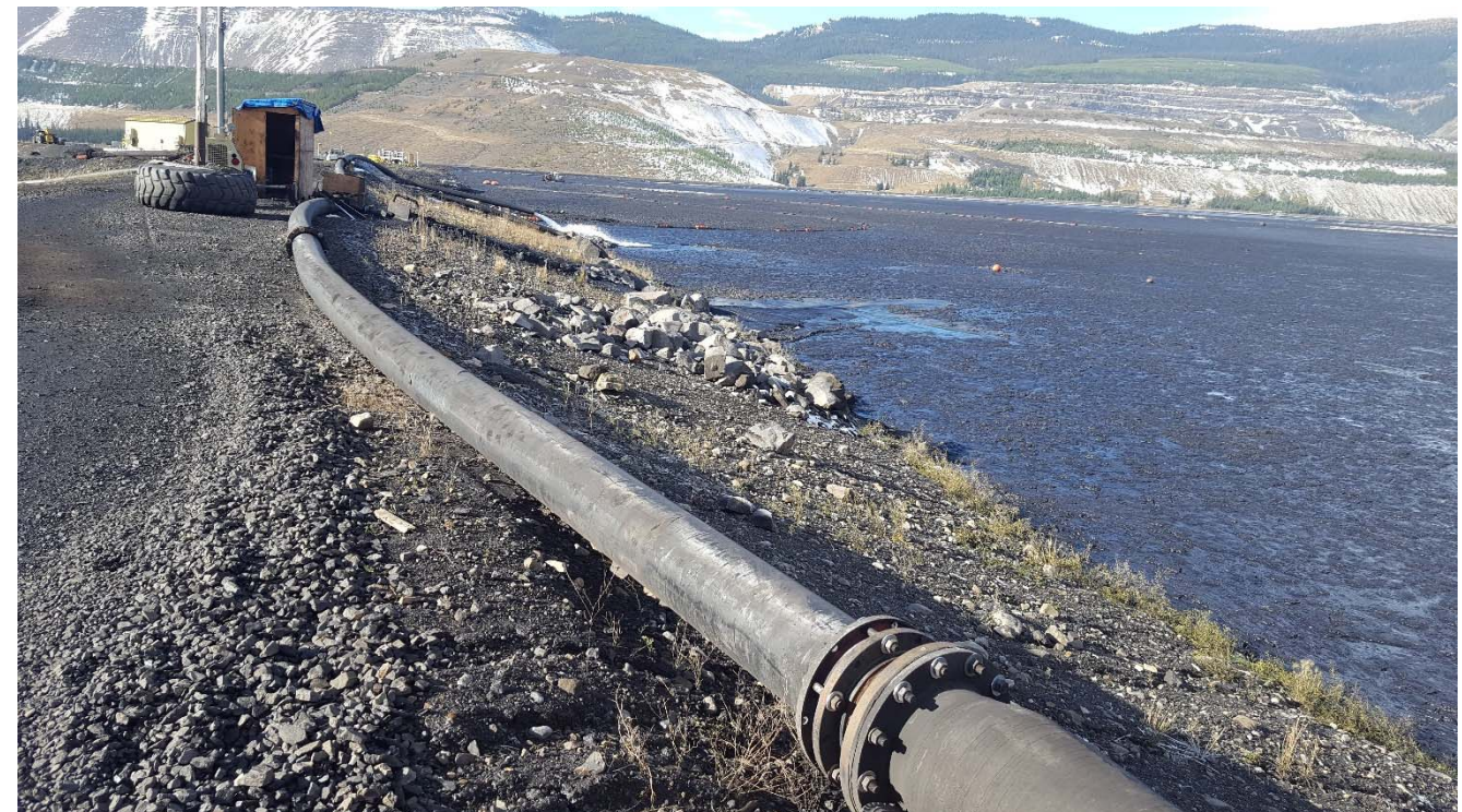
Photograph 26: STP south abutment till blanket area and upstream slope, looking southwest. 4 October 2017.
