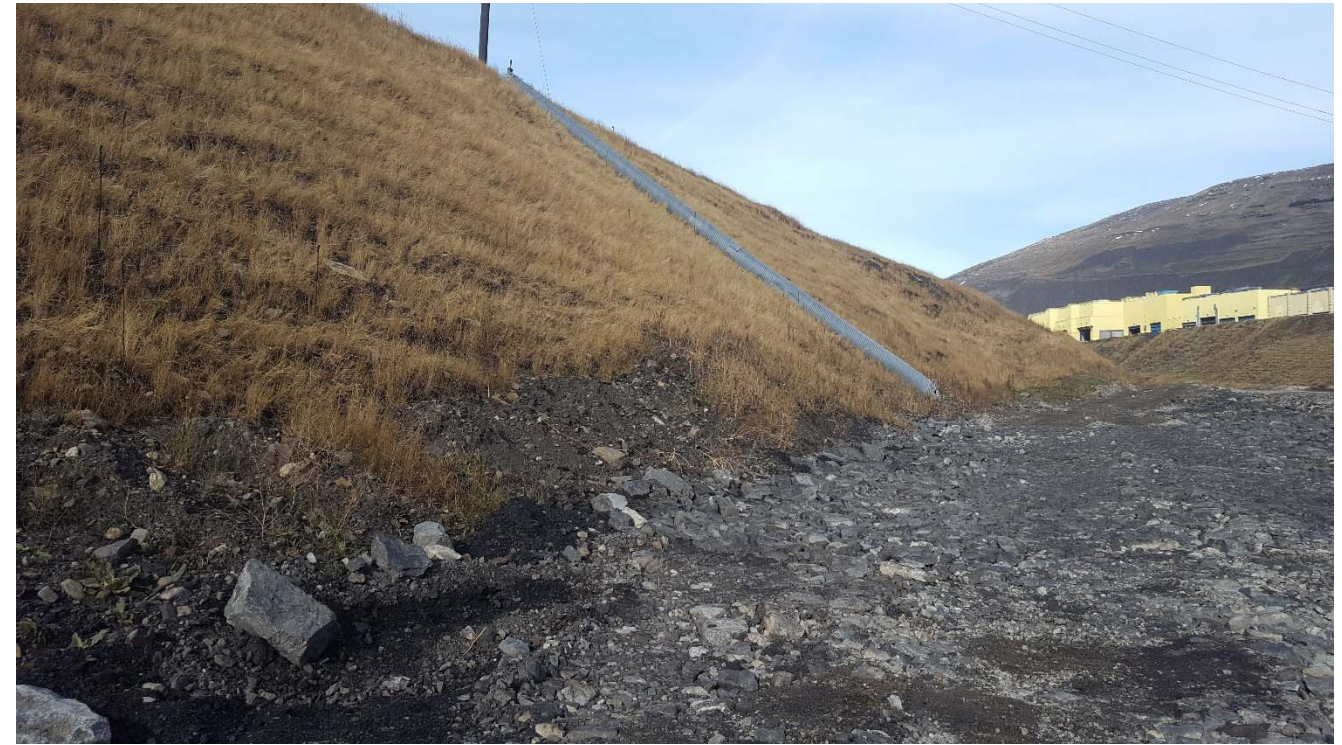
Photograph 9: NTP dam downstream slope with unused pipe along surface of slope, looking northeast. 4 October 2017.
