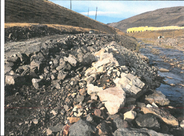
Photo 7: Looking upstream at NTP downstream tie-in of raised riprap (approx. Sta. 0+900 to 1+070)
