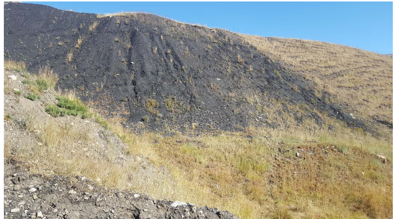
Photograph 35: STP corner of West and Main dams, looking northeast. Note vegetation not taking root in CCFR. 4 October 2017.
