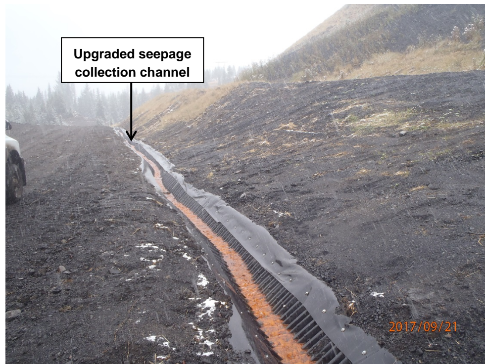
Photograph 15: Site C – upgraded seepage trench at toe of Site C refuse spoil, looking southwest. 21 September 2017.
