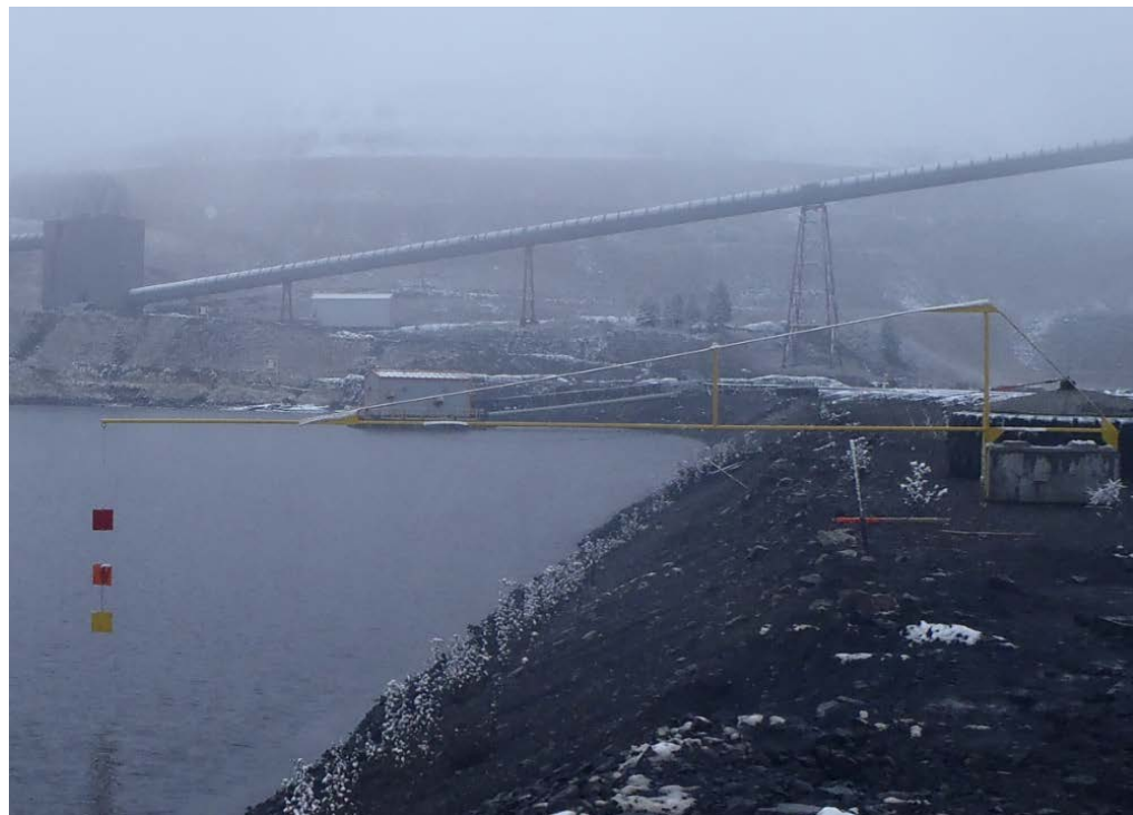
Photograph 4: Main Dam – overview of barge, east abutment, pond level indicator, and natural ground north of GHO Tailings Pond, looking north. 21 September 2017.
