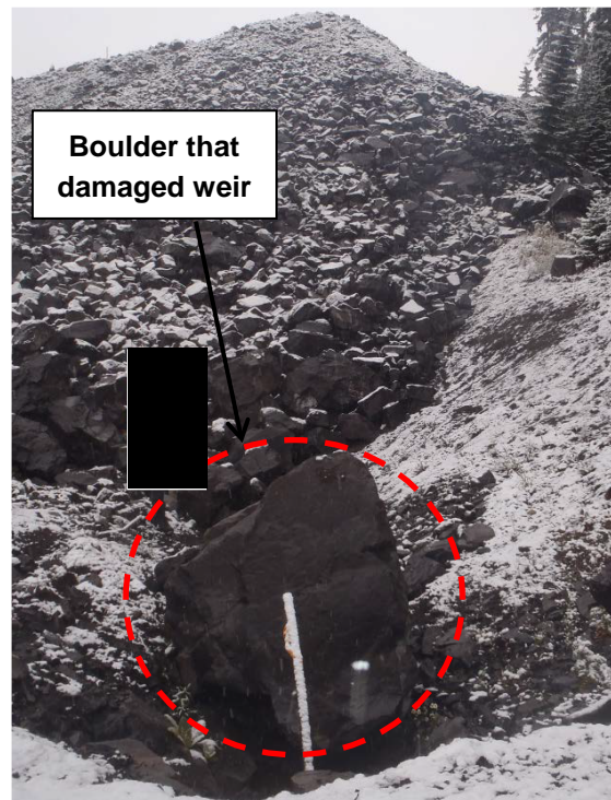
Photograph 24: West Dam – view drainage channel along downstream slope at south abutment, looking east. 21 September 2017.
