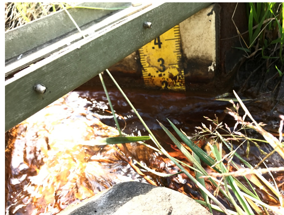
Photograph 16: Site C – weir at toe of Site C refuse spoil prior to trench upgrade, looking west. 30 July 2017.
