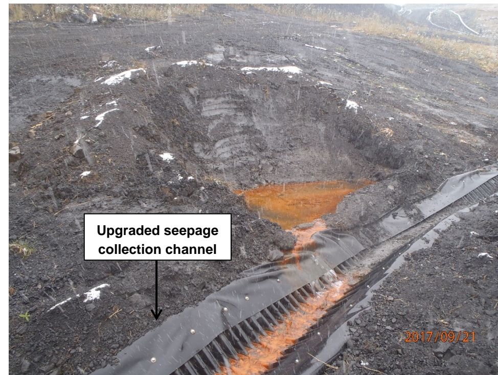
Photograph 14: Site C – view of upgraded seepage collection channel. Seepage water is red-brown. Looking northwest. 21 September 2017.
