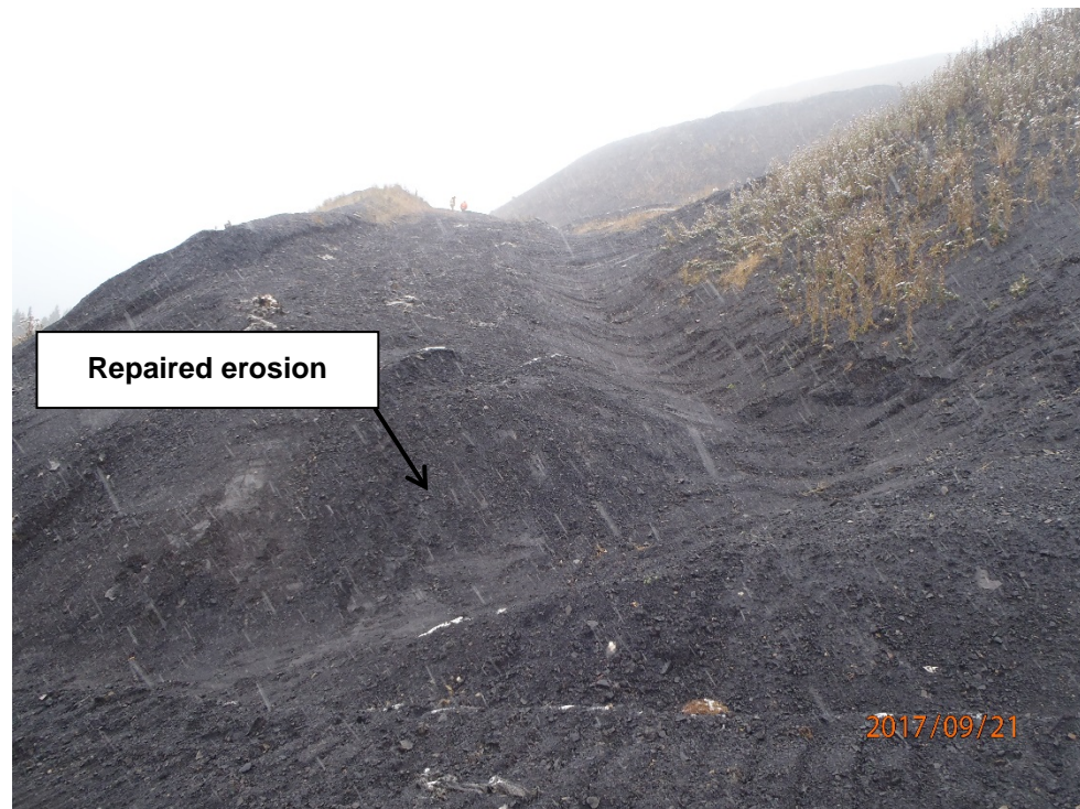
Photograph 13: Site C – repaired stormwater runoff erosion on west side of refuse dump, looking northwest. 21 September 2017.
