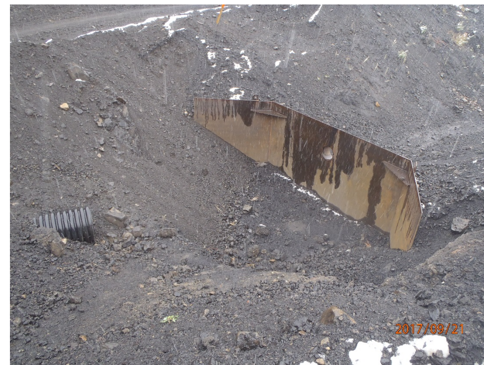
Photograph 12: Site C – view of new weir under construction on west side of refuse dump, looking north. 21 September 2017.
