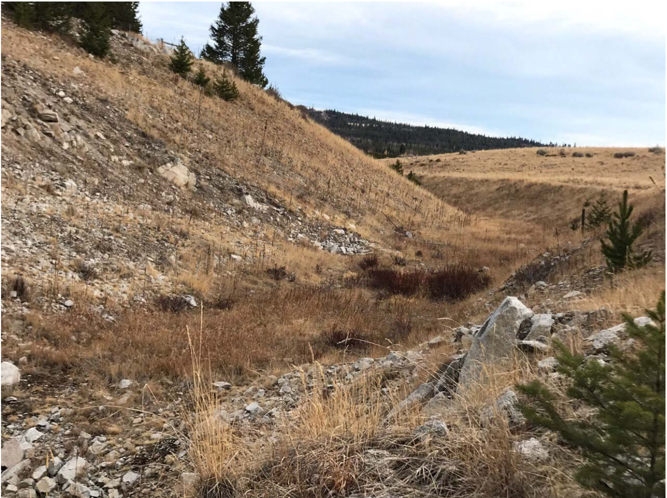
Photo II-A- 18 Spillway curve at transition point from till to bedrock view upstream (TRJ-2017-03)
