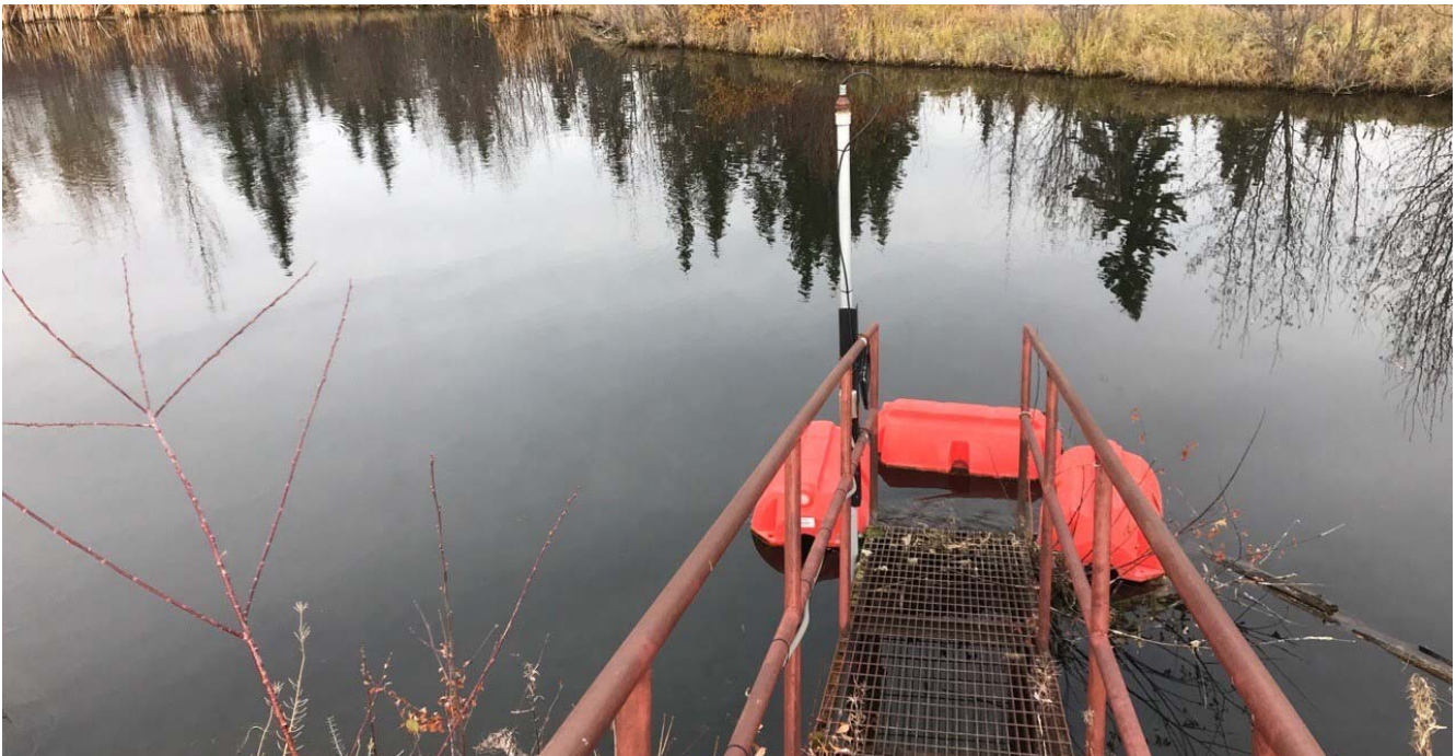
Photo II-C- 10 Debris boom and outfall intake. Obstruction from plant debris present (TRJ-2017-21)
