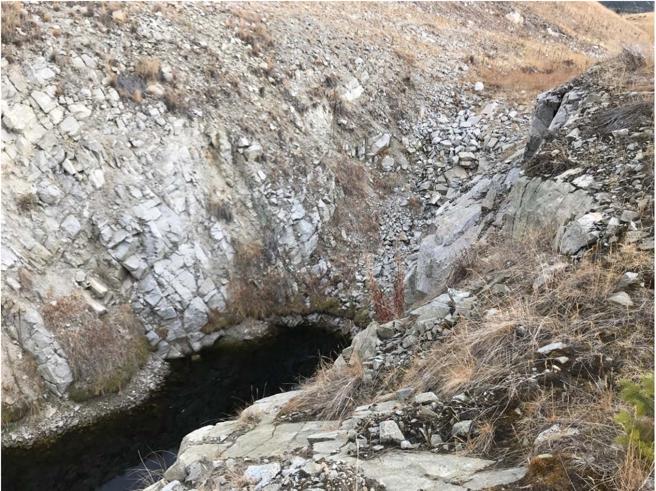
Photo II-A- 19 Spillway channel transition to bedrock with pooled water at low point, minor water level decrease from 2016 DSI inspection (TRJ-2017-03)
