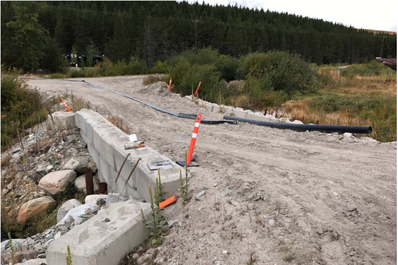
Photo II-B-22 S5: access road between central pond (right of photo) and pumping cell (left of photo). (HGH-2017-36)
