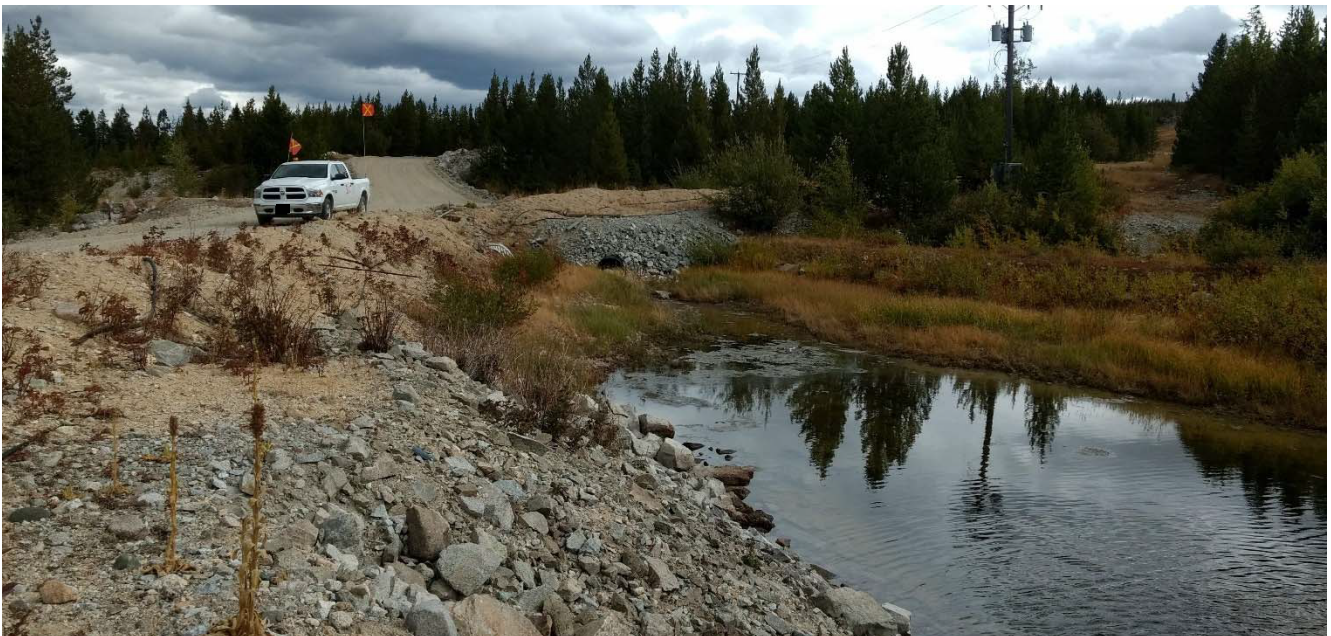
Photo II-B-10 S8: upstream slope, right abutment and spillway intake to S1 pond. (HGH-2017-17)
