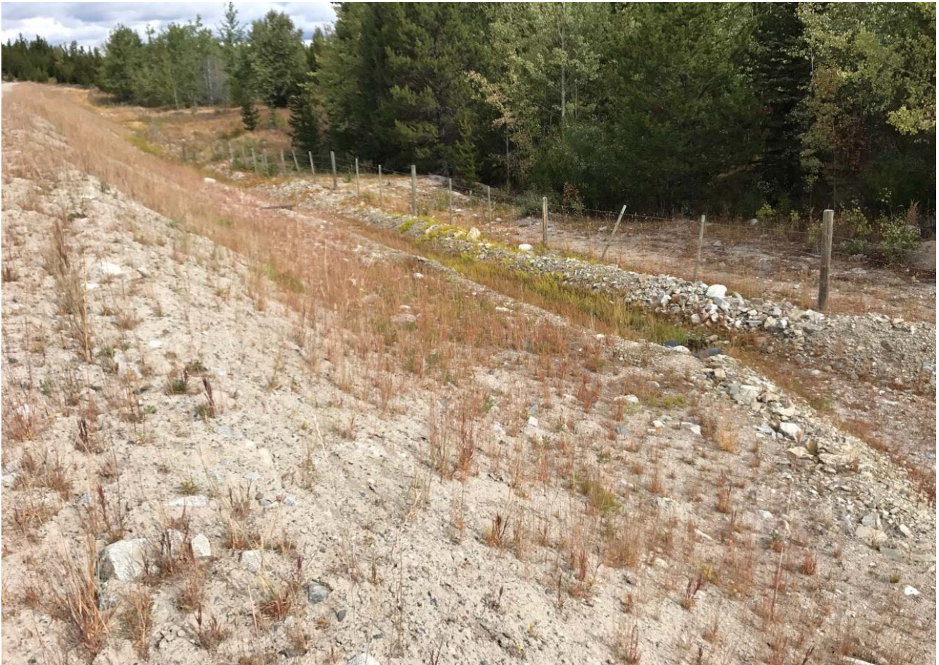
Photo II-B-27 S5: downstream slope and spillway pipes outlet at toe of dam. (HGH-2017-39)
