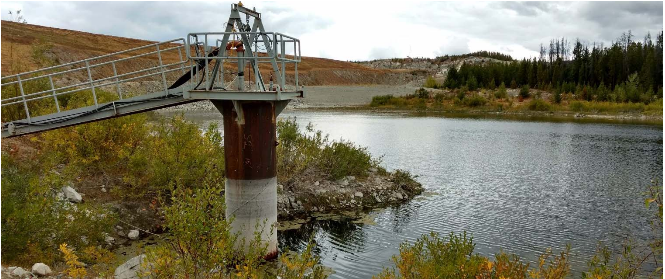
Photo II-B-6 S2: outlet pump to Seepage Recovery Pond S8. North Dam downstream slope in background. (HGH-2017-16)
