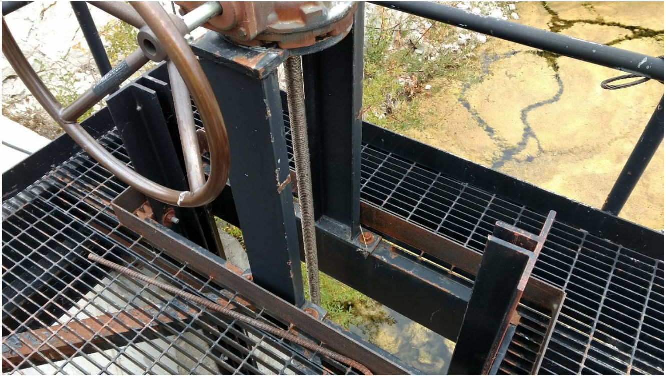
Photo II-A- 7 Spillway flow control gate (HGH-2017-03)
