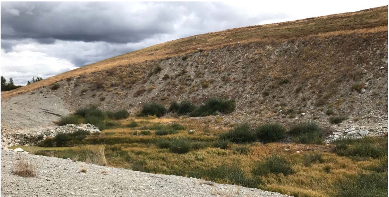
Photo II-A-15 Steepened section of downstream slope (HGH-2017-08)
