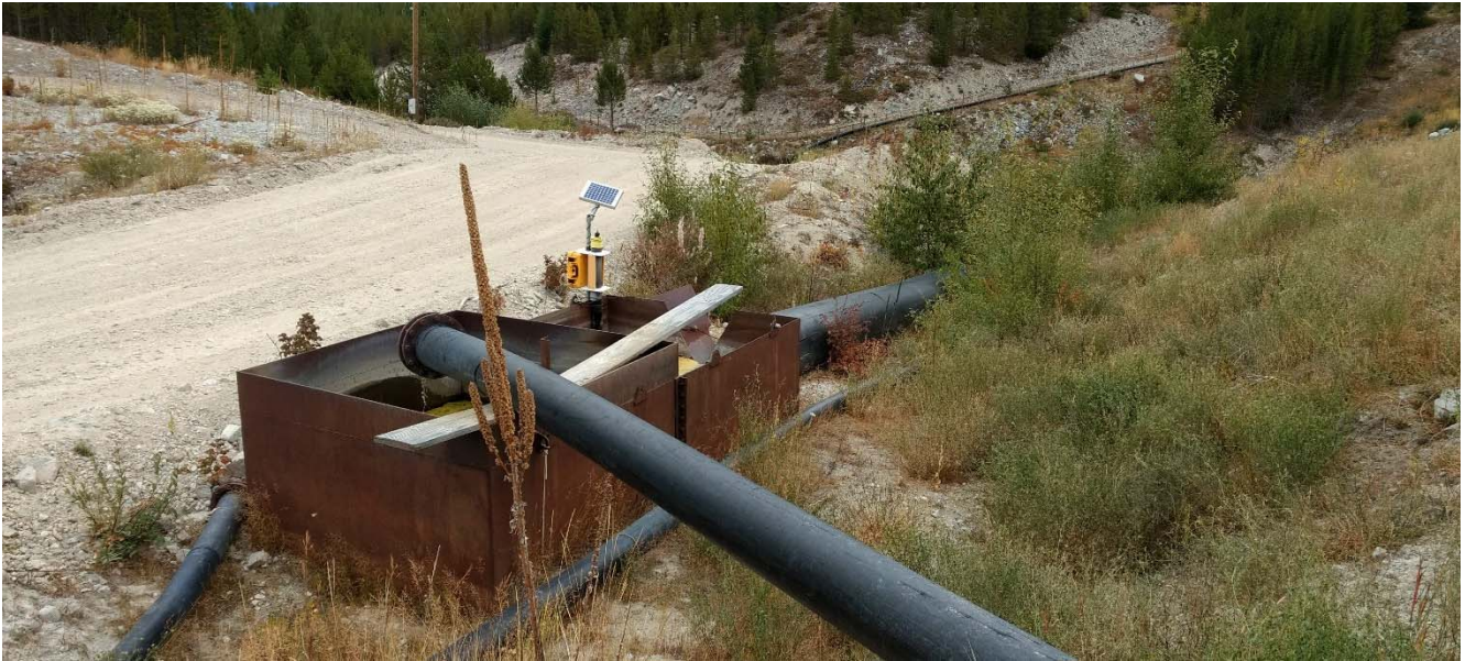
Photo II-B-12 S1: Highmont spillway diversion pipe to S1 pond. (HGH-2017-19)
