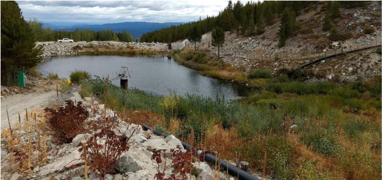
Photo II-B-14 S1: overview of pond and upstream slope of dam. System components from left to right: outlet pump to Highmont tailings pond, inflow channel from Highmont spillway diversion, inflow channel from toe drain, inflow pipe from S5 pond. (HGH-2017-23)
