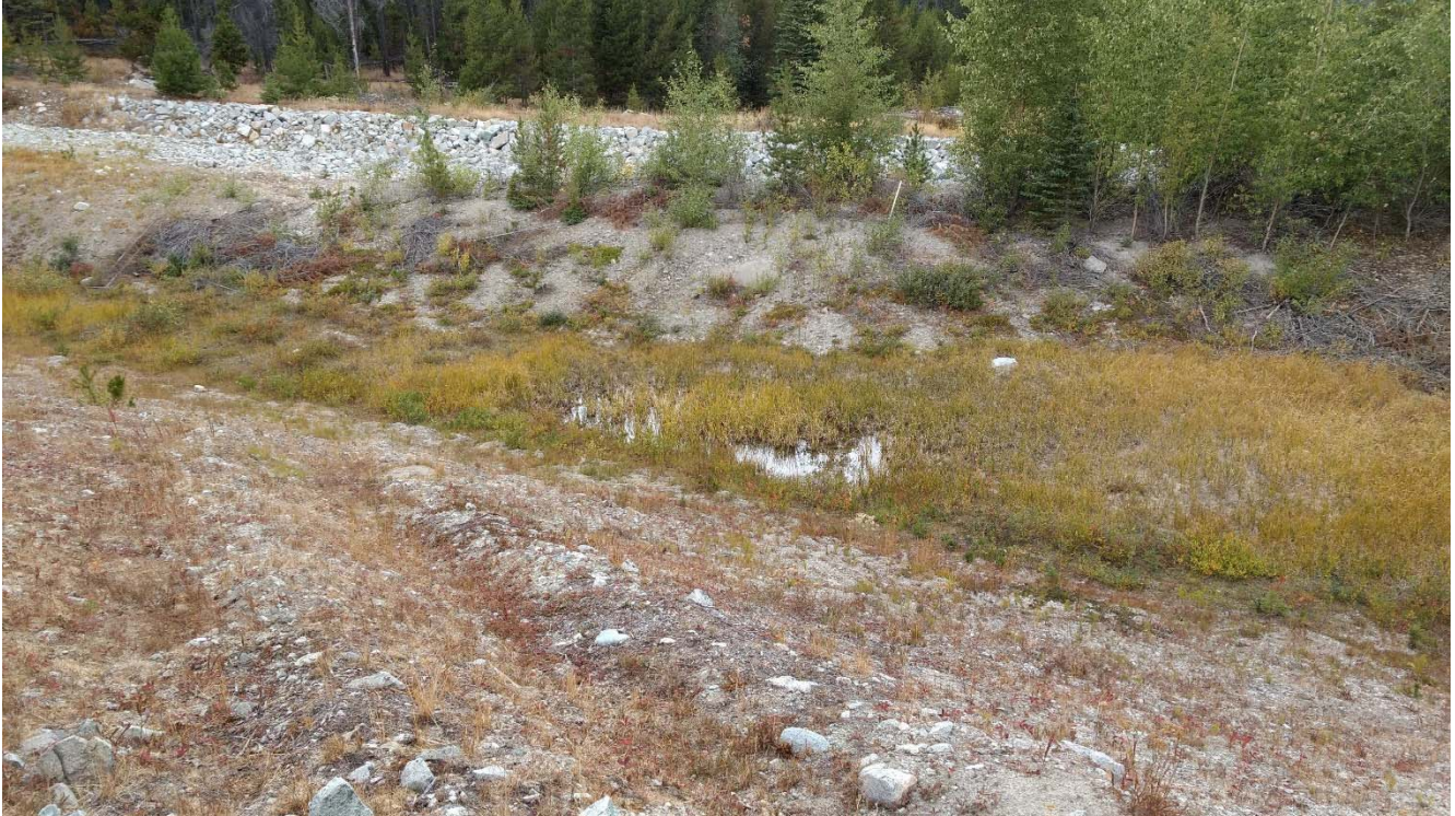
Photo II-B-4 S2: ponded water at downstream toe, similar in size to the pond noted during the 2015 and 2016 DSI. (HGH-2017-14)
