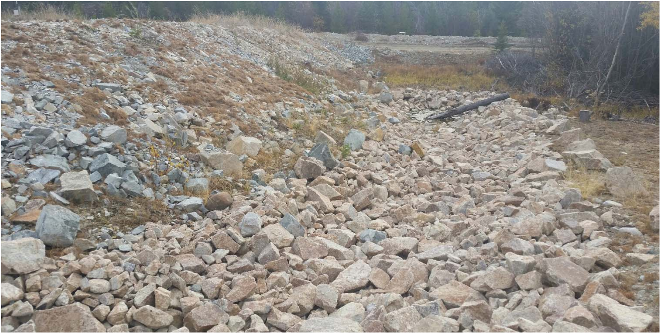
Photo II-C-8 Spillway view downstream from channel bend, no signs of erosion or deterioration, log obstruction present in lower section (BTH-2017-25)
