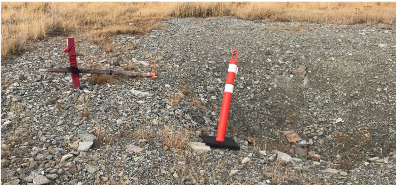
Photo II-A-9 Sinkhole on tailings beach and it's instrumentation (BTH-2017-04)
