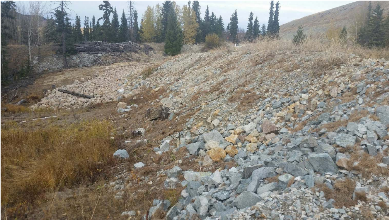
Photo II-C-10 Downstream slope of dam, view towards right abutment and spillway, no signs of erosion or deterioration (BTH-2017-28)
