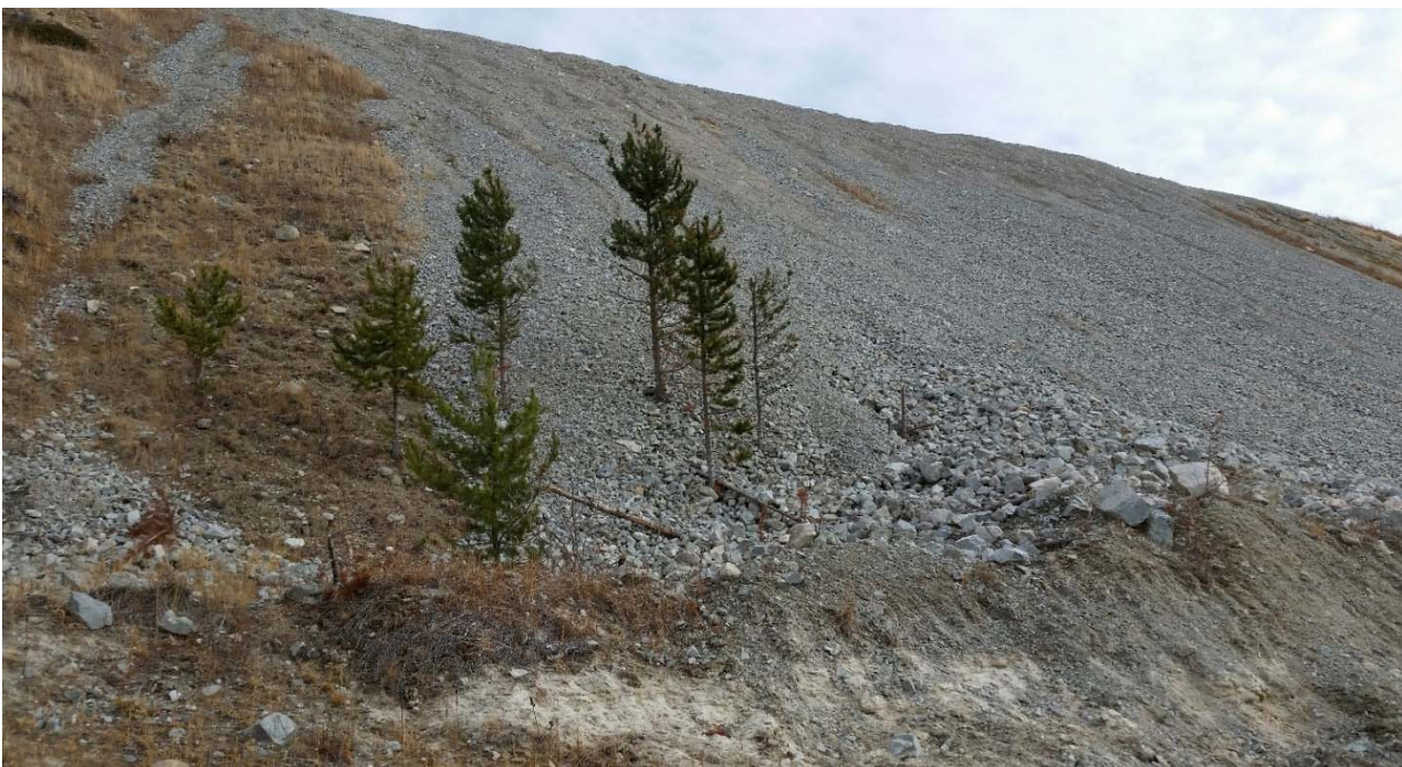
Photo II-A-3 Downstream slope of dam, historic repair of slope scar, no new signs of erosion or scouring. View towards left abutment (BTH-2017-02)
