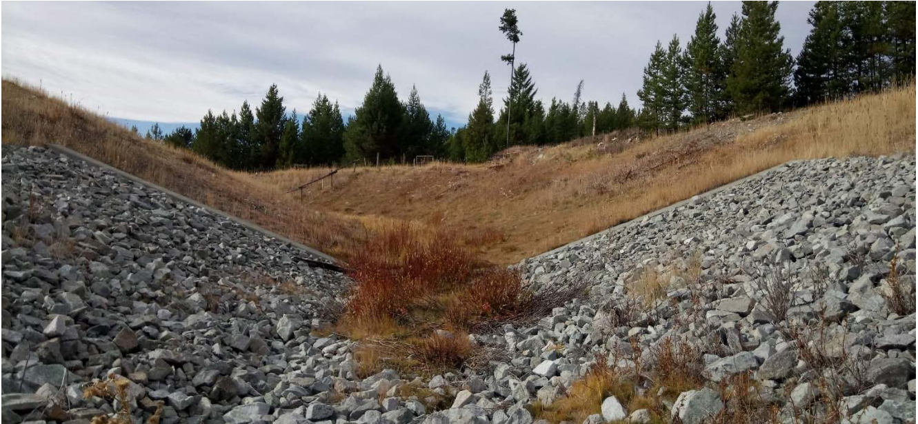
Photo II-B-14 Spillway transition point, view upstream. Trapezoidal channel in good condition with no signs of erosion. Minor vegetation at the invert, should continue to be monitored to ensure it does not reduce spillway capacity (BTH-2017-16)
