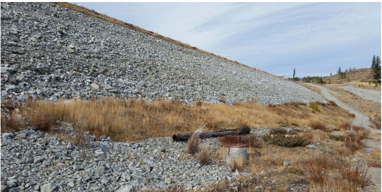
Photo II-B-7 Toe drain, no visible damage, view towards left abutment. Lower portion of dam from toe drain to the service road, transitions from rockfill armour to till, no signs of erosion or deterioration observed (BTH-2017-12)
