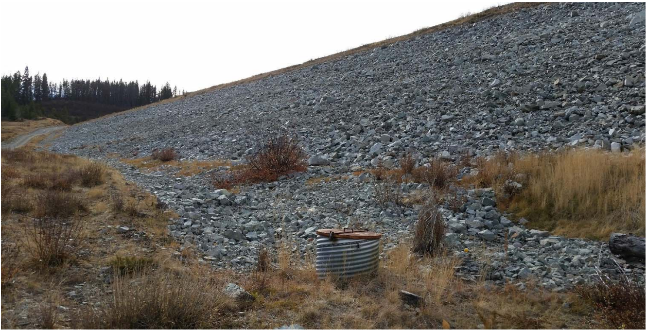
Photo II-B-8 Toe drain, no visible damage, view towards right abutment at the till/rockfill armour transition point (BTH-2017-12)
