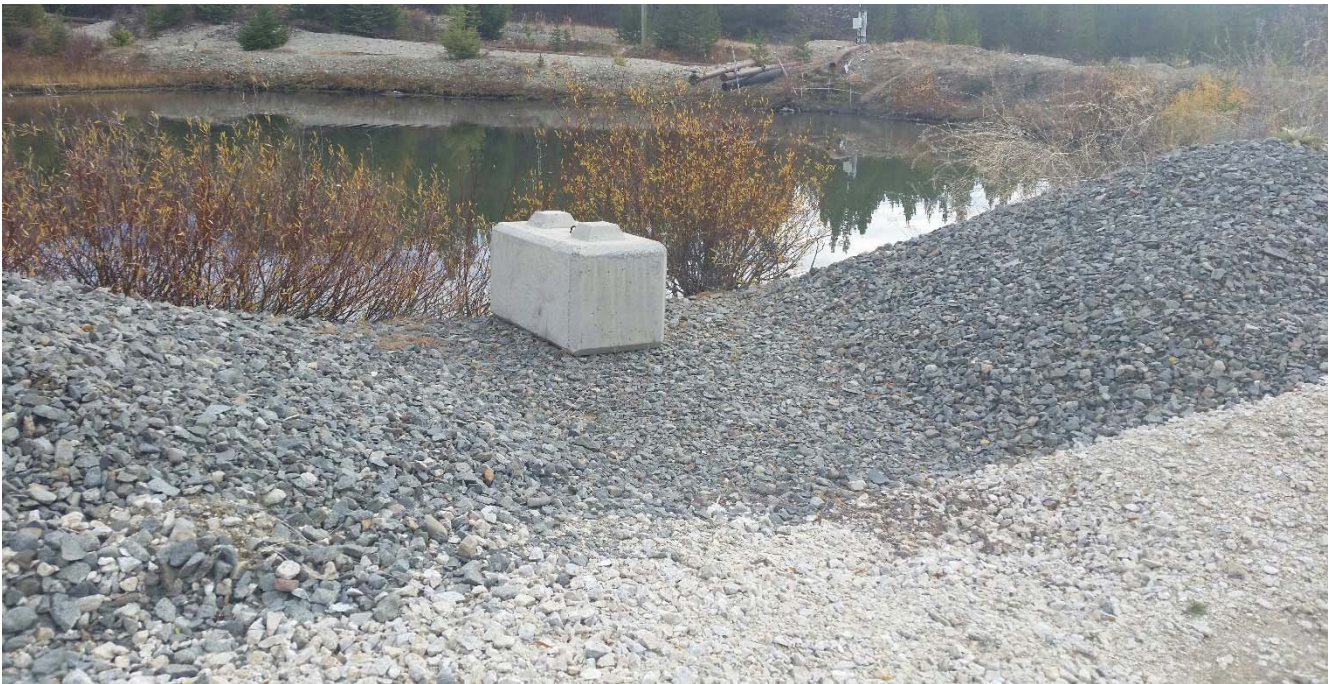
Photo II-C-5 Spillway inlet, trapezoidal channel in good condition, no signs of erosion in fine riprap (BTH-2017-24)
