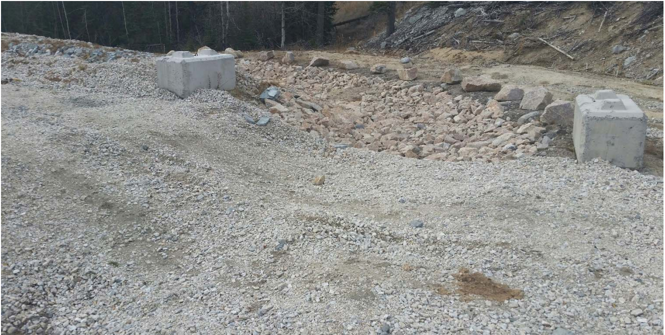
Photo II-C-6 Spillway view downstream from crest of dam, transition to large riprap as channel steepens (BTH-2017-24)
