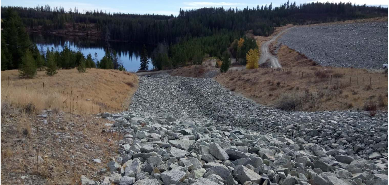
Photo II-B-16 Spillway channel looking downstream towards Bose Lake. Flow discharges past the road via two culverts (~1.2m and 0.5m in size) no signs of deterioration to spillway channel observed (BTH-2017-18)
