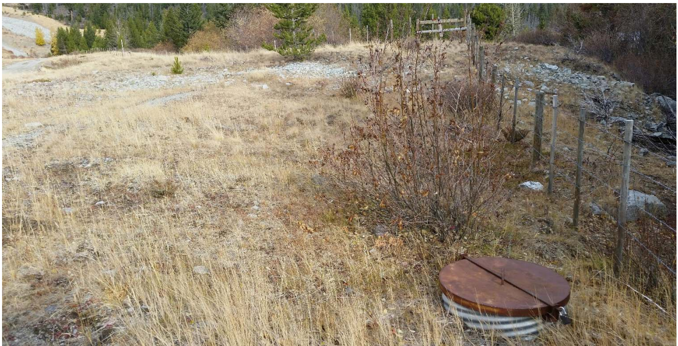
Photo II-B-5 Toe drain located along fence line, no visible damage, view downstream (BTH-2017-10)
