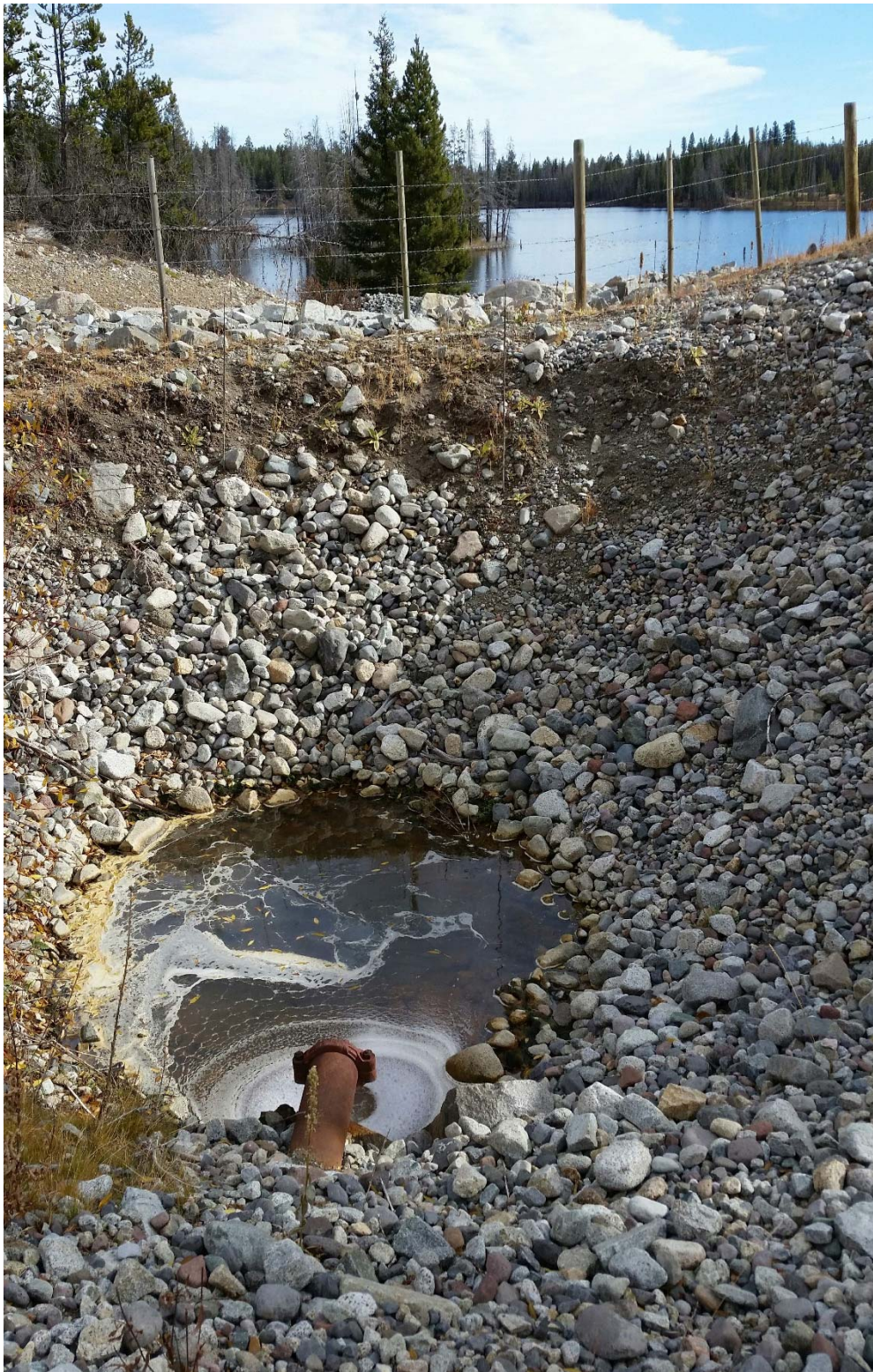
Photo II-B-11 Seepage outflow to riprap lined infiltration basin. Flow is clear and steady flowing at approximately 2 L/s (BTH-2017-13)
