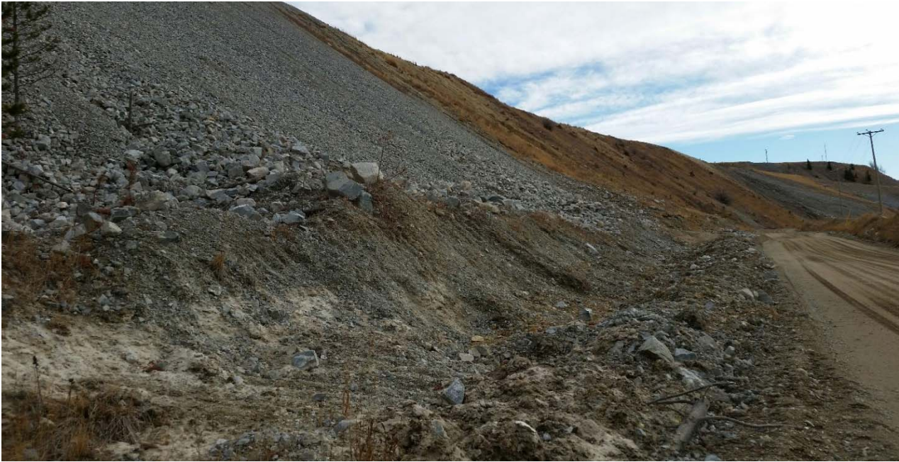
Photo II-A-4 Downstream slope of dam, historic repair of slope scar, no new signs of erosion or scouring. View towards left abutment lower down (BTH-2017-02)
