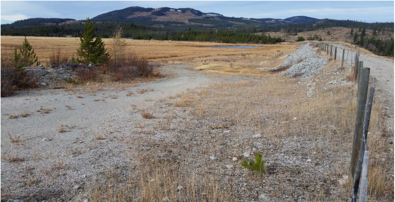
Photo II-B-2 Upstream slope of dam looking towards left abutment. The rockfill riprap on the upstream slope is intact and shows no signs of degradation or erosion (BTH-2017-07)
