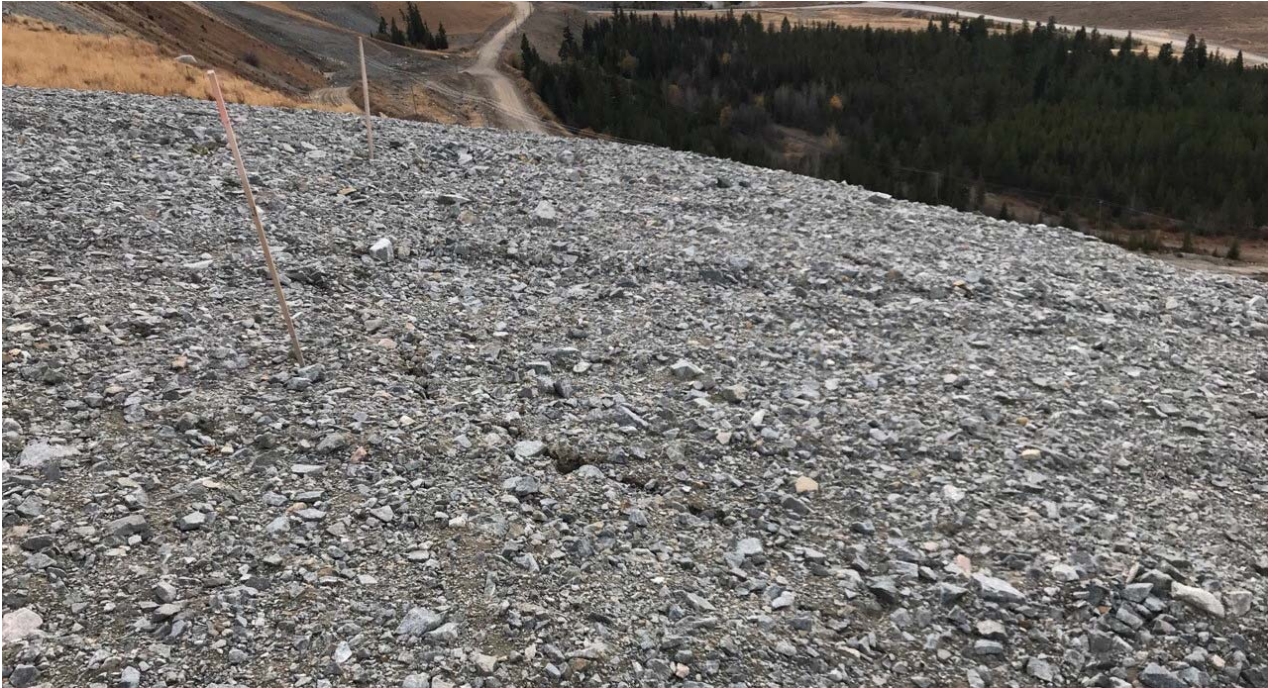
Photo II-A-2 Crack from September 2015 rockfill placement (repair of erosion gully). Area marked and monitored by THVCP, no visible change from 2016 report, crack width ~35mm (BTH-2017-03)
