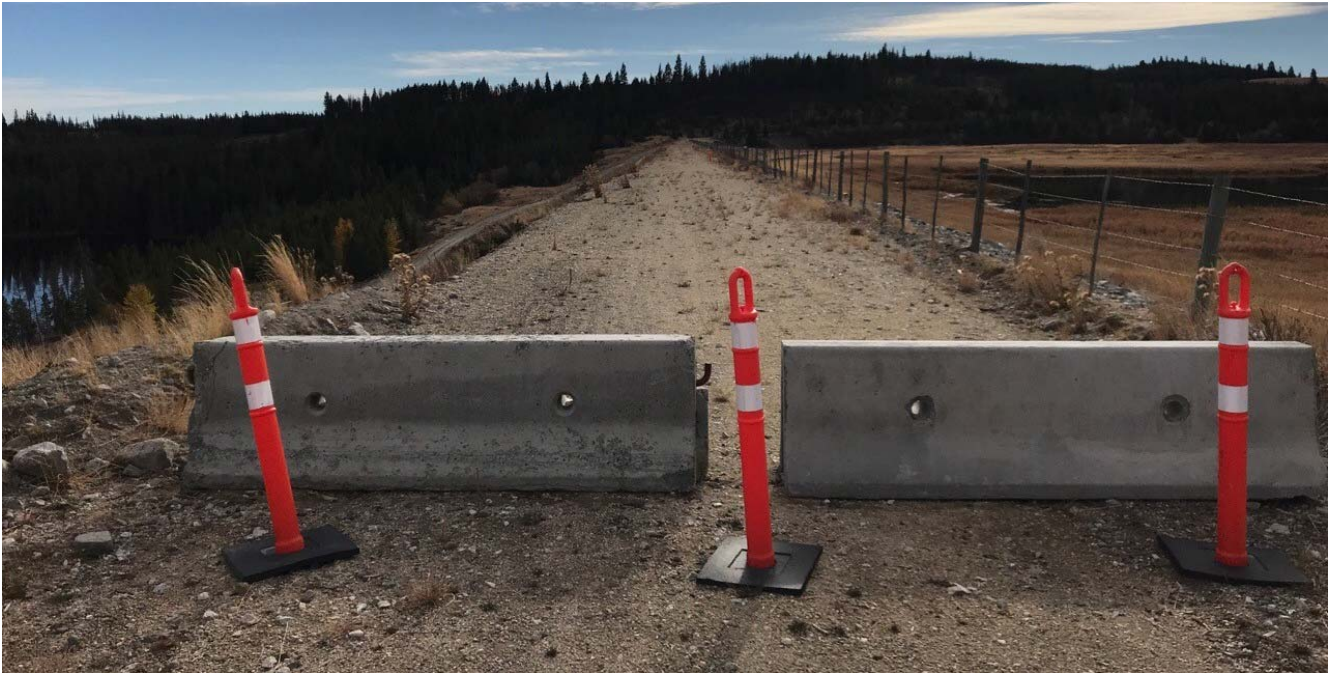
Photo II-B-18 Crest of dam view towards right abutment, vehicle access blocked off at time of inspection (BTH-2017-20)
