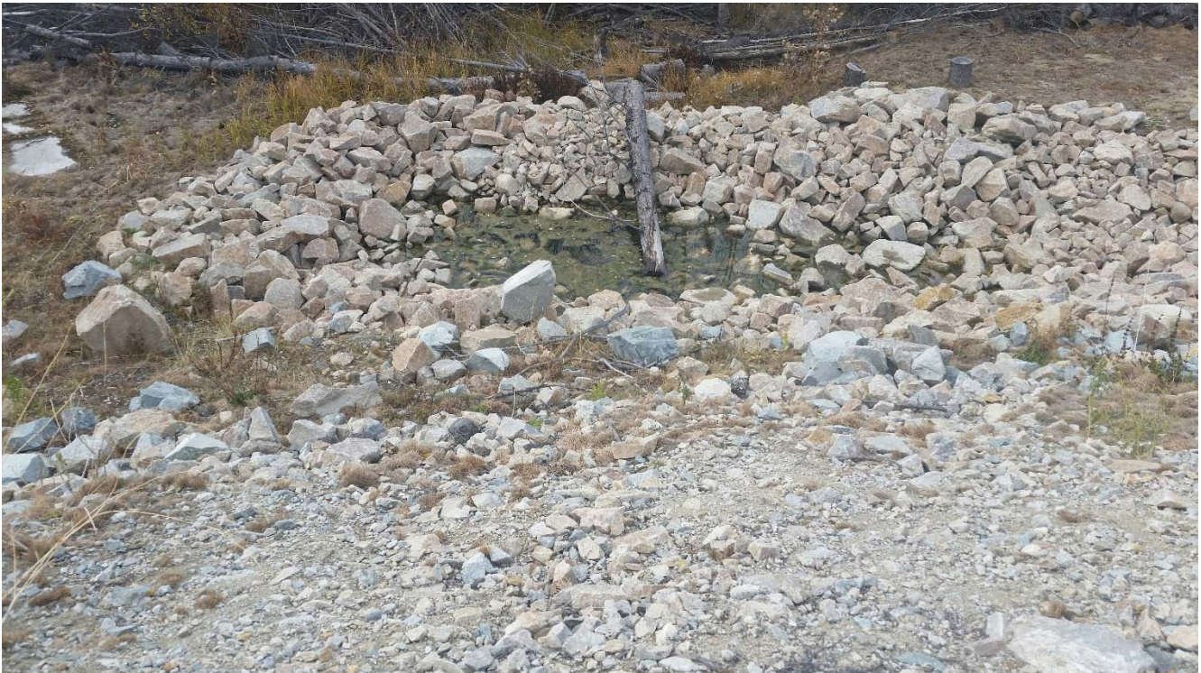
Photo II-C-9 Accumulation of water at the end of spillway riprap (BTH-2017-26)
