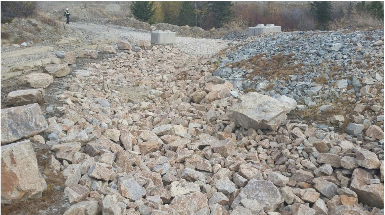
Photo II-C-7 Spillway channel in good condition, no signs of deterioration. Downstream riprap material size 50-300mm with outliers as large as 600mm (BTH-2017-25)
