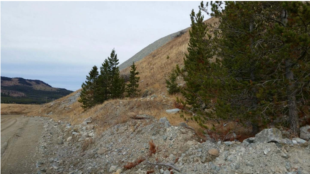
Photo II-A-5 Downstream slope of dam, historic repair of slope scar, no signs of erosion or scouring. View towards right abutment (BTH-2017-02)
