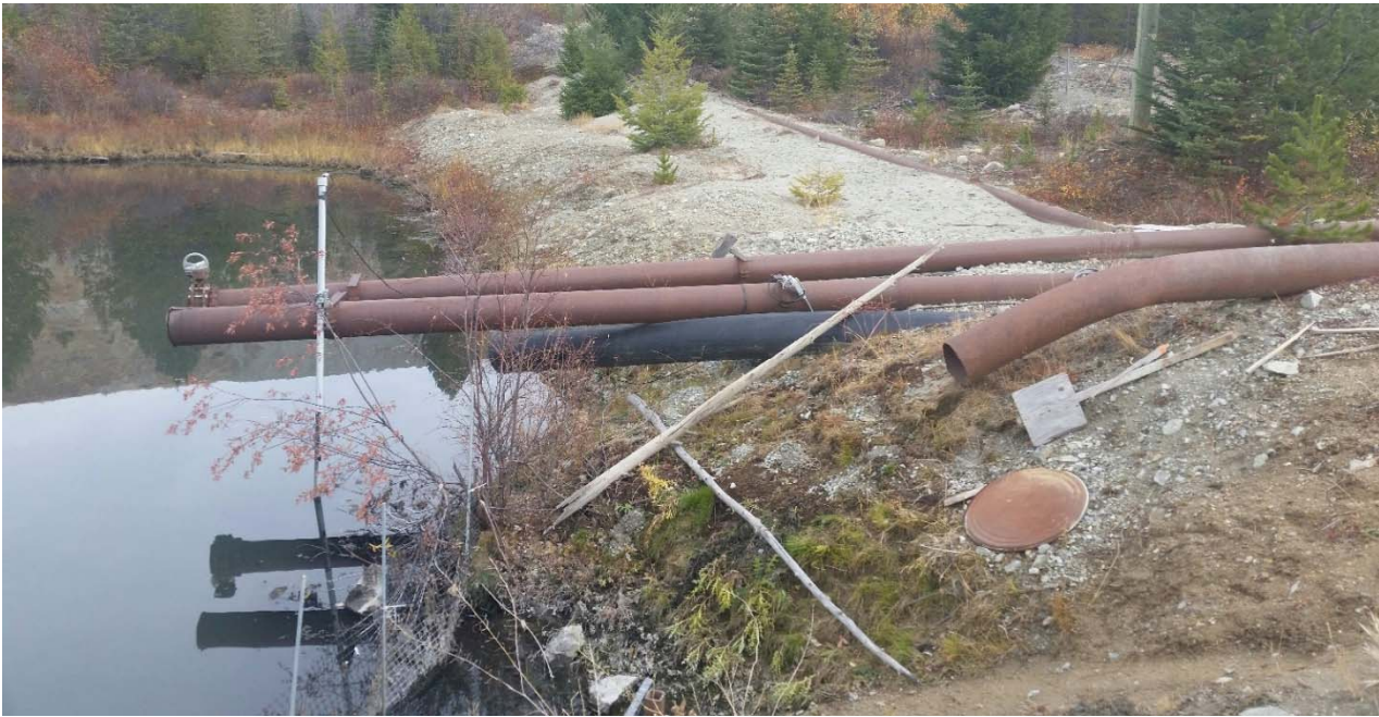
Photo II-C-2 Decommissioned outflow pipes, and surrounding debris (BTH-2017-27)
