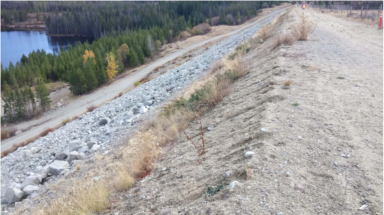
Photo II-B-20 Signs of erosion along crest and upper till section of the downstream slope of the dam (BTH-2017-21)
