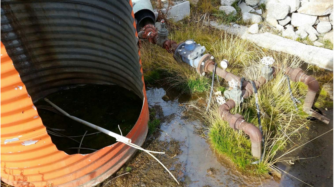
Photo II-B-10 Seepage outfall valve control at gauge-house (BTH-2017-13)
