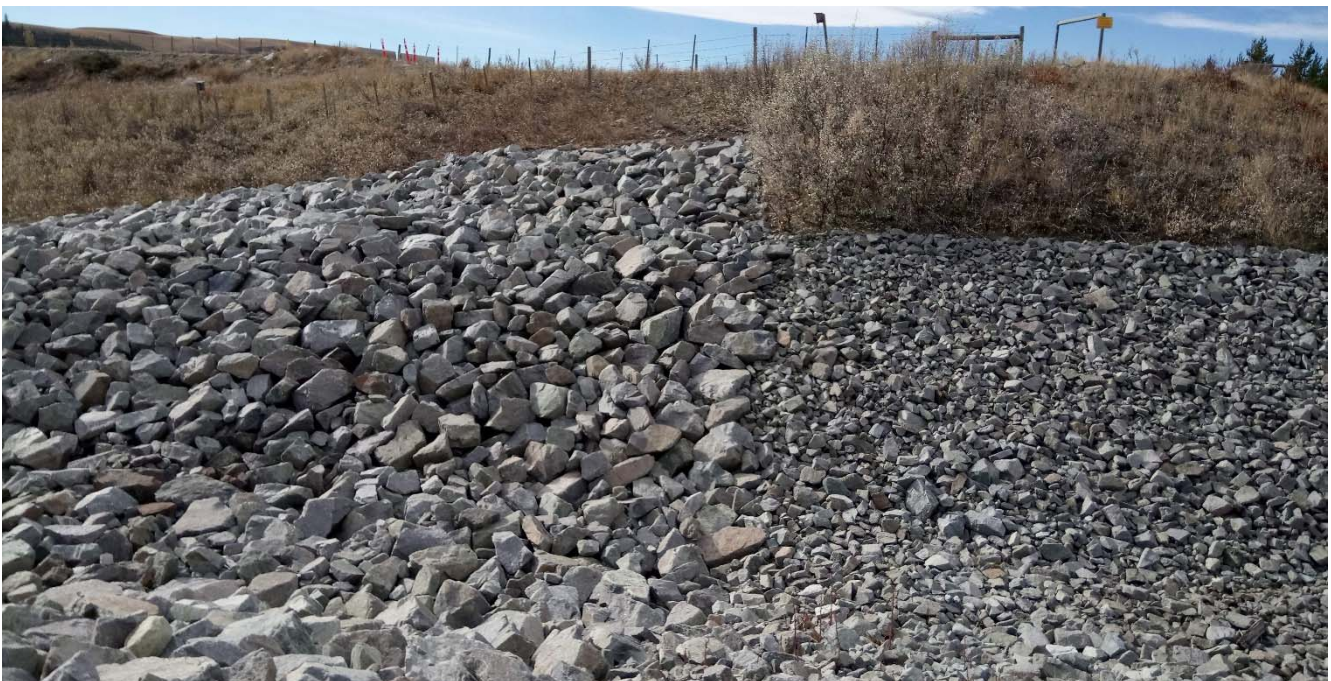
Photo II-B-15 Spillway transition from fine riprap to coarse riprap as the channel steepens, view towards dam crest. Fine riprap size approximately 50-125mm, Coarse riprap approximately 150-300mm (BTH-2017-17)
