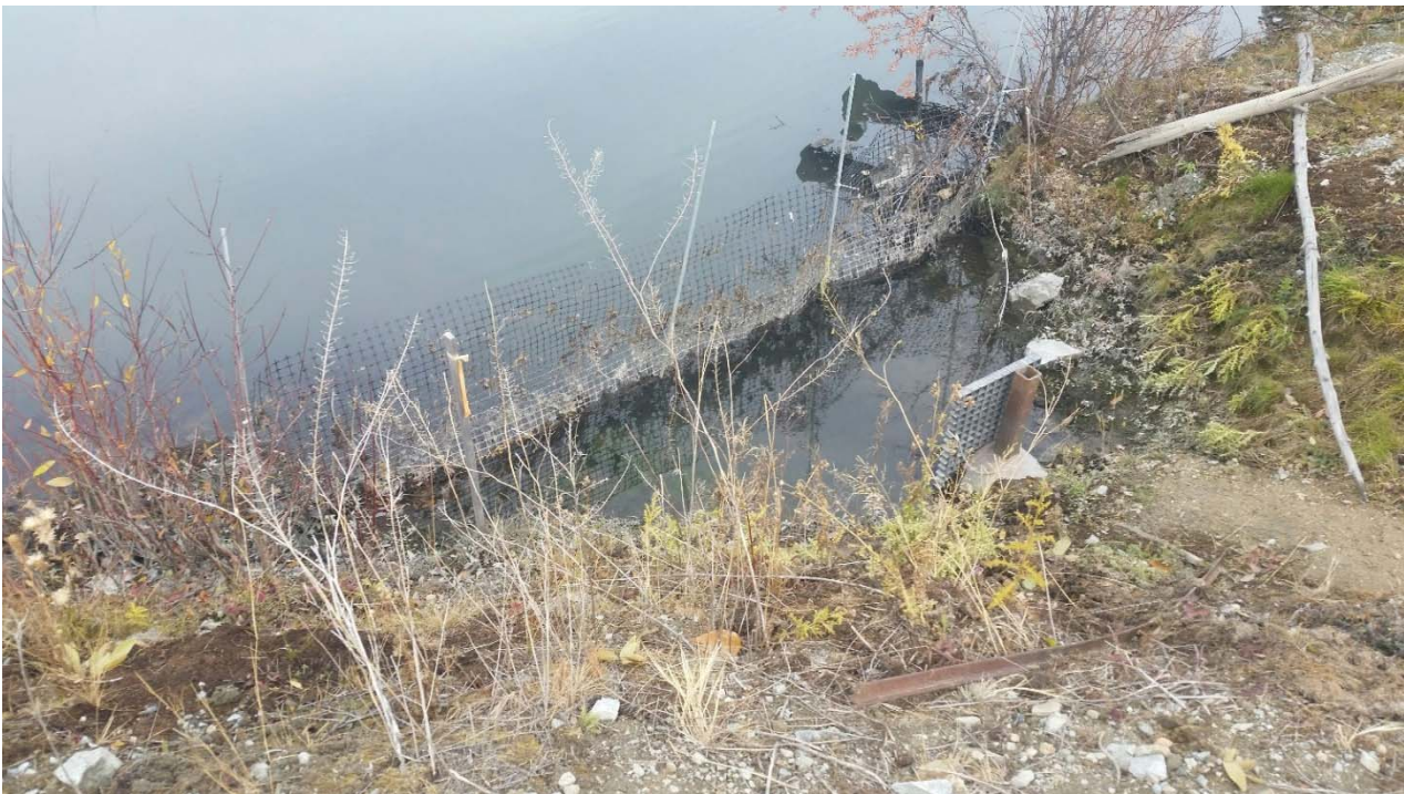
Photo II-C-3 Outlet intake with clear trash rack and debris fence with minor obstructions (BTH-2017-27)
