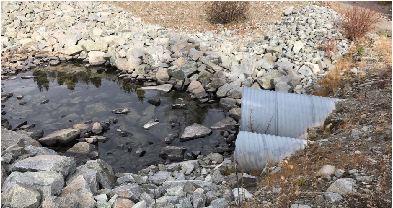
Photo II-B-17 Water accumulation on upstream side of spillway culverts, no flow observed at time of inspection. Both culverts clean, and free of obstructions (BTH-2017-19)
