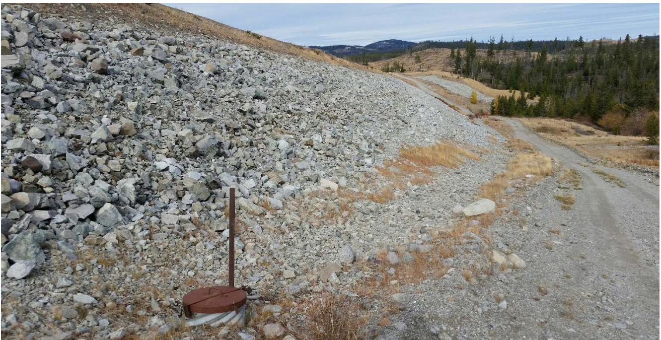
Photo II-B-3 Downstream slope of dam including toe drain near right abutment, no signs of erosion or scouring in outer rock layer (BTH-2017-08)
