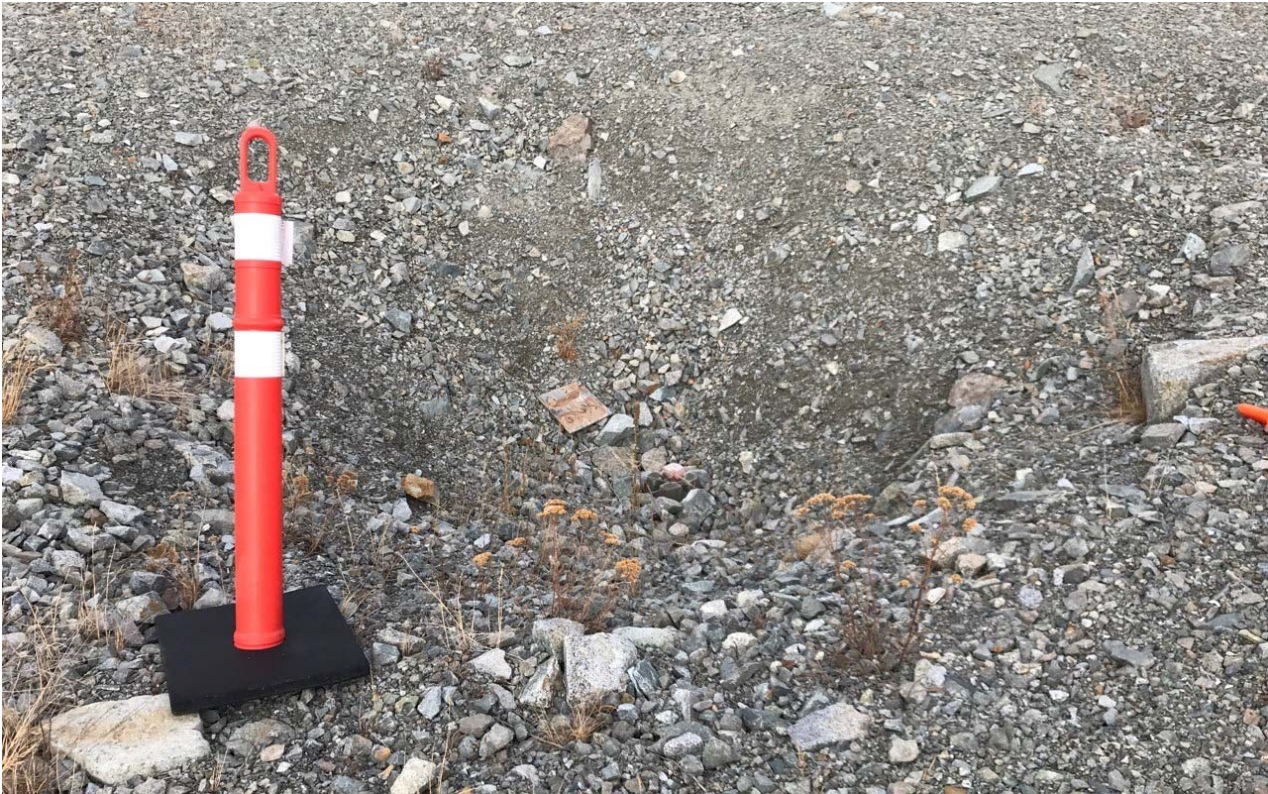
Photo II-A-8 Sinkhole on tailings beach, no additional cracks or depressions since 2016 inspection (BTH-2017-04)
