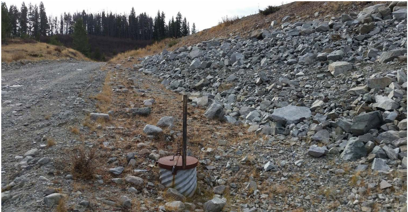
Photo II-B-4 Downstream slope of dam including toe drain near right abutment, view towards right abutment (BTH-2017-08)
