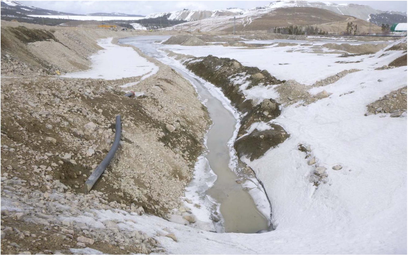
Photo II-15 Inflow pipes at southwest corner of pond. No flow from pipes. Photo taken looking northeast (SDP-2017-11)
