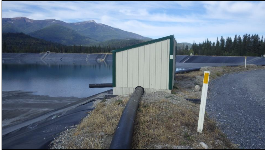
PHOTO 22 – Typical spigot location discharge point (with hut).
