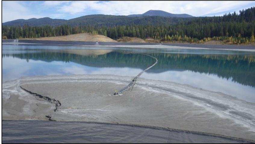
PHOTO 16 – W2 floating pipe discharge location.
