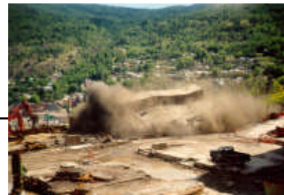
The Dressing Plant, part of Trail's lead production circuit in the days prior to KIVCET, was demolished in July 1999.
