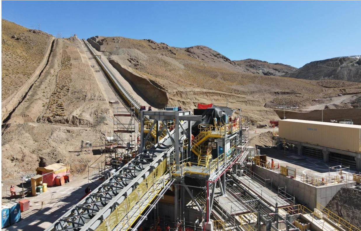
QB2 Crushing and Conveying
