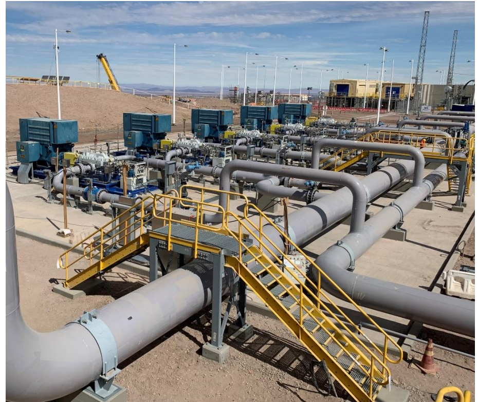
Water supply pump station 3, July 2022
