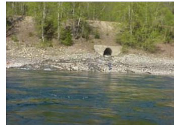
Sullivan Creek showing effect of road and culvert on habitat
